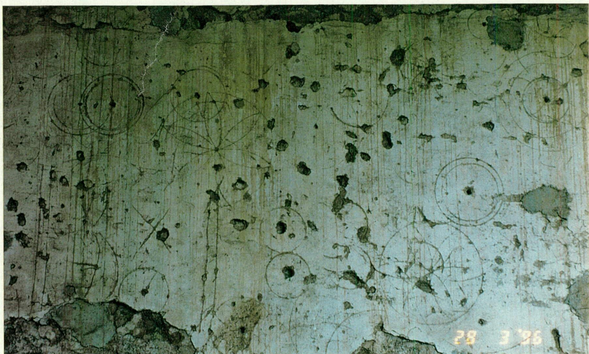
Plate 12 The stub of the original southwest end wall shows on the southeast side.
