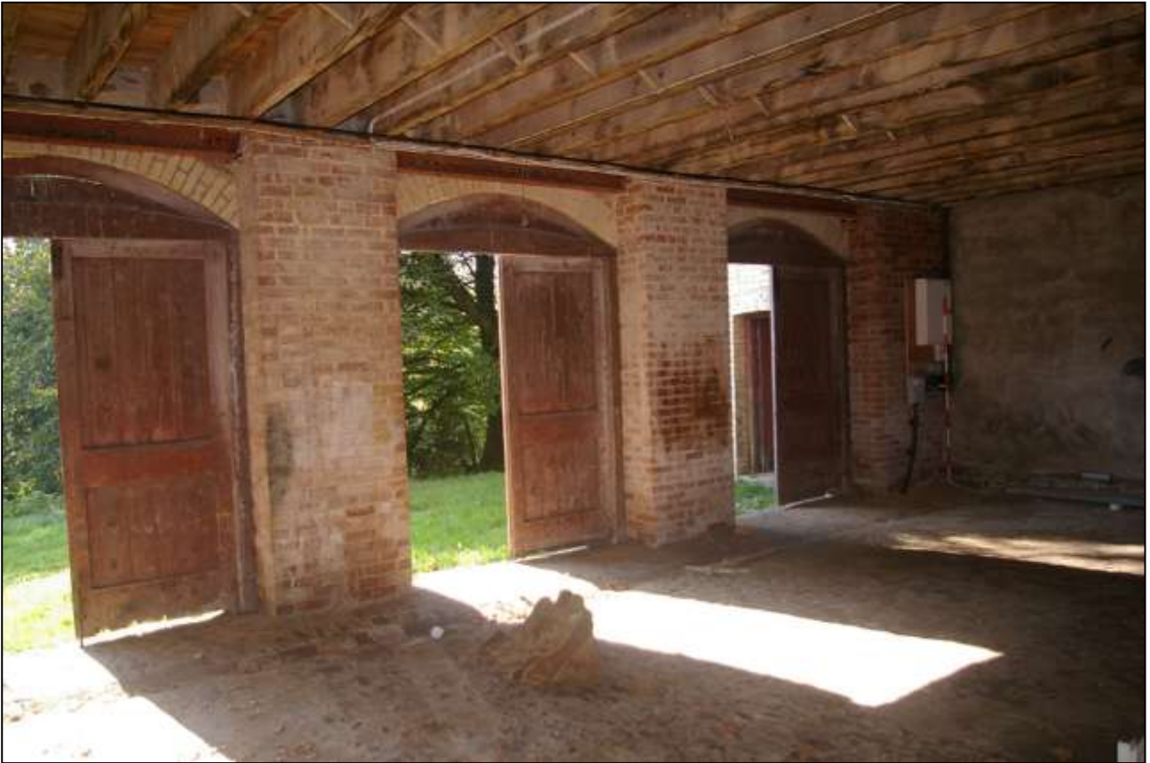
45. THE SOUTH WALL OF THE CARRIAGE HOUSE WITH THE THREE MATCHED DOORS; FROM THE NORTH-EAST.
