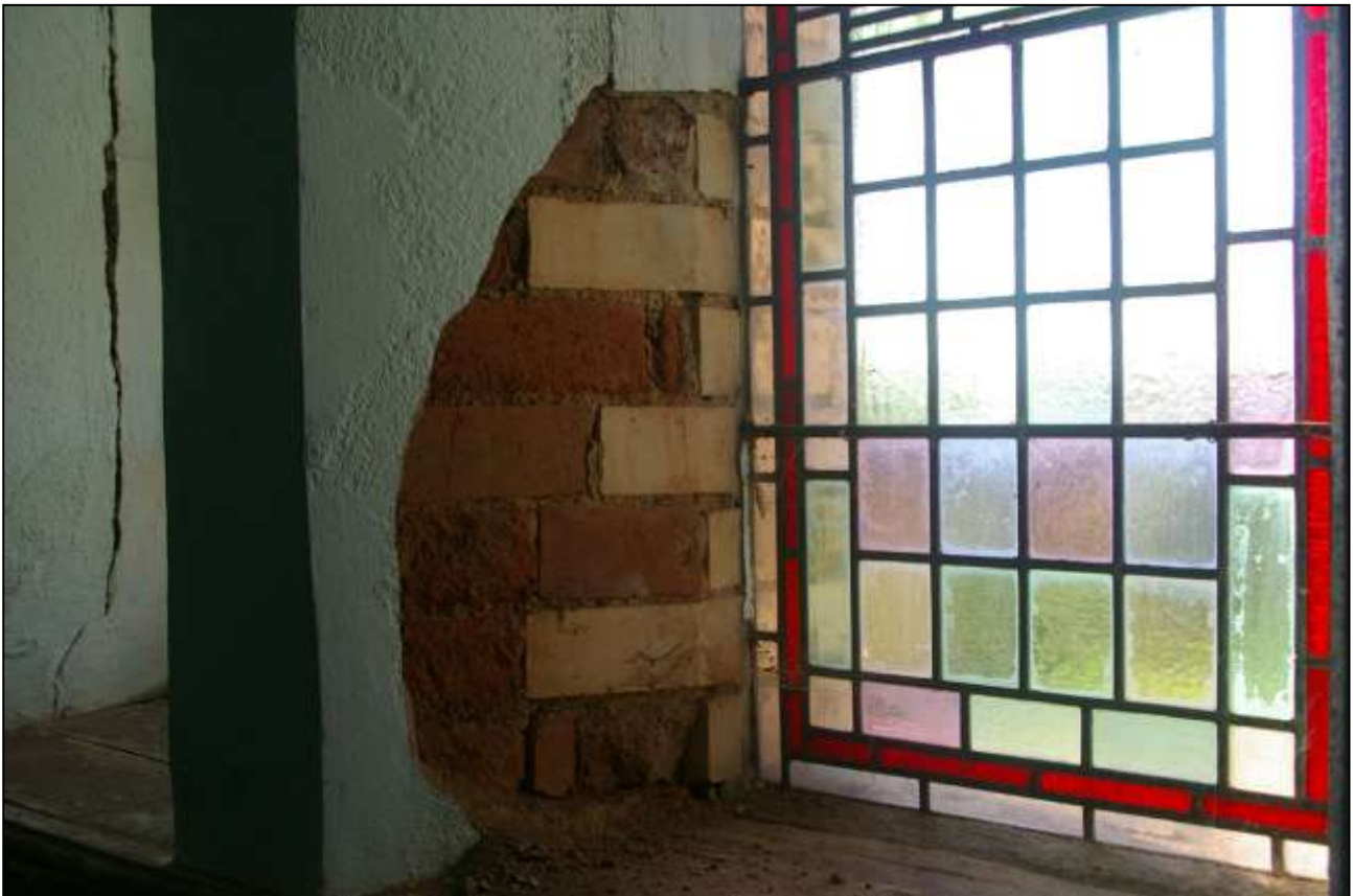
111. DETAIL OF REMOVED PLASTER AT WEST WINDOW, W18; SHOWING EXTERNAL CREAM CERAMIC BRICK, INTERNAL RED ENGINEERING BRICK; FROM THE EAST-NORTH-EAST.
