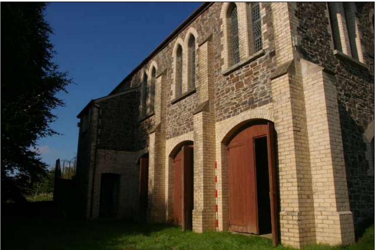
22. THE SOUTH ELEVATION OF THE CROSSWING, SHOWING SUBTLE DIFFERENCES IN BUILD, SUCH AS BRICK BUTTRESSES AND LOWER GROUND FLOOR; FROM THE SOUTH-EAST.
