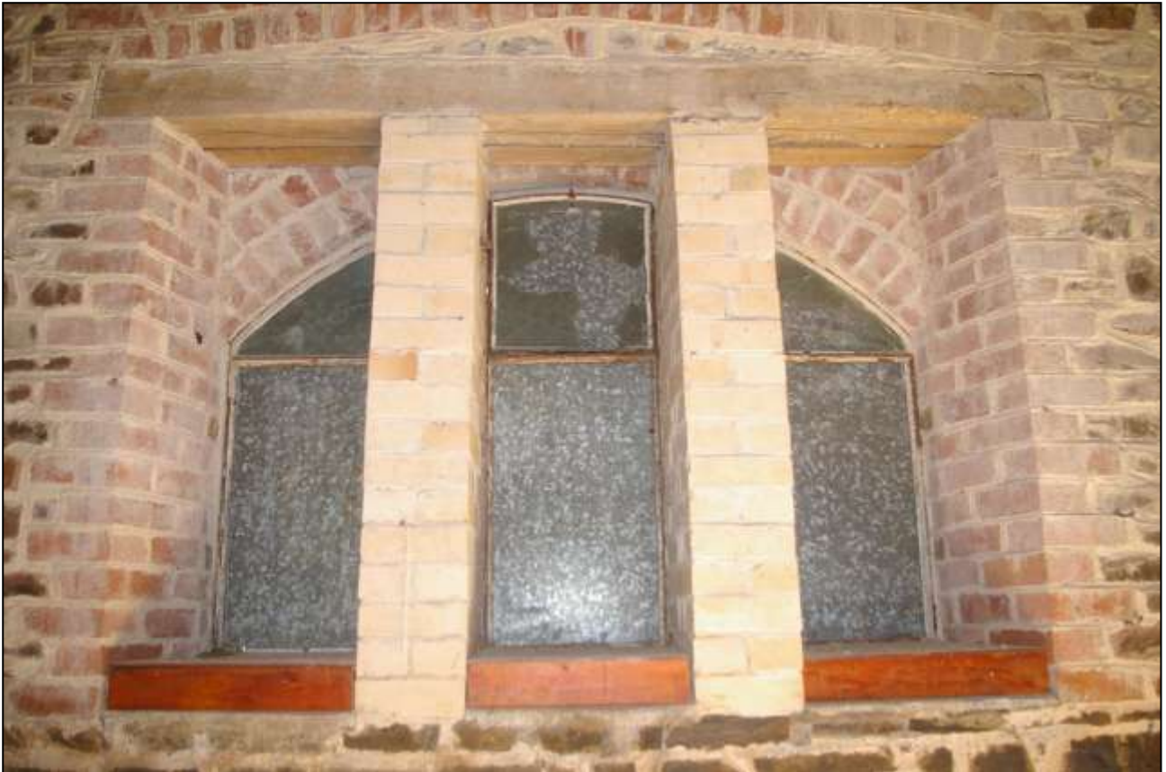
52. THE EAST TRIPARTITE WINDOW WHICH LIGHTS THE CARRIAGE HOUSE; FROM THE WEST.
