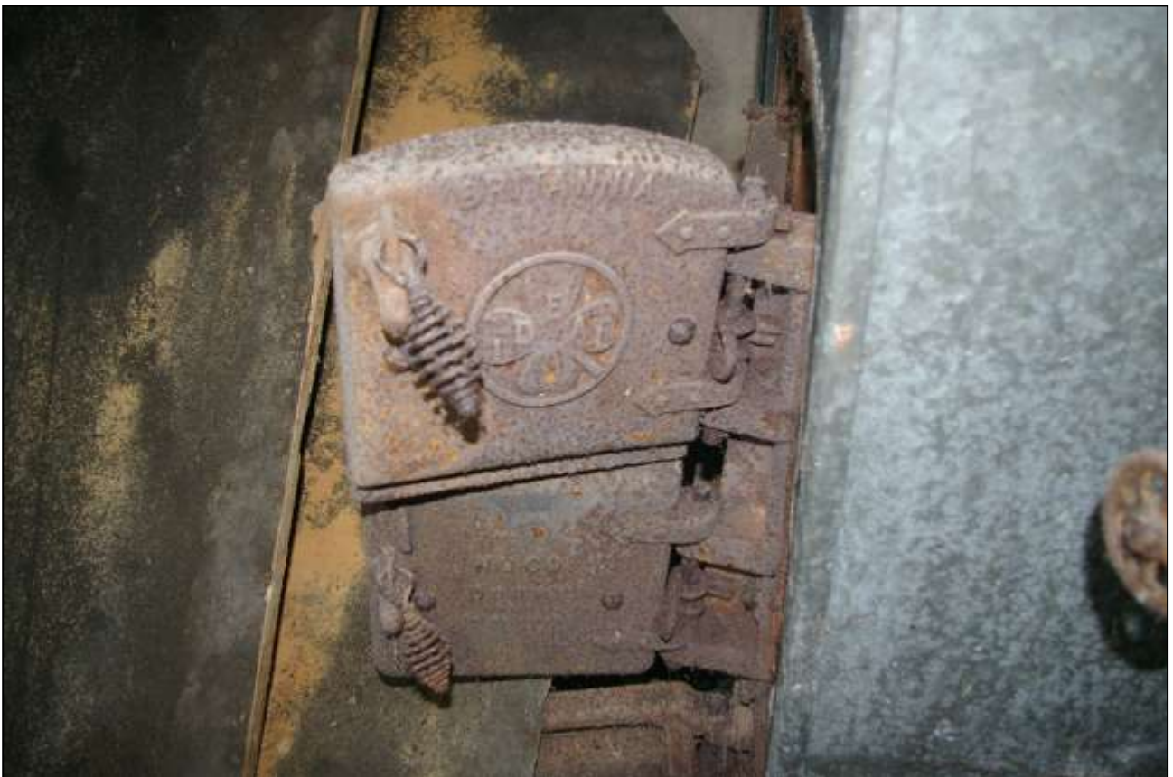
33. THE MAKE AND MODEL OF THE BOILER; FROM THE WEST.
