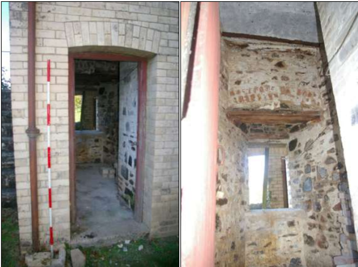
40. LEFT: D15, LOOKING INTO THE BASEMENT FLOOR OF THE SERVICES BLOCK, WITH 2M SCALE; FROM THE EAST, SOUTH-EAST.
