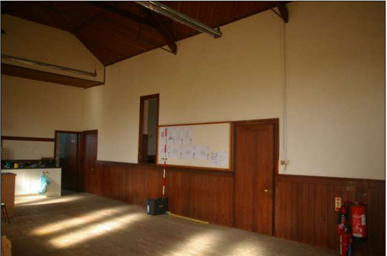
97. THE PARTY WALL BETWEEN COMMUNITY HALL AND CHAPEL, WITH 2M SCALE; FROM THE SOUTH-EAST.
