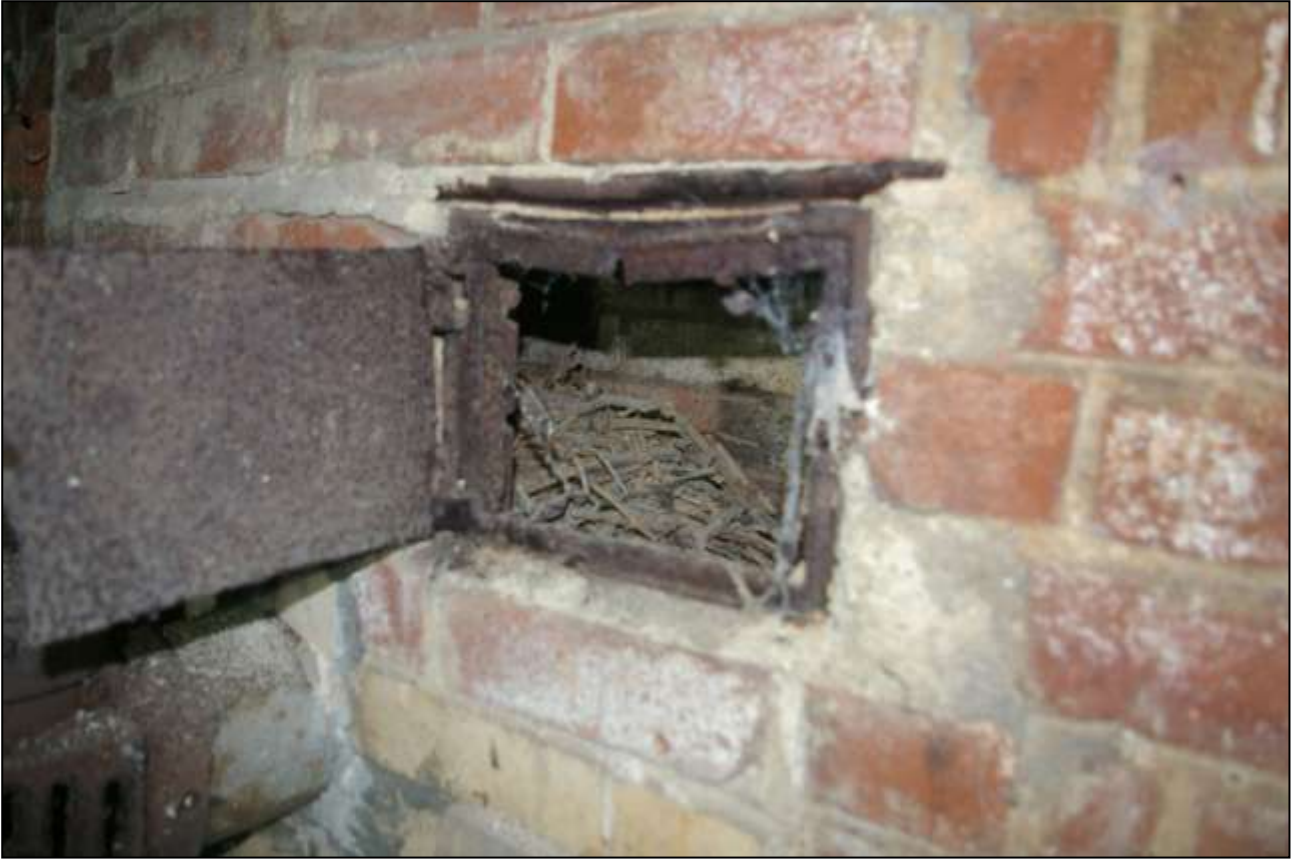
32. VIEW THROUGH THE HATCH SHOWING THE FLUE BLOCKED WITH JACKDAW NESTS; FROM THE NORTH-WEST.
