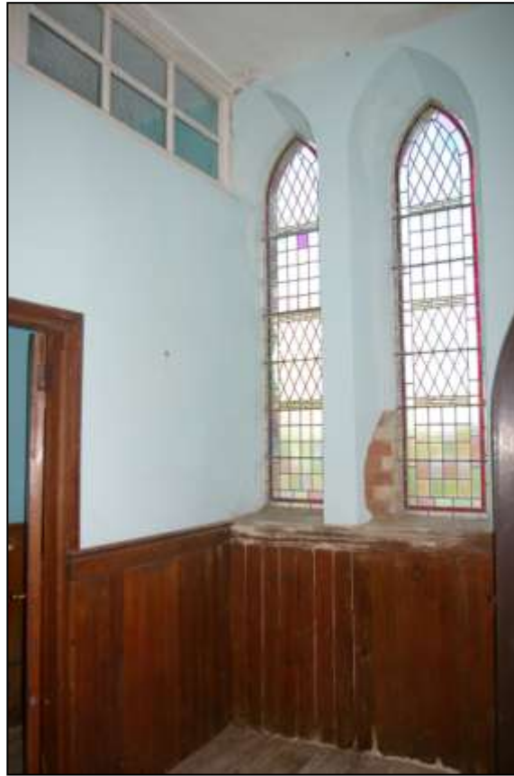
110. THE CURRENT WEST CLOAKROOM AND GENTS TOILETS, WITH INSERTED PARTITION; FROM THE EAST-NORTH-EAST.
