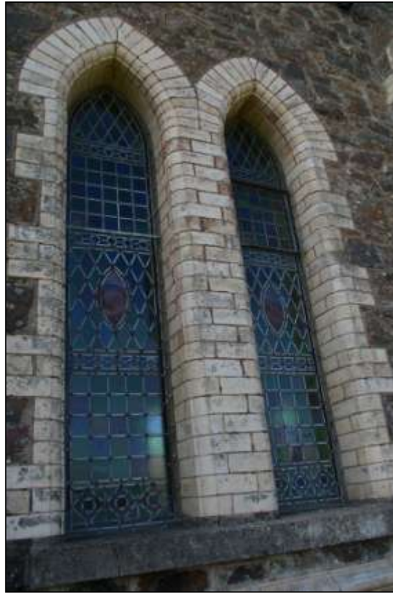
17. WINDOW 6 ON THE EAST WALL, AN EXAMPLE OF THE SIDE ELEVATION WINDOW DESIGN; FROM THE EAST.
