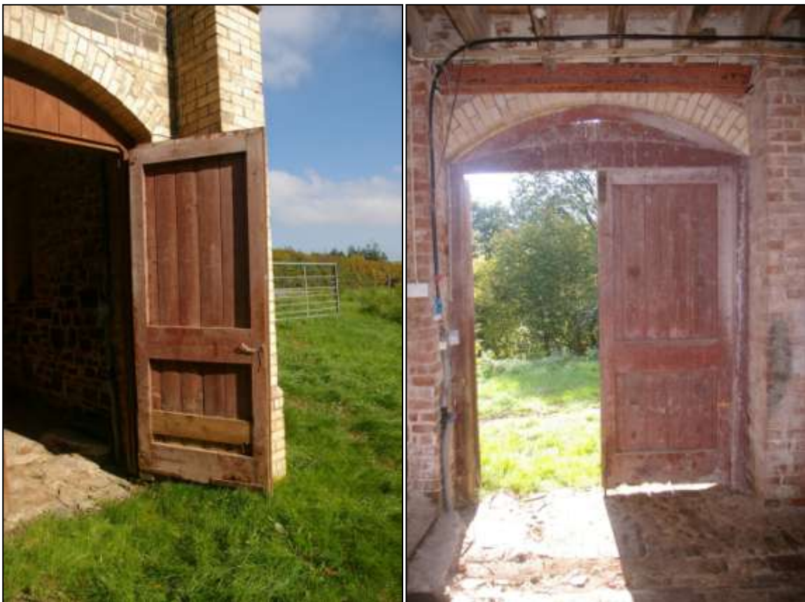
43. LEFT: D12, AN EXAMPLE OF ONE OF THE BOARDED AND FRAMED DOORS; FROM THE SOUTH, SOUTH-WEST.
