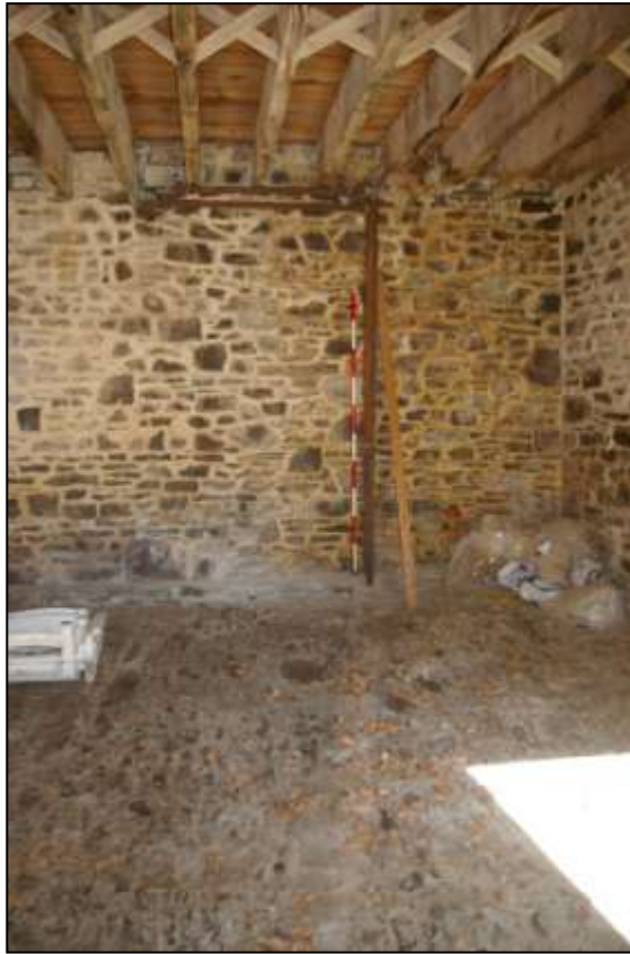
50. THE BOILER PIPES, WHERE THEY BREACH THE WALL OF THE CARRIAGE HOUSE, WITH 2M SCALE; FROM THE SOUTH.
