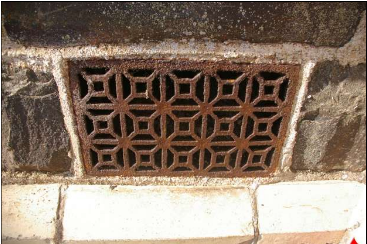
11. THE IRONWORK GRILLS TO THE AIR VENTS ON THE EAST WALL OF THE CHAPEL; FROM THE NORTH-EAST.
