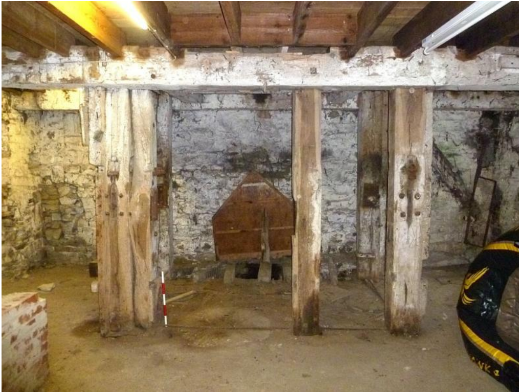
Ground floor. Bridge posts and hurst from the west (half metre scale)
