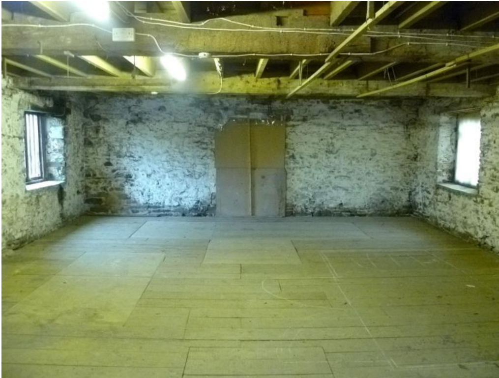
First floor, looking east. Plywood panels indicate former millstone positions, a former opening over the brick plinth (left) and the sack traps (centre foreground)
