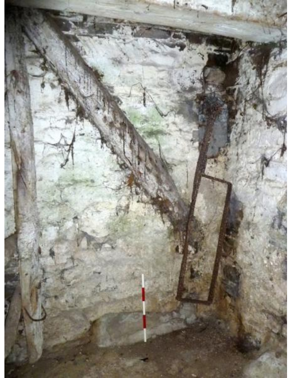
Penstock control lever in south-east corner
