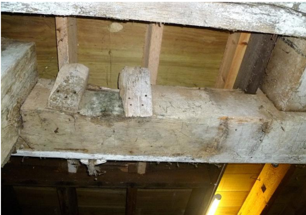
Rear of front hurst beam, with cleats marking former millstone spindle position
