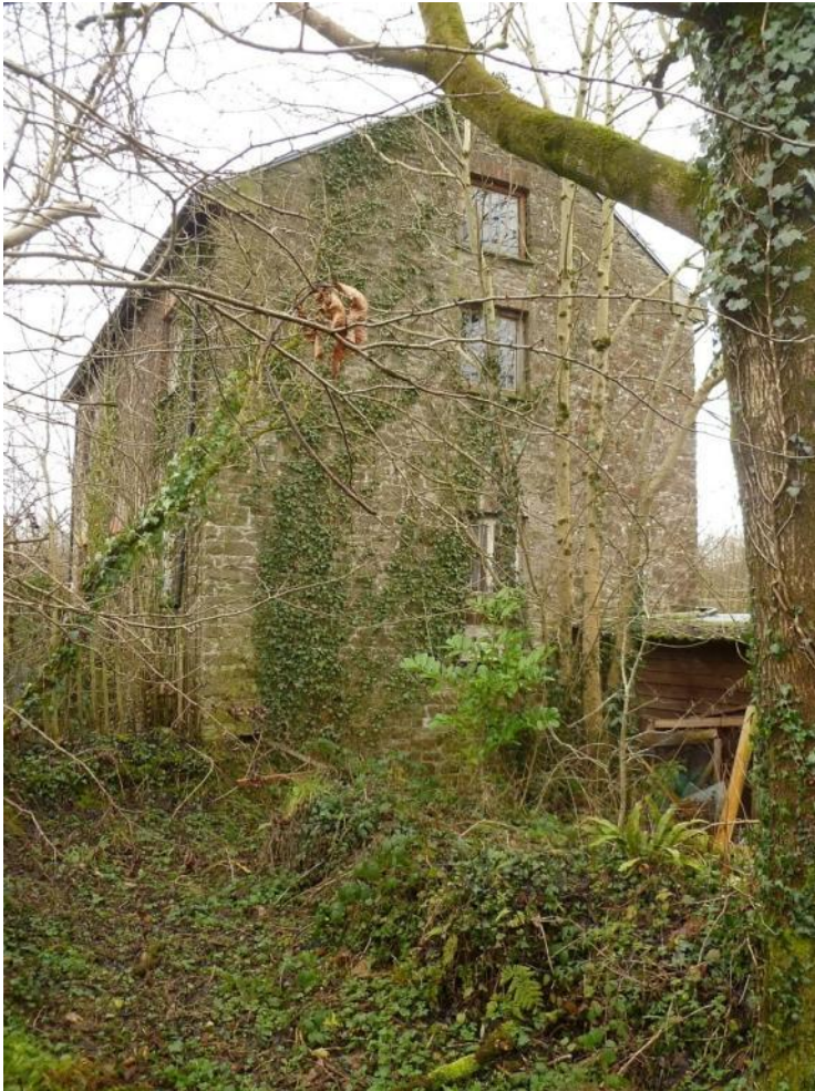
East gable end with silted leat to left foreground
