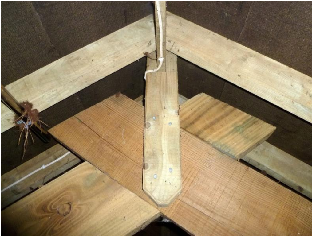
Detail at apex of roof truss, with timber nailed onto principal to carry ridge board
