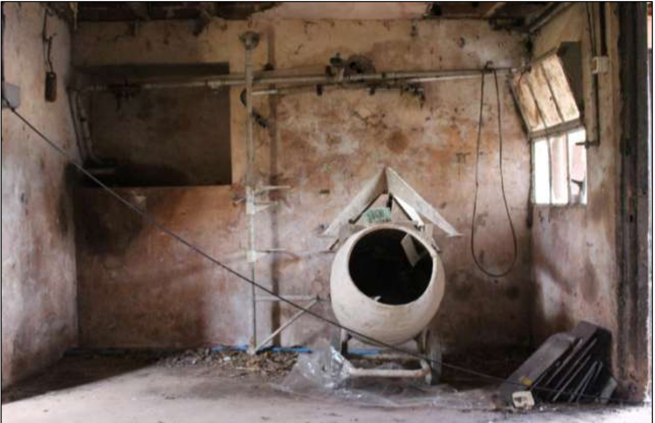
B5 GF INTERIOR, THE DAIRY, SHOWING THE BLOCKED DOORWAY TO B4A; VIEWED FROM THE SOUTH-WEST.
