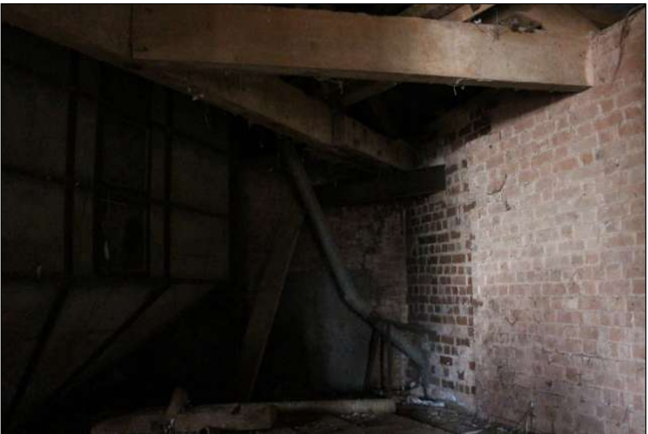
B5 FF INTERIOR, THE NORTH-WEST CORNER SHOWING THE BLOCKED LOADING DOOR; VIEWED FROM THE ENE.
