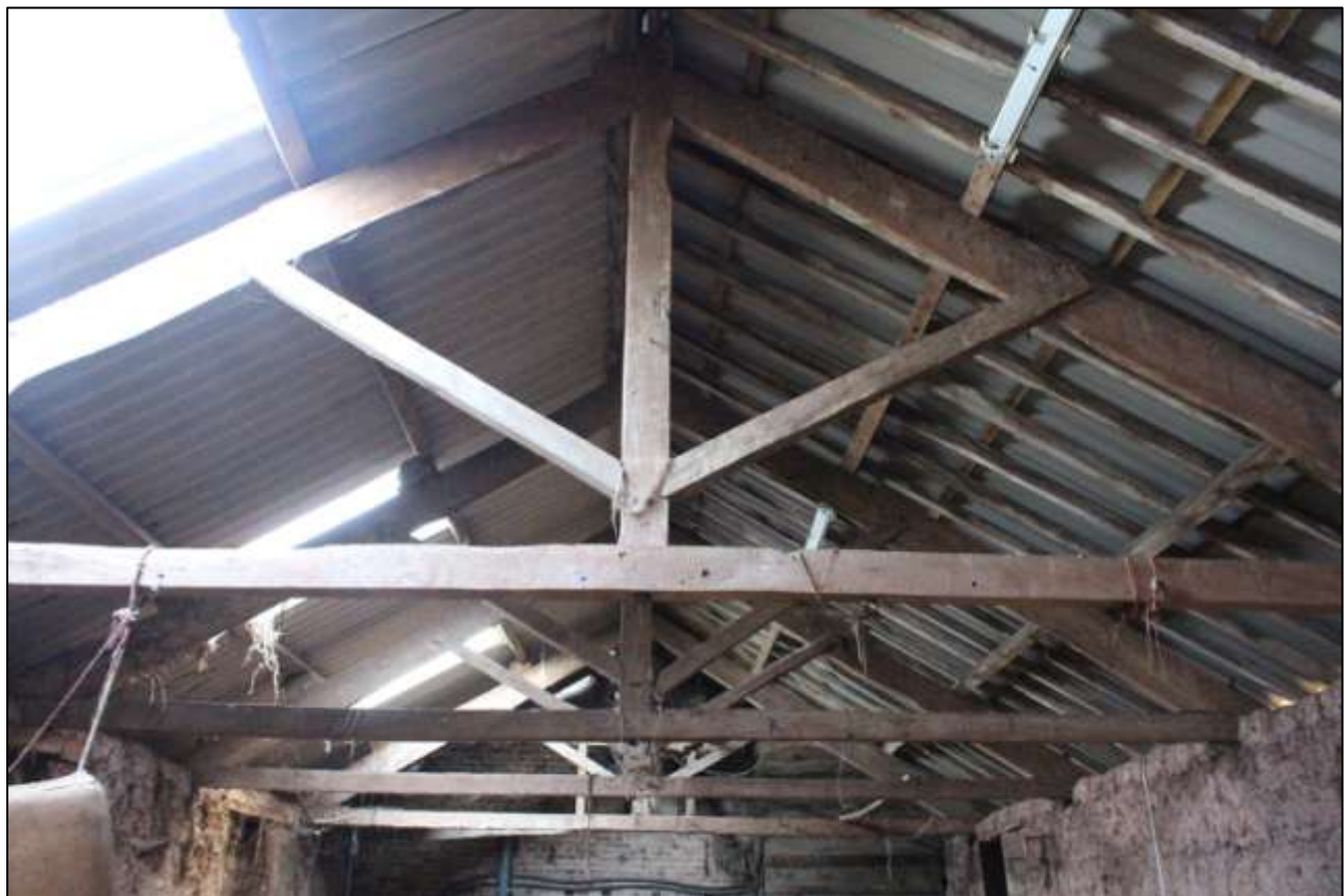
B2 FF INTERIOR, SHOWING THE KINGPOST ROOF TRUSSES; VIEWED FROM THE SOUTH.
