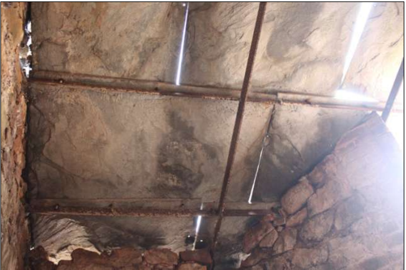
B3 INTERIOR, THE ROOF OF SLABS ON IRON BEAMS; VIEWED FROM THE SOUTH-WEST AND BENEATH.
