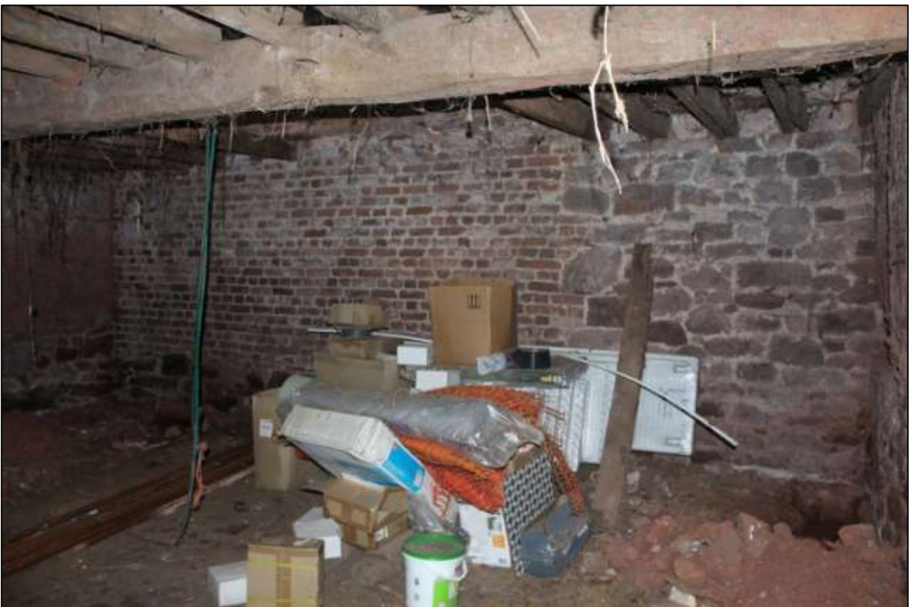
B2 GF INTERIOR; THE WALL OF THE FARMHOUSE AT THE SOUTH END OF THE BUILDING; VIEWED FROM THE NNW.
