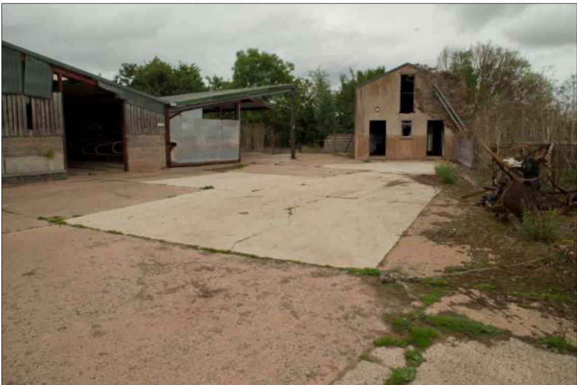
FIGURE 27: B11 THE MODERN COW CUBICLES (LEFT) AND B12 MILKING PARLOUR (RIGHT); VIEWED FROM THE SOUTH-WEST.
