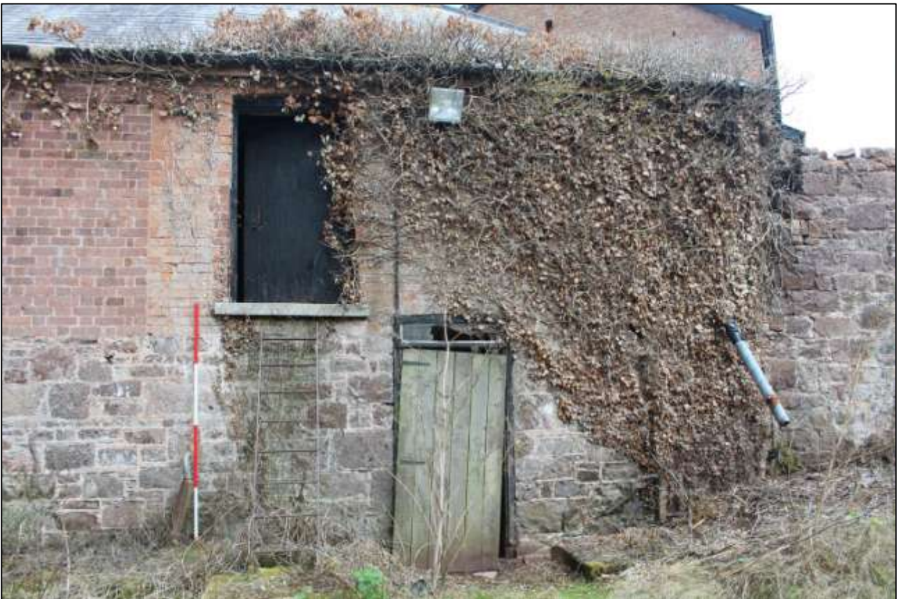
B5 EXTERIOR, NORTH-WEST WALL SHOWING GF DOOR AND FF FORCED LOADING DOOR; VIEWED FROM THE NORTH-WEST (SCALE 2M).
