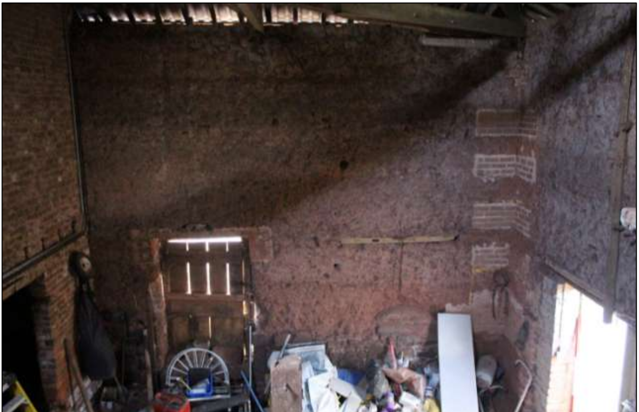
B1 INTERIOR, WEST WALL WITH D2 AND BO1; VIEWED FROM THE EAST.
