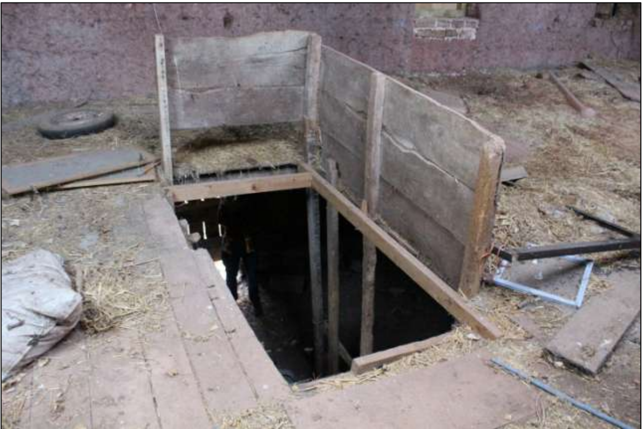
B2 FF INTERIOR, DETAIL OF THE RAIL AROUND THE STAIRWELL; VIEWED FROM THE EAST.
