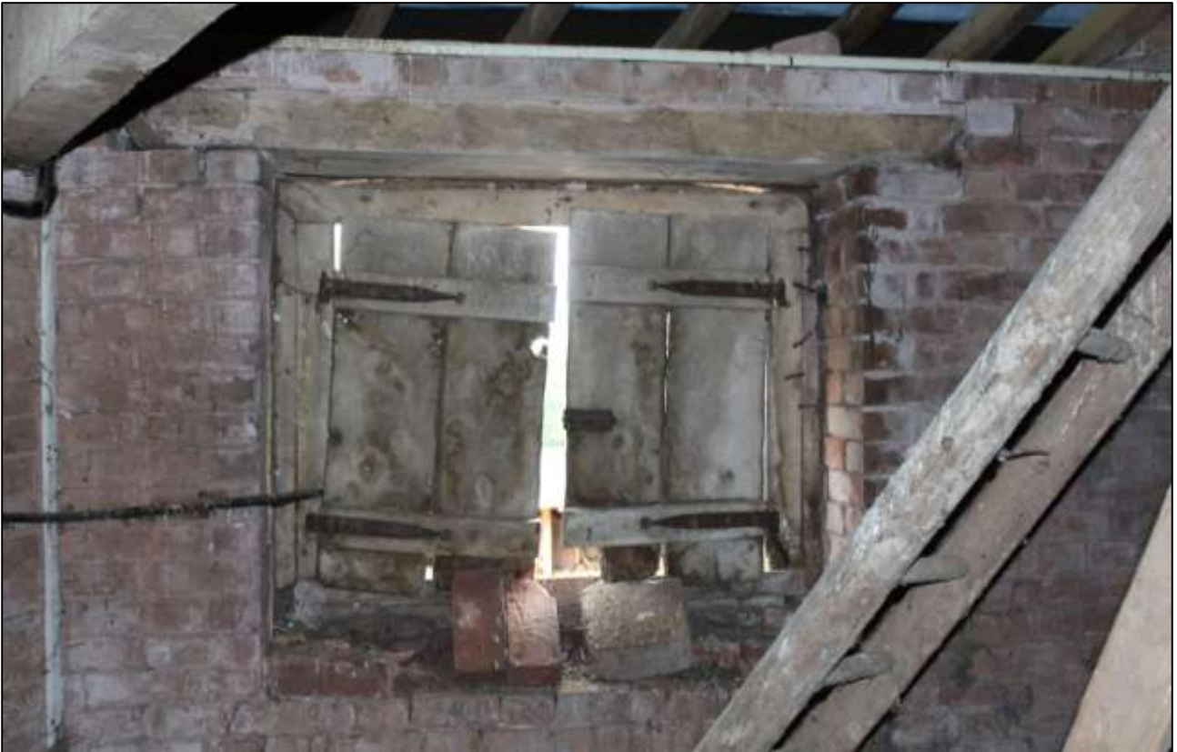
B5 FF INTERIOR, DETAIL OF THE SHUTTERED WINDOW IN THE SOUTH-EAST WALL; VIEWED FROM THE NORTH-WEST.
