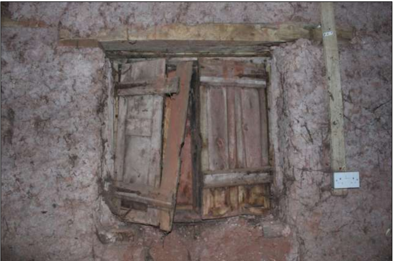
B2 GF INTERIOR, WEST WALL, DETAIL OF W2; VIEWED FROM THE EAST.
