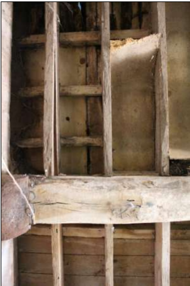
B6 GF INTERIOR, DETAIL OF THE REINFORCED FLOORS BENEATH THE THRESHING FLOORS BETWEEN THE WINNOWING DOORS, NORTH DOOR ON THE WEST SIDE; VIEWED FROM BELOW.
