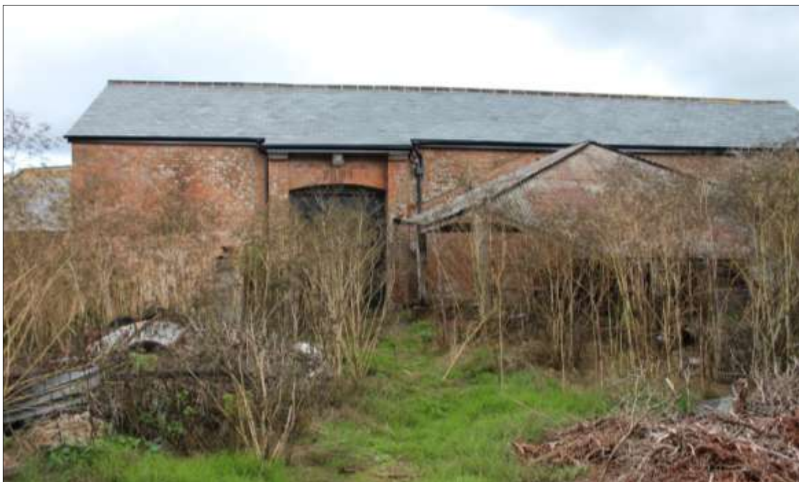
FIGURE 22: THE WEST ELEVATION OF B6 THE THRESHING BARN; VIEWED FROM THE WEST.
