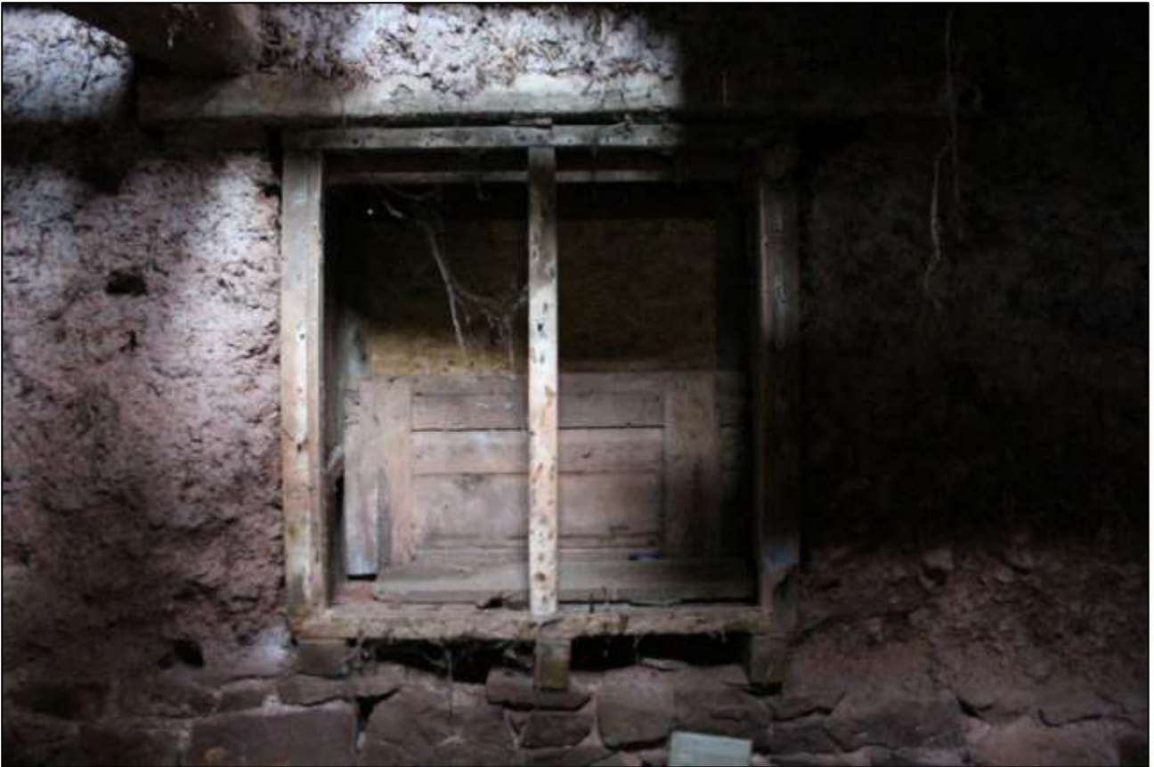
B2 GF INTERIOR, WEST WALL, DETAIL OF W1; VIEWED FROM THE EAST.
