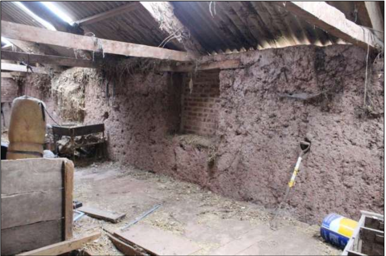
B2 FF INTERIOR, DETAIL OF THE EAST WALL AND W18; VIEWED FROM THE SOUTH-WEST.
