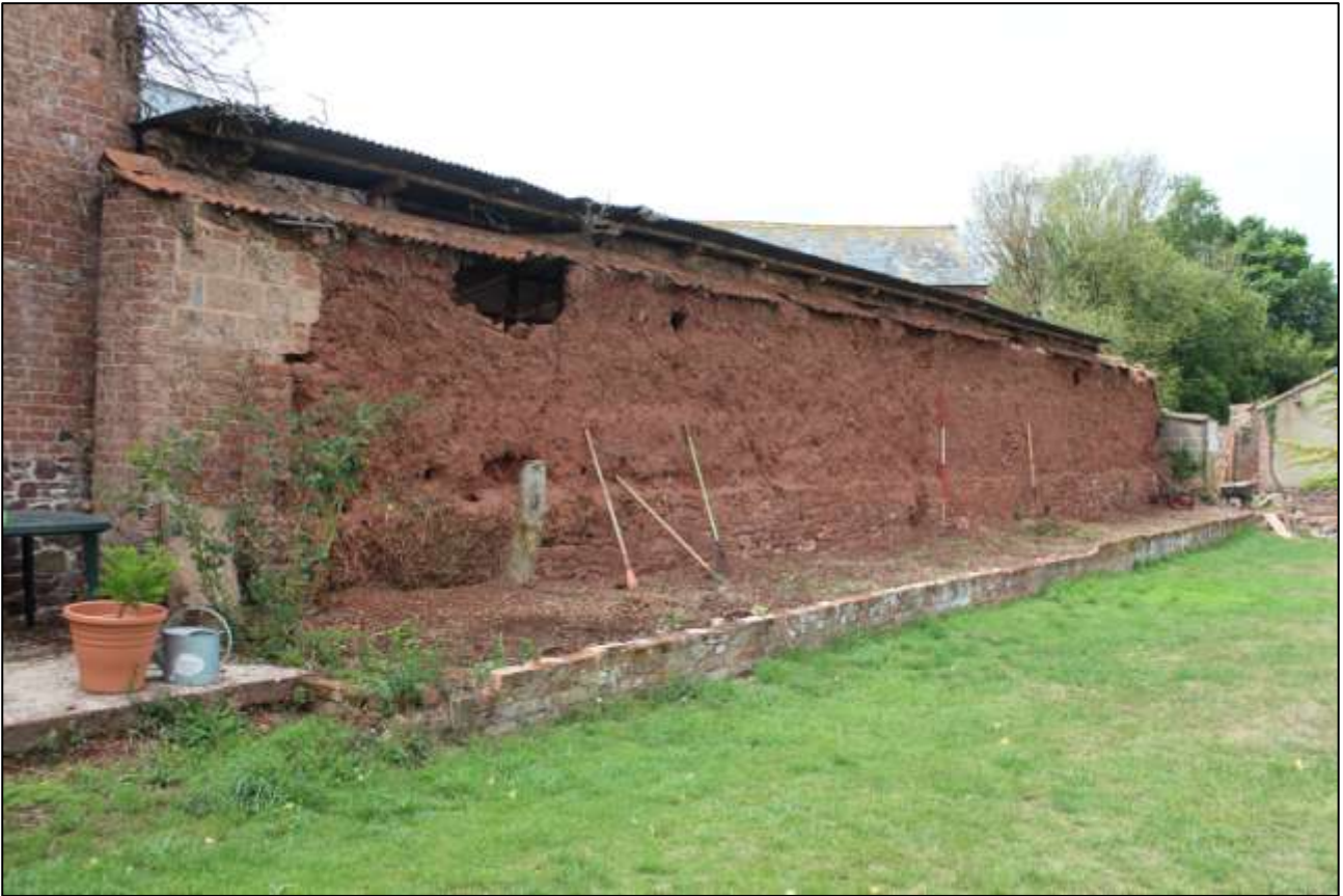
DETAIL OF THE COB GARDEN WALL; VIEWED FROM THE SOUTH-EAST (SCALE 2M).
