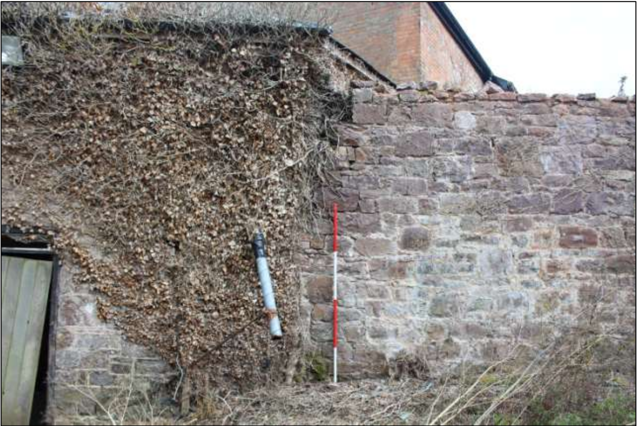
B5 EXTERIOR, NORTH-WEST WALL, SHOWING THE JOIN WITH THE STONE YARD WALL TO THE WEST; VIEWED FROM THE NORTH-WEST (SCALE 2M).
