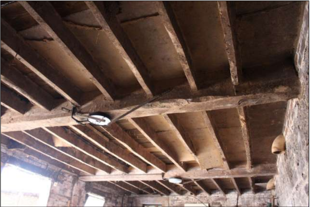
B4A INTERIOR, DETAIL OF THE CEILING; VIEWED FROM THE NORTH-EAST AND BENEATH.
