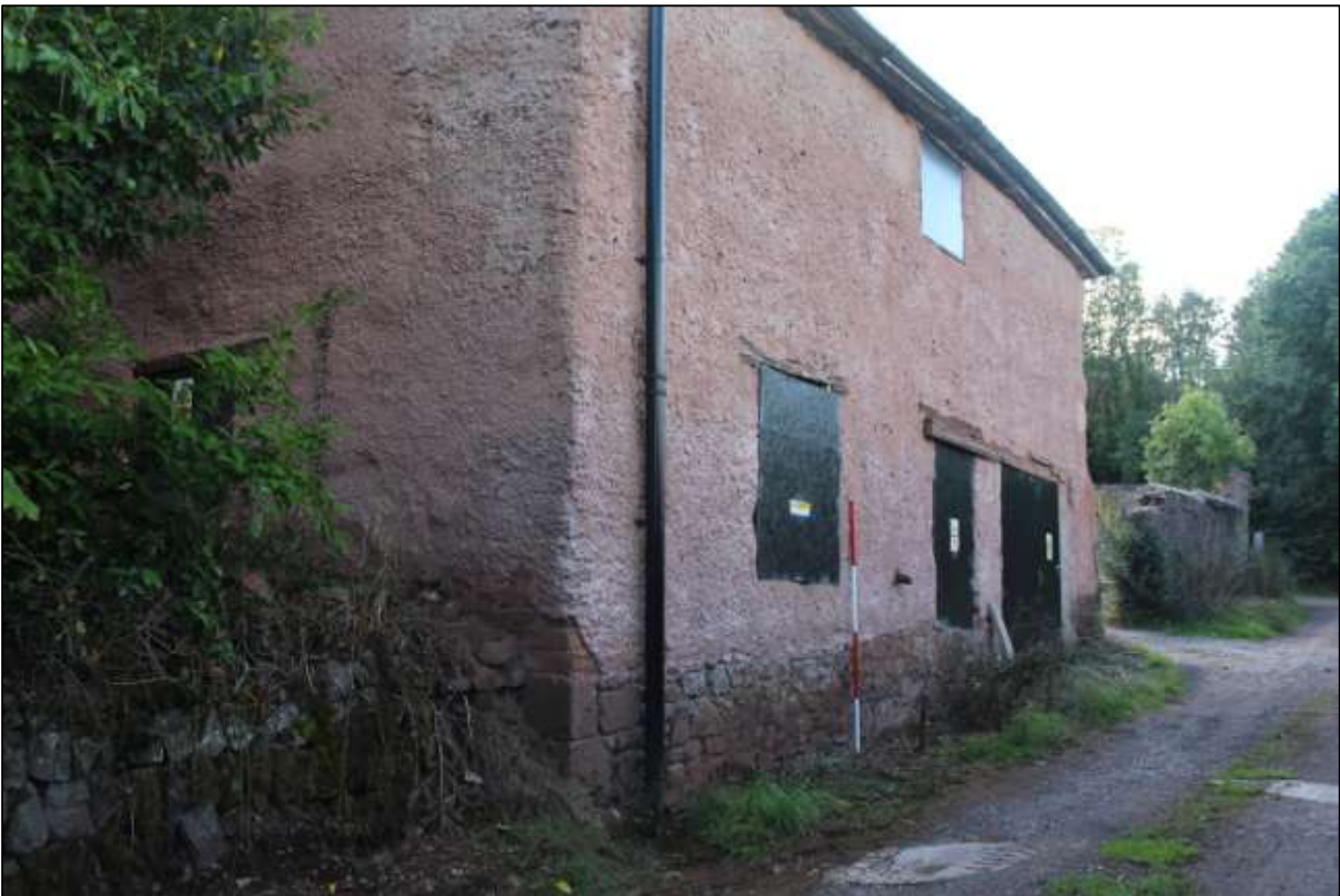
B1 EXTERIOR, THE NORTH AND EAST ELEVATIONS; VIEWED FROM THE NORTH-EAST (SCALE 2M).
