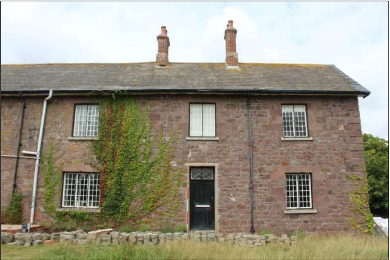
AS ABOVE, THE EASTERN (MORE RECENT) END OF THE FARMHOUSE; VIEWED FROM THE SOUTH (SCALE 2M).
