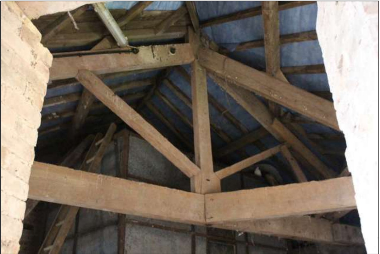
B5 FF INTERIOR; DETAIL OF THE KINGPOST ROOF STRUCTURE; VIEWED FROM THE NORTH-EAST.
