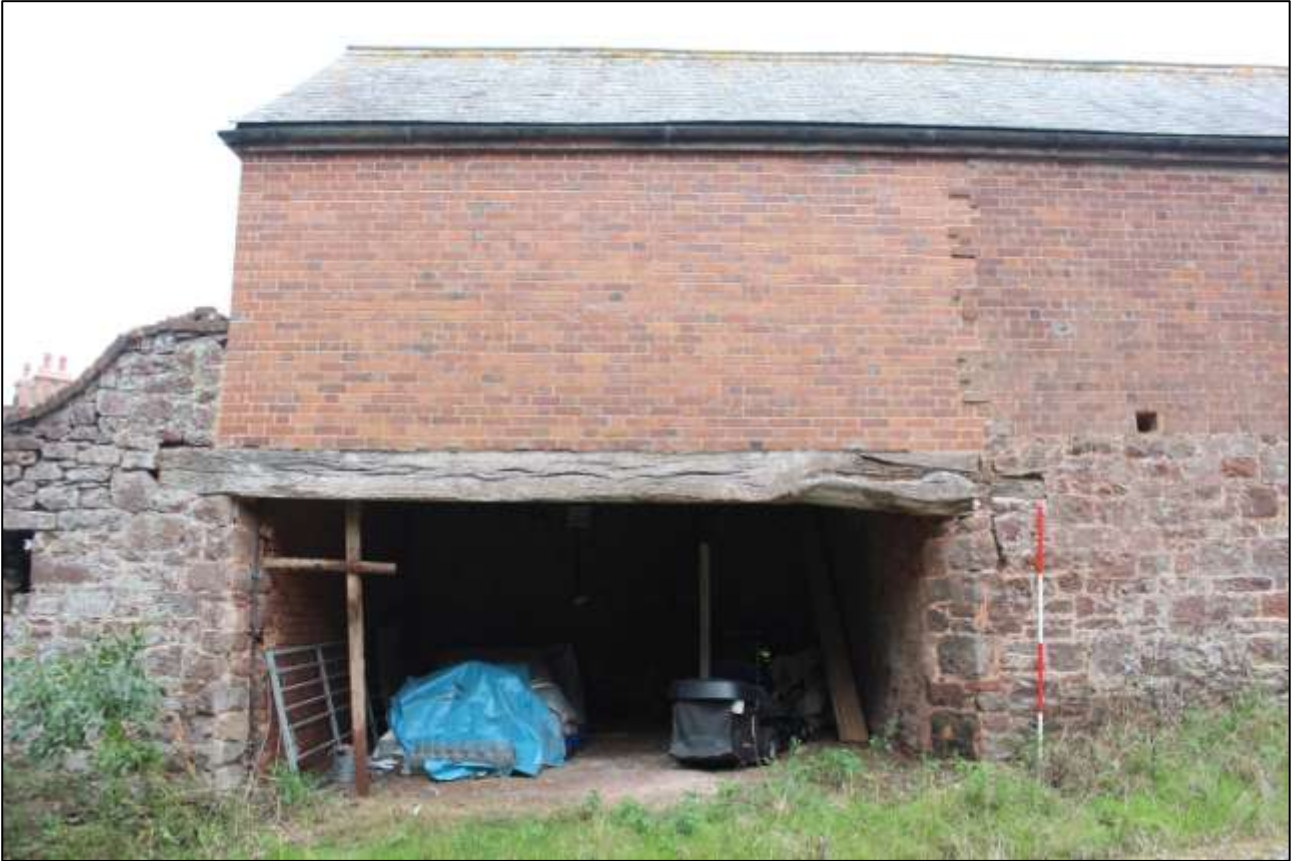
B4 EXTERIOR, NORTH-EAST END, SHOWING THE REBUILT WALL OVER THE CARTSHED OPENING TO B4B; VIEWED FROM THE NORTH-WEST (SCALE 2M).
