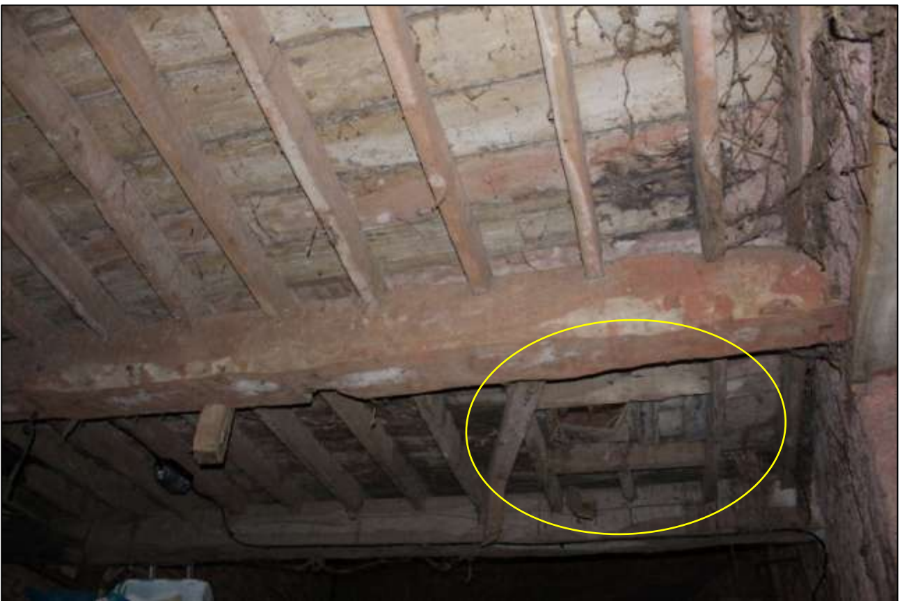
B1 GF INTERIOR, STRUCTURE OF THE GALLERY SHOWING THE HATCH (INDICATED); VIEWED FROM THE ENE AND BENEATH.
