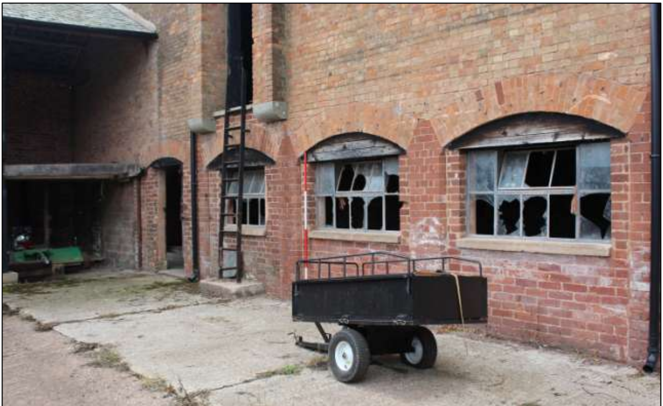
B6 EXTERIOR, EAST WALL, DETAIL OF THE BLOCKED GF OPENINGS; VIEWED FROM THE NORTH-EAST (SCALE 2M).
