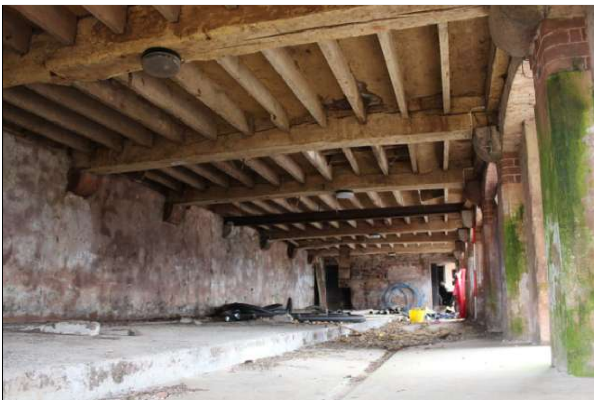
FIGURE 23: THE INTERNAL GROUND-FLOOR OF B6 SHOWING THE HEAVY ROOF STRUCTURE; VIEWED FROM THE SOUTH (SCALE 2M).
