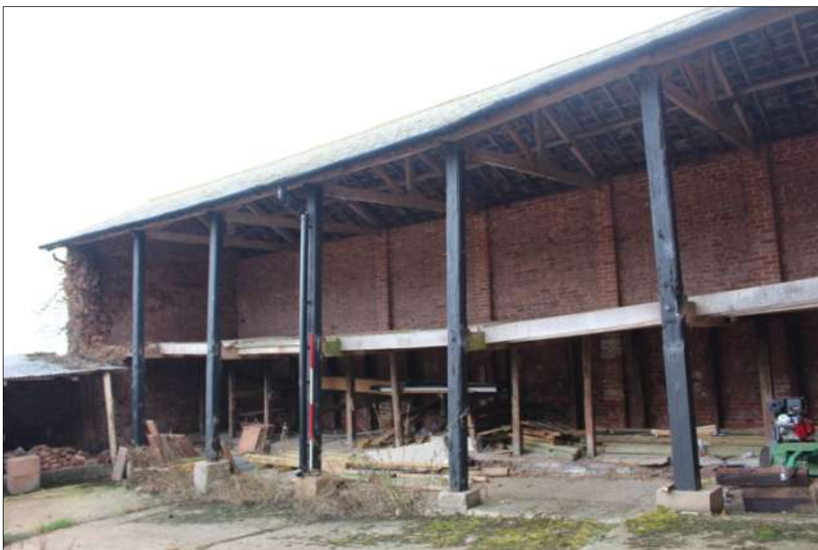
FIGURE 24: THE NORTH ELEVATION OF THE LINHAY; VIEWED FROM THE NORTH-WEST (SCALE 2M).
