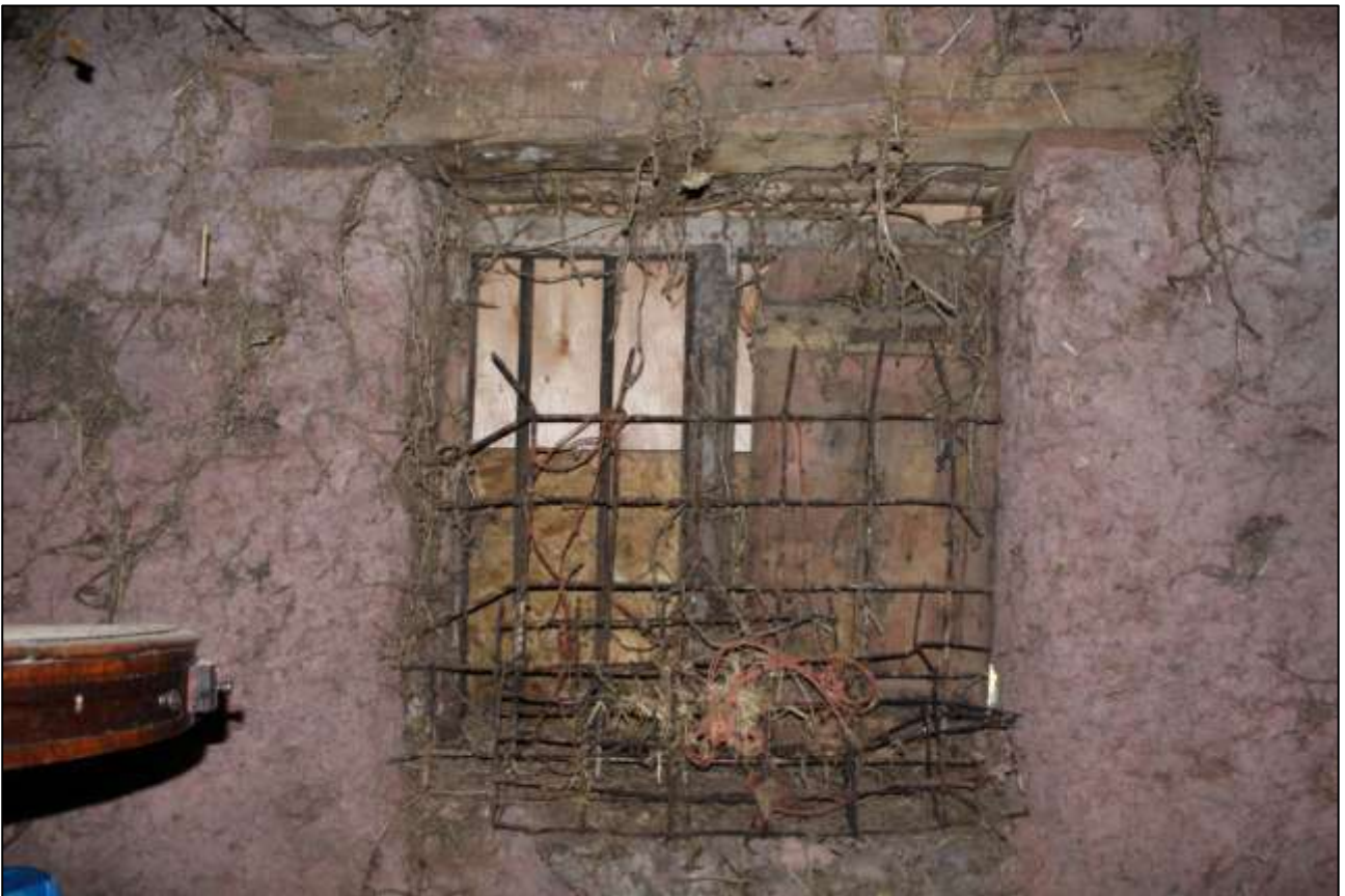
B2 GF INTERIOR, EAST WALL, DETAIL OF W8; VIEWED FROM THE WEST.
