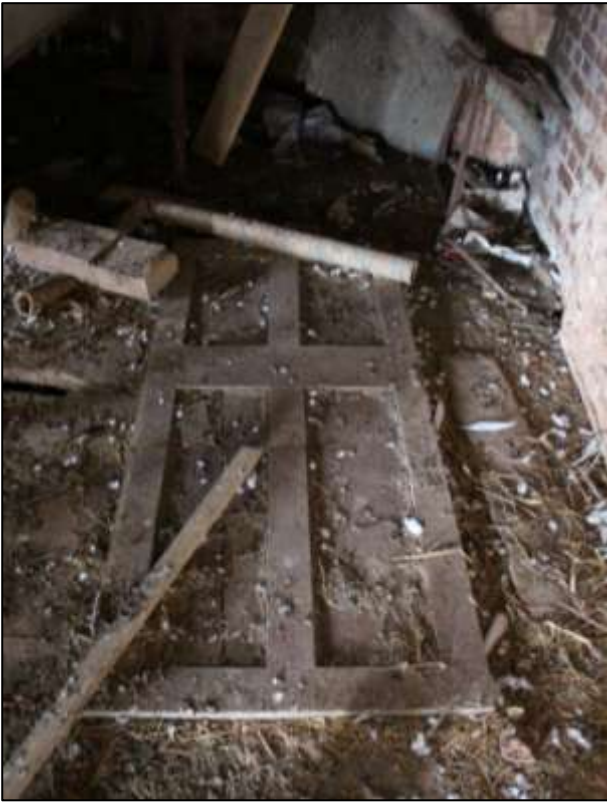
RIGHT: B5 FF INTERIOR, EX SITU DOOR ON THE FLOOR; VIEWED FROM THE EAST.
