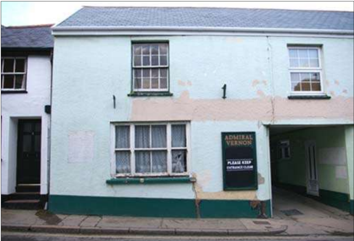
SOUTH ELEVATION, SHOWING HORNED SASH WINDOW TO GROUND FLOOR, AND HORNLESS SASH TO FIRST FLOOR; VIEWED FROM THE SOUTH.
