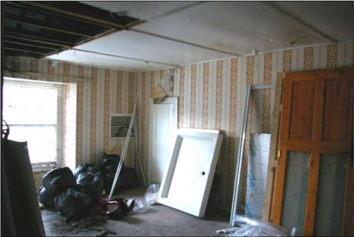
INTERNAL SOUTH AND WEST WALLS OF FR1 SHOWING DETAIL OF WALLPAPERING AND FULL HEIGHT CUPBOARD WITH D13 IN WEST WALL, AND SMALL CUPBOARD WITH D14 IN SOUTH WALL; VIEWED FROM THE NORTH-EAST (NO SCALE).
