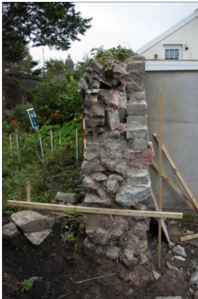
FIGURE 18: WALL {004}, NORTH FACING PROFILE WITH MODERN RETAINING/REPAIR {014}; VIEWED FROM THE NORTH (0.30M SCALE).
