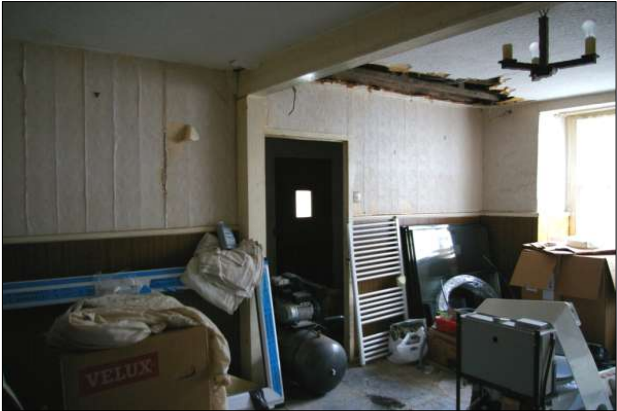
INTERNAL EAST WALL OF GR1 SHOWING WALLPAPERING, DADO RAIL AND IMITATION PANELLING, ALONG WITH DETAIL OF MODERN CEILING; VIEWED FROM THE NORTH-WEST (NO SCALE).
