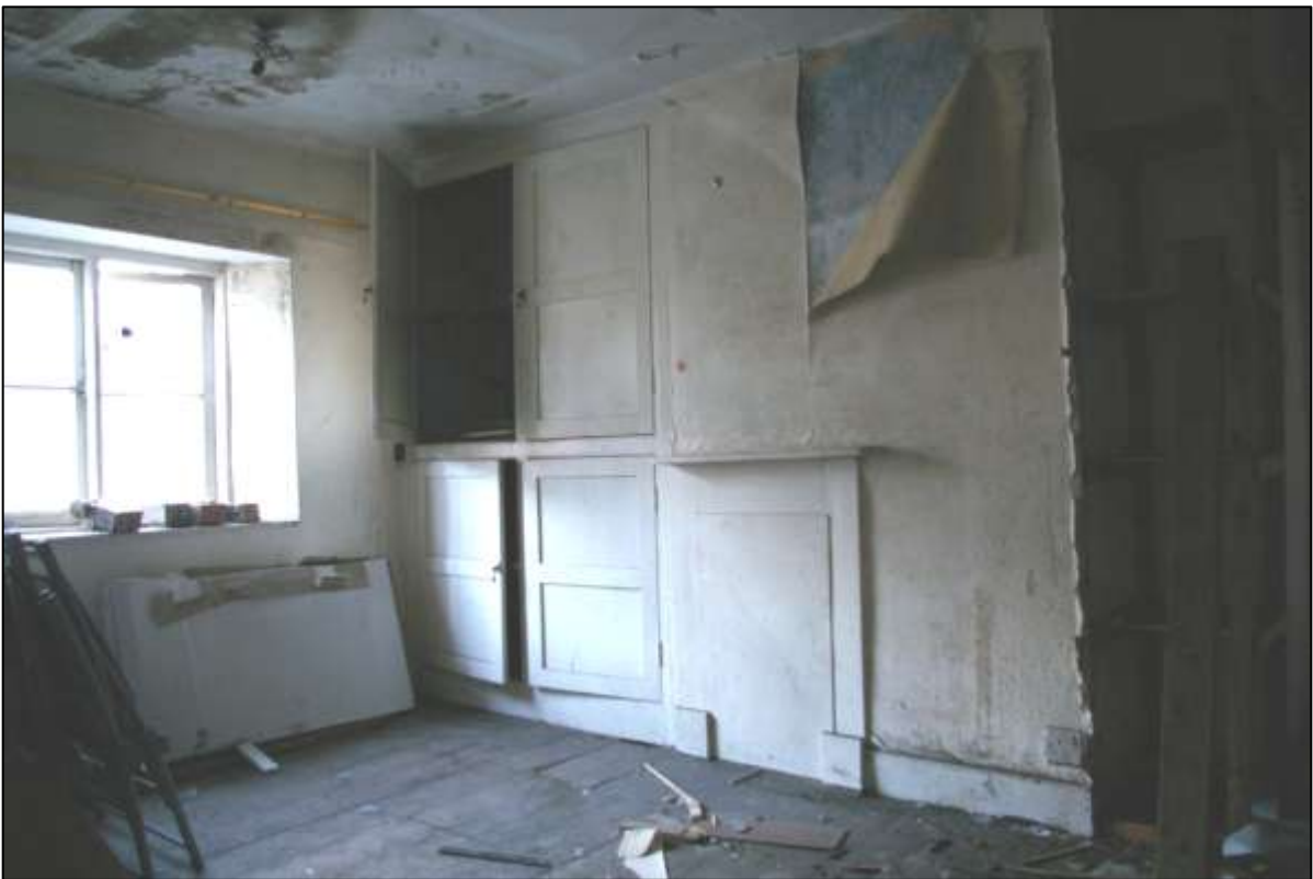
INTERNAL EAST WALL OF FR2 SHOWING BLOCKED FIREPLACE (FP3); VIEWED FROM THE NORTH-WEST (NO SCALE).
