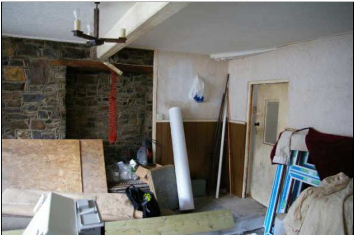
DETAIL OF INTERNAL WEST WALL OF GR1, NORTH END, SHOWING THE CENTRAL RECESS; VIEWED FROM THE SOUTH-EAST (NO SCALE).
