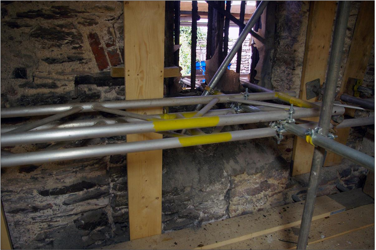
113. B2 FF INTERIOR, NORTH WALL, SHOWING W13 FORCED THROUGH THE BLOCKED FP2; VIEWED FROM THE SOUTH.
