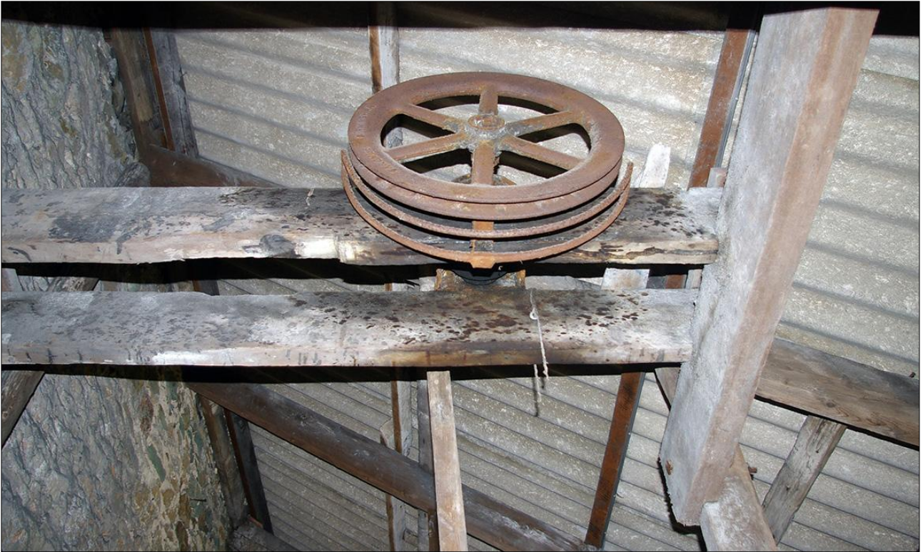
174. B3 FF INTERIOR, THE FLYWHEEL (S24) OVER HATCH S14; VIEWED FROM THE SOUTH.
