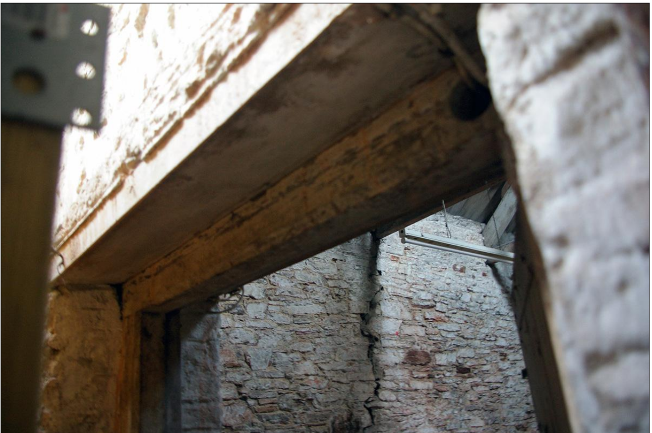
73. B1 FF R1, DETAIL OF THE DOORFRAME TO D20; VIEWED FROM THE SOUTH-EAST.
