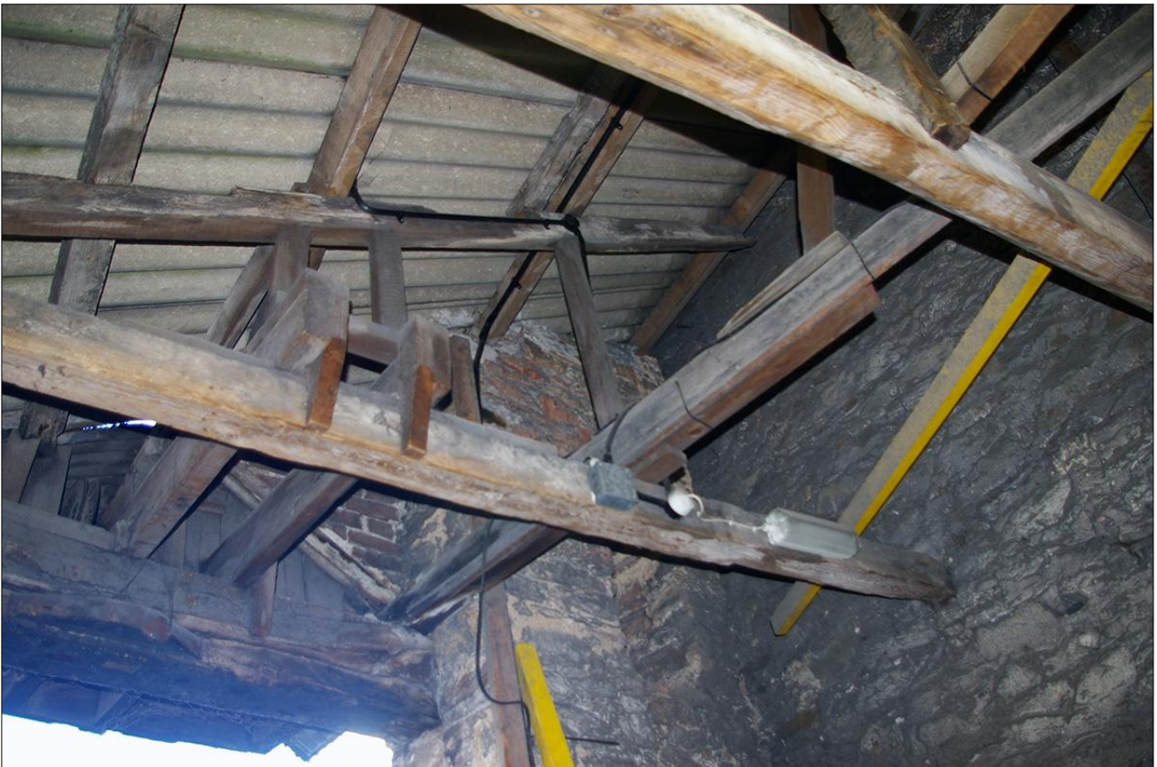
169. B3 FF INTERIOR, THE ROOF STRUCTURE OVER THE SOUTHERN END AND BEAMS FOR HOIST (S23); VIEWED FROM THE NNE.
