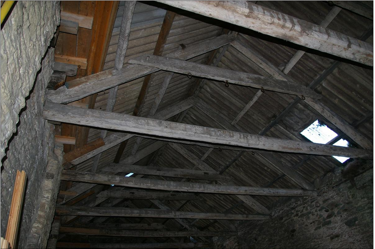
132. AS ABOVE, THE NORTHERN HALF OF THE ROOF; VIEWED FROM THE SOUTH.
