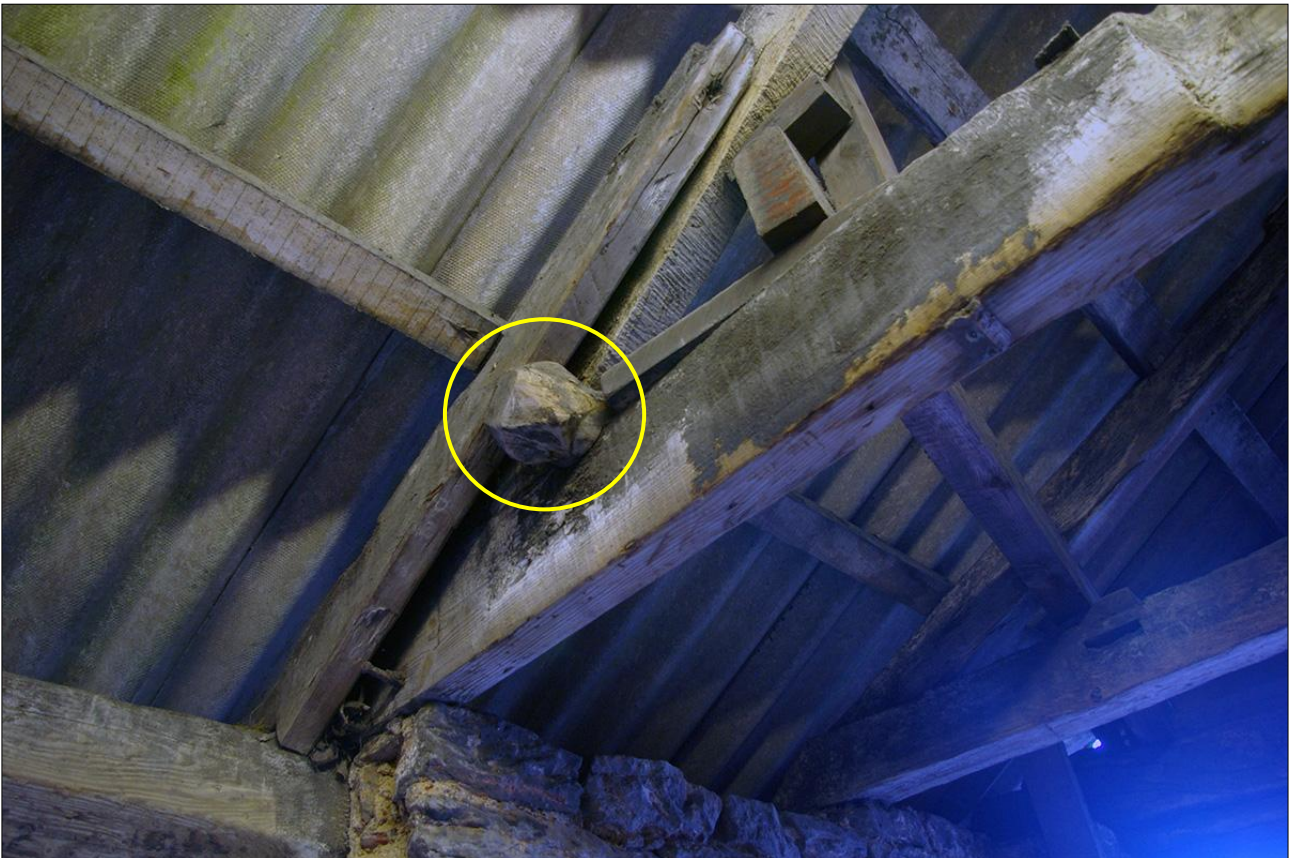
171. B3 ROOF STRUCTURE, SHOWING THE RE-USED SHAPED TIMBER (INDICATED) (S12); VIEWED FROM THE NNW.
