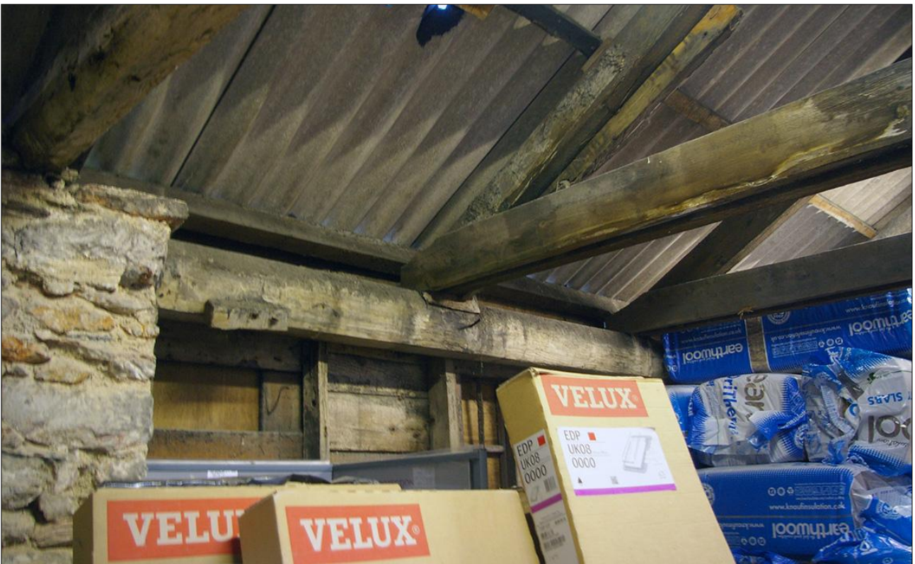
182. B3 FF INTERIOR, SHOWING ORIGINAL WOODEN FRAMEWORK TO BO17; VIEWED FROM THE WNW.
