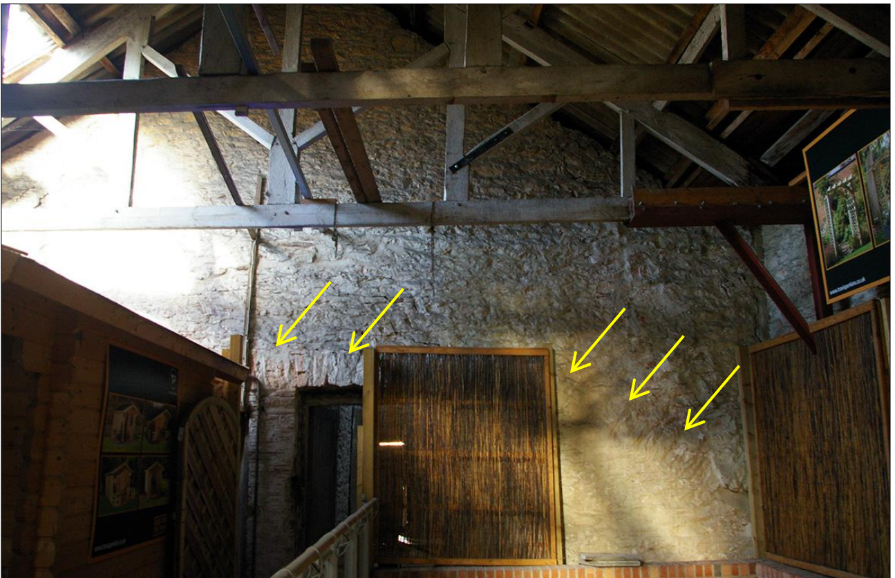
68. B1 FF R1, THE NORTH WALL SHOWING D19 BELOW THE WIDE RELIEVING ARCH (INDICATED); VIEWED FROM THE SOUTH.
