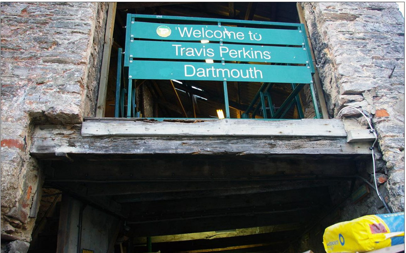
142. THE SOUTH ELEVATION OF B3, SHOWING THE LINTEL OVER D13; VIEWED FROM THE SOUTH.
