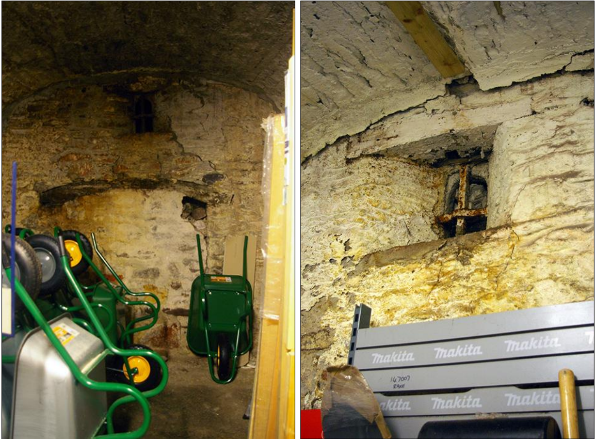
LEFT FIGURE 21: BO5 IN VAULT 5, WITH CURVING TIMBER LINTEL AND W5 ABOVE; VIEWED FROM THE EAST. RIGHT FIGURE 22: DETAIL OF W2 IN VAULT 2, WITH IRON FERRAMENTA; VIEWED FROM THE ENE.
