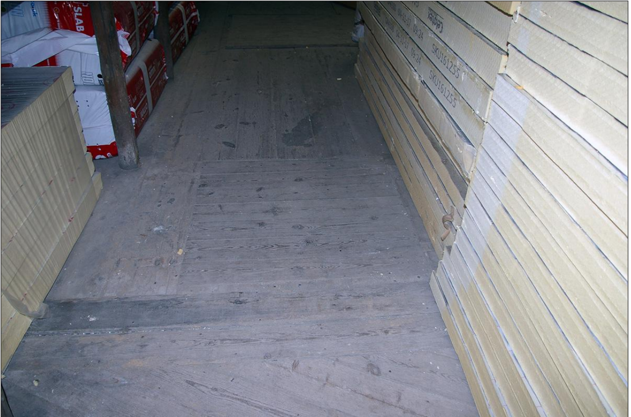
179. B3 FF INTERIOR, HISTORIC FLOORBOARDS (S13) AND HATCH (S14); VIEWED FROM THE NORTH.
