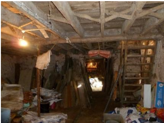
Interior of cellar (west range) showing first floor construction and steps up to granary
