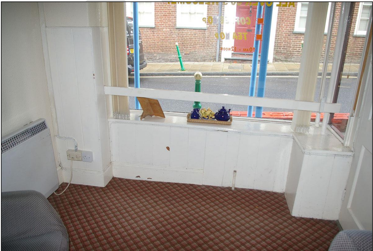
18. THE SURVIVING BEADED PLANK PANELLING UNDER WINDOW AND TO SOUTH WALL, SOUTH-EAST CORNER OF R2; FROM THE NORTH.
