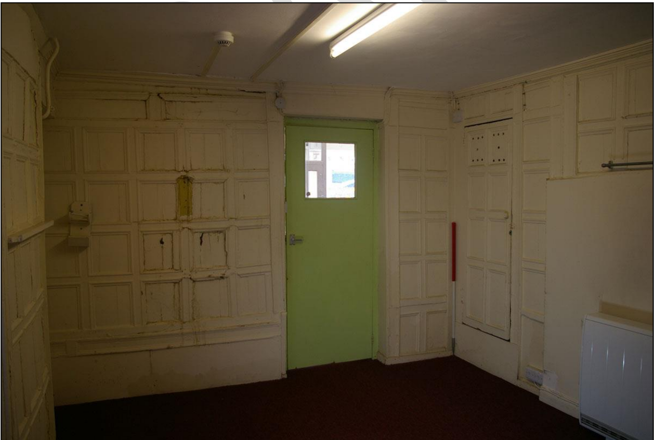
64. THE SOUTH AND WEST WALLS, D24 AND CUPBOARD, WITH 1M SCALE; FROM THE NORTH-EAST.
