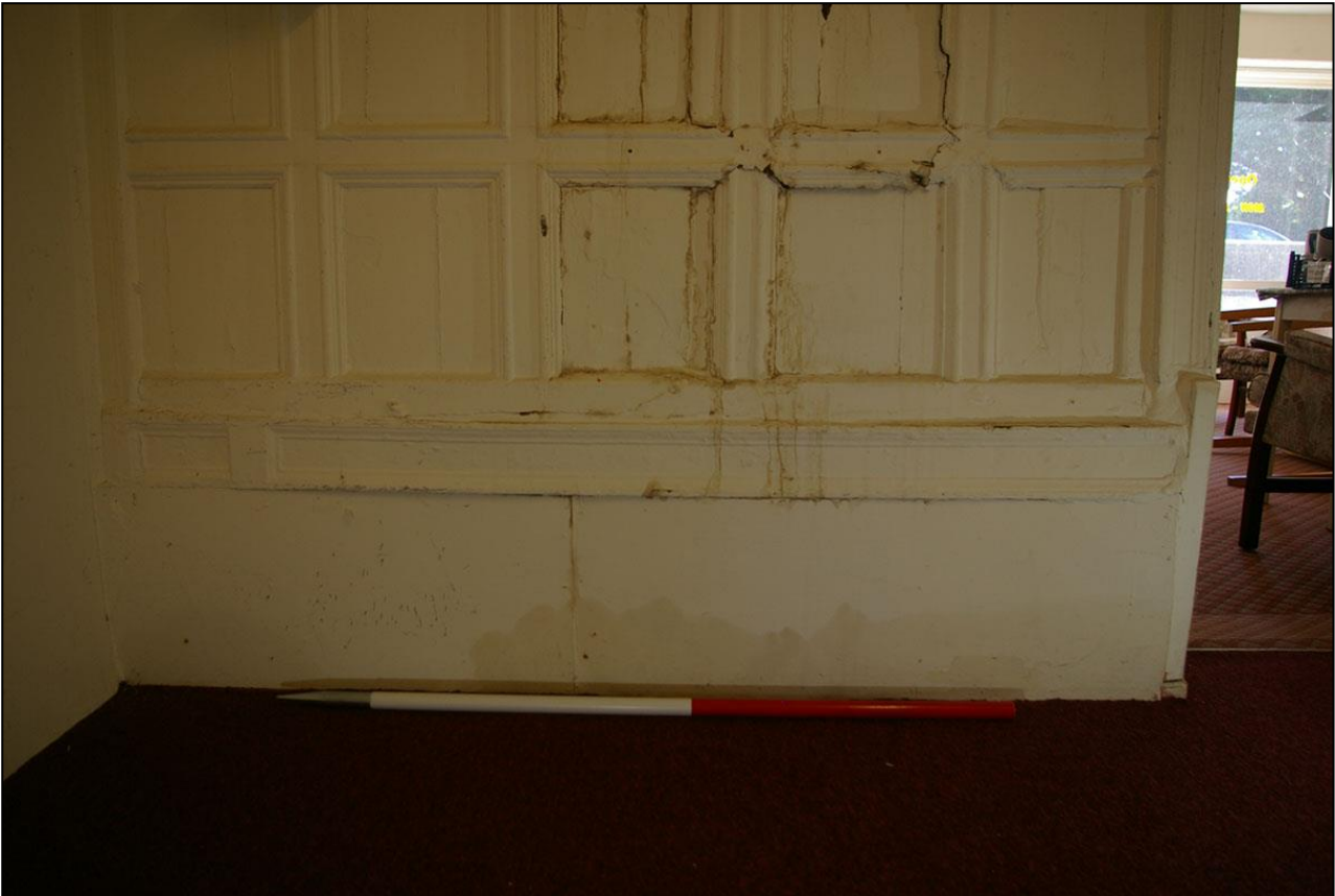
87. THE BASE OF THE SOUTH WALL, WITH 1M SCALE; FROM THE NORTH.
