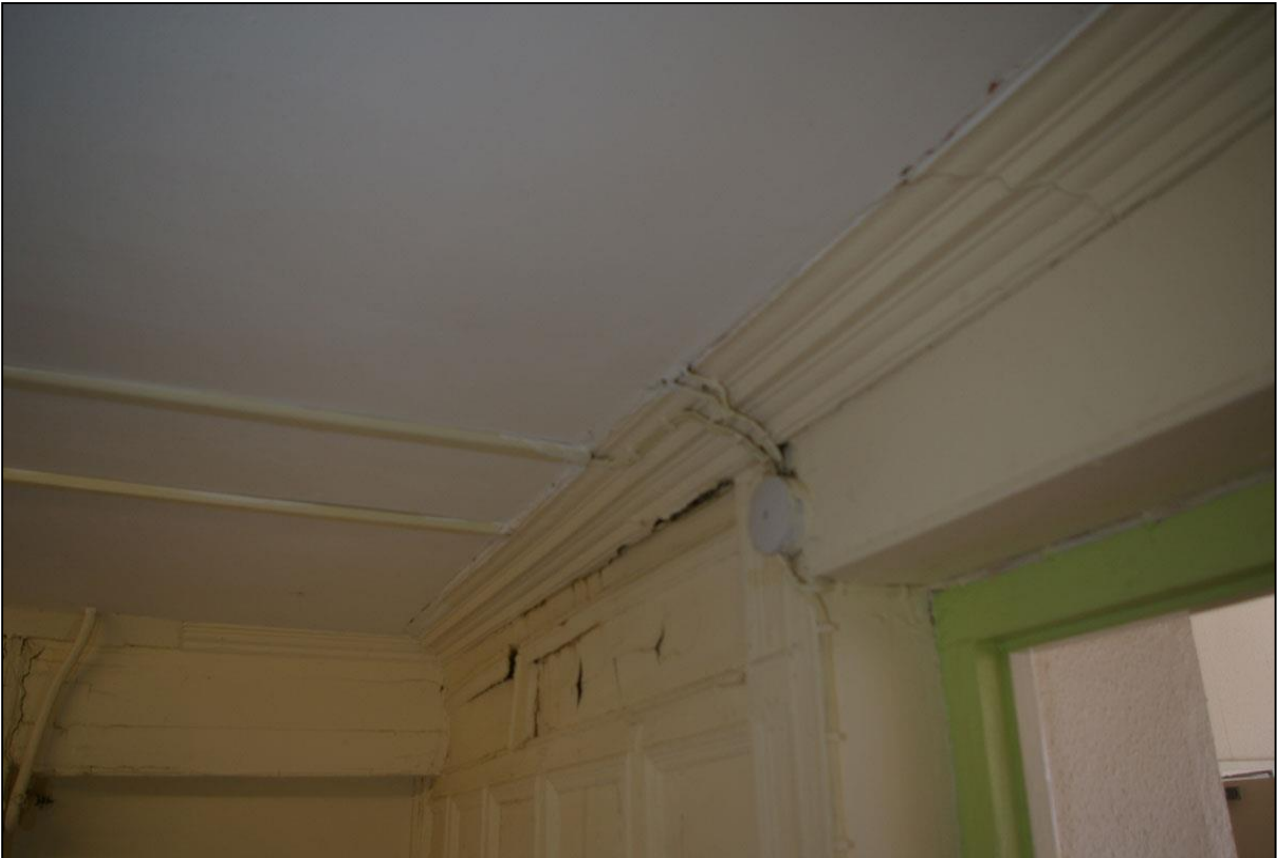
85. THE COMPLEX DEEP CORNICE OF OGEE, CAVETTO, OVULO AND BEADING, ALONG THE SOUTH WALL; FROM THE WEST-NORTH-WEST.
