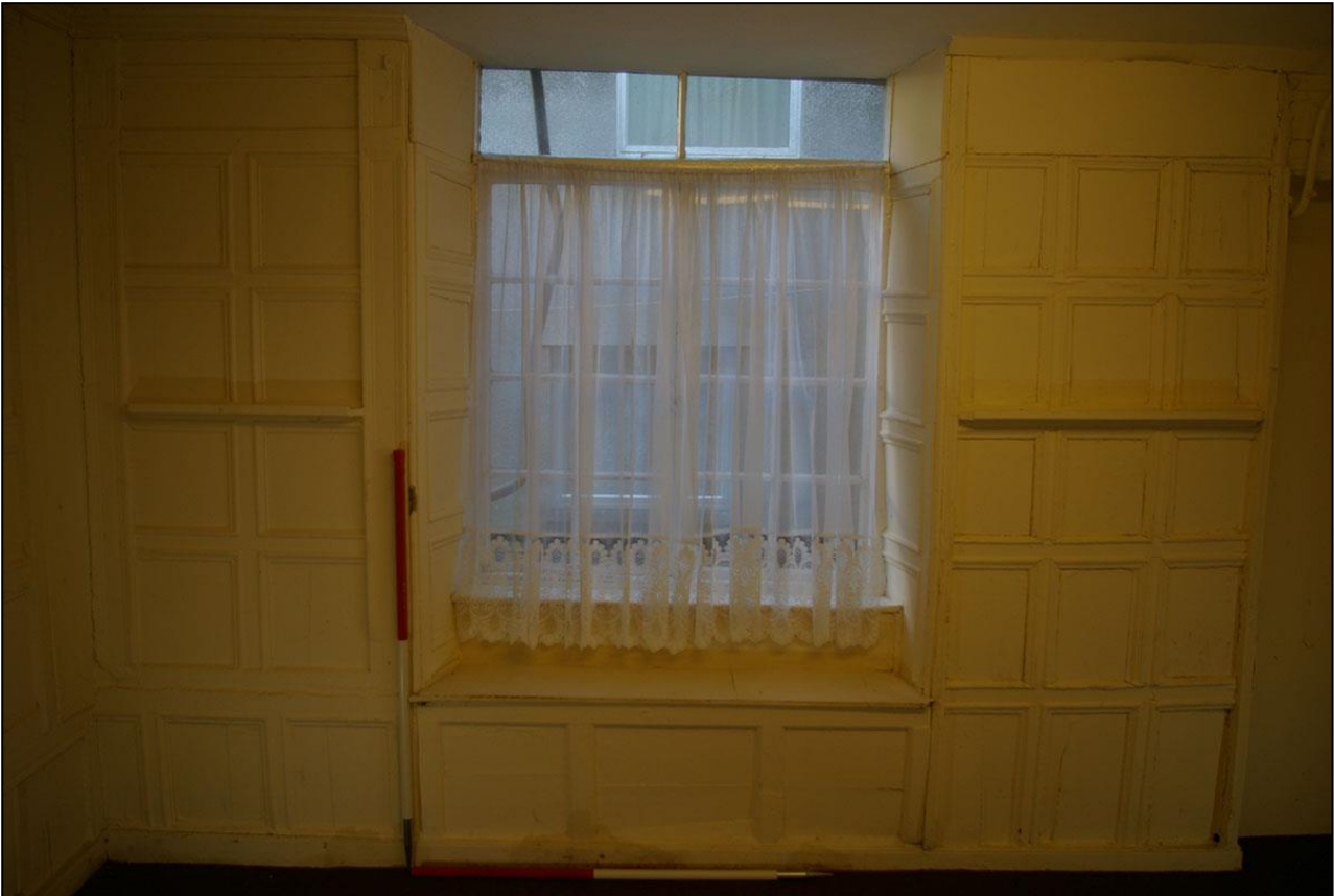
61. THE EAST WALL AND W13 WITH 2 X 1M SCALES; FROM THE WEST.
