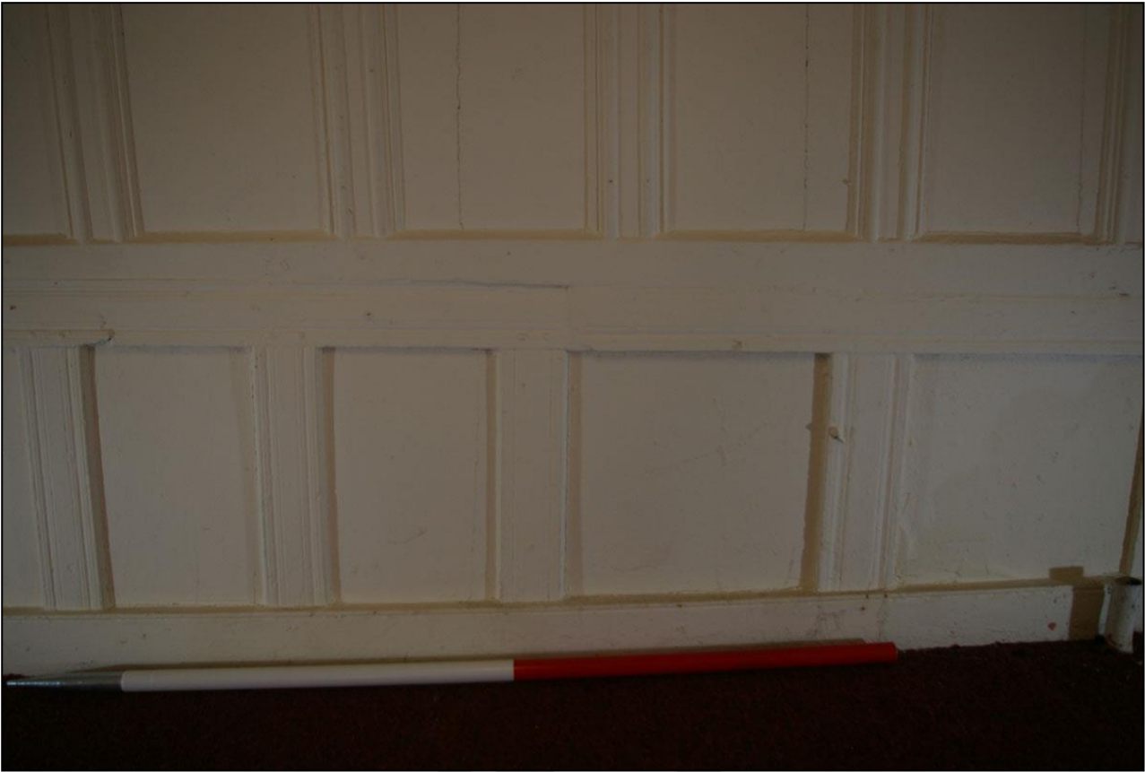
71. THE CUT AND DAMAGED SECTION OF PANELLING, WITH 1M SCALE; FROM THE SOUTH.
