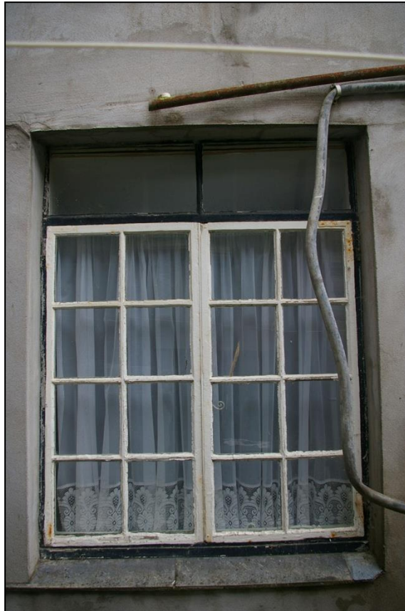
35. W13, 19 TH CENTURY CASEMENT WITH GLASS FILLET ABOVE, INFILLING AN ORIGINALLY TALLER OPENING; FROM THE EAST.
