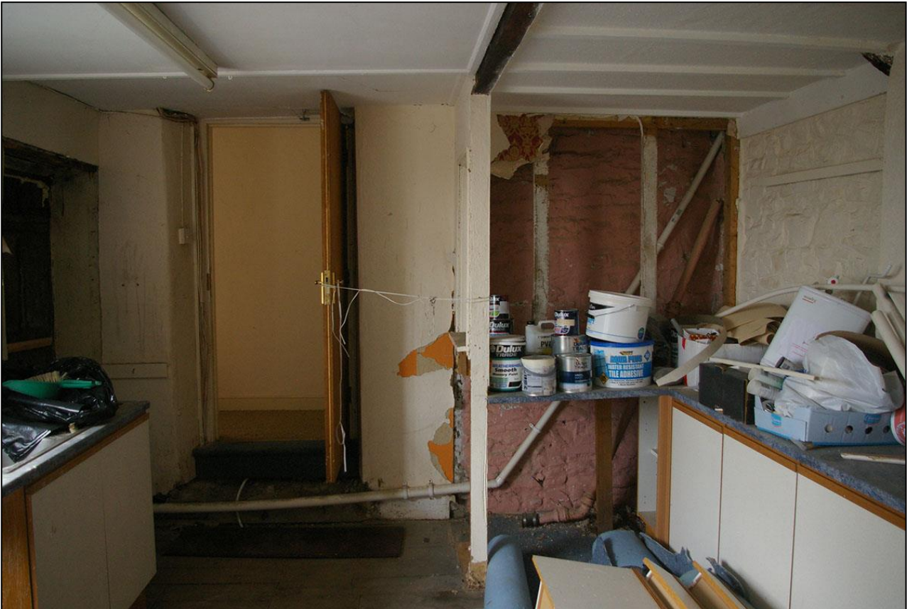
49. THE SOUTH PARTY WALL BETWEEN BUILDING 1 AND BUILDING 2, WITH FORCED DOOR, D29; FROM THE NORTH.
