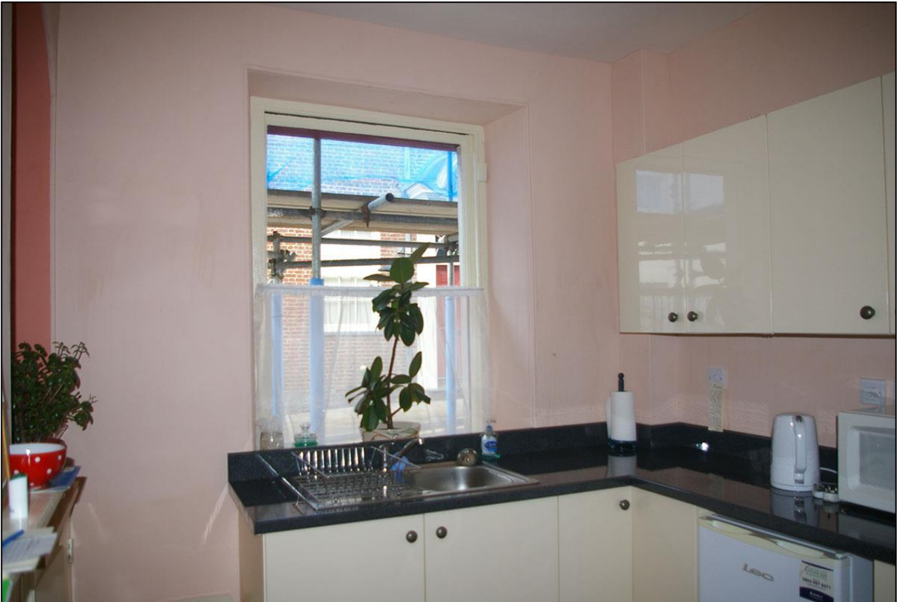
15. THE SASH WINDOW IN THE SOUTH WALL, WITHIN BEADED OPENING; FROM THE NORTH-EAST.
