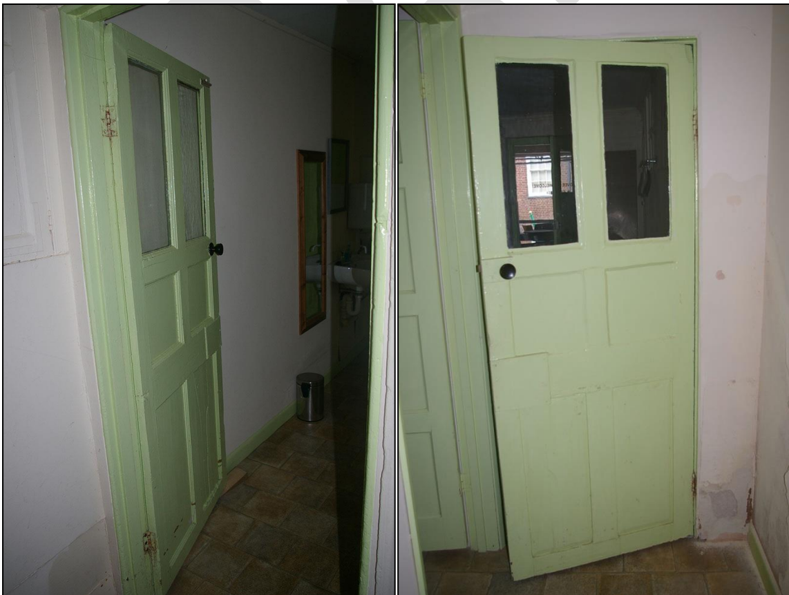
40. LEFT & RIGHT: D25, BETWEEN R17 AND R19, 18TH CENTURY STYLE DOOR WITH TWO GLASS PANES INSERTED; FROM THE SOUTH-EAST AND NORTH.
