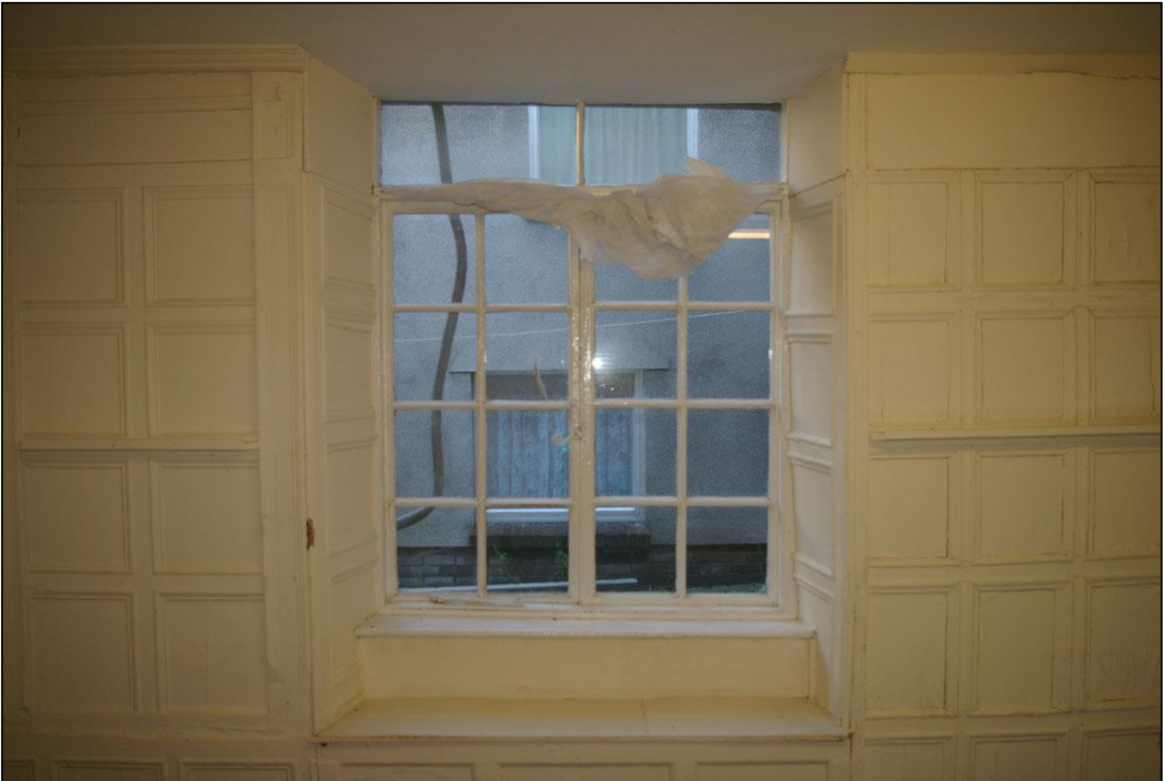
37. W13, WITH RECYCLED AND RESET 18 TH CENTURY PANELLED SECTIONS TO THE SIDES, SHUTTERS, CUT AND NAILED SHUT AND WINDOW SEAT; FROM THE WEST.
