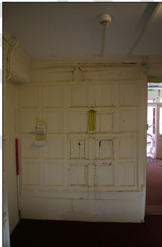
84. THE SOUTH WALL, EAST END, WITH 1M SCALE, D7 AND D24, SHOWING THE WATER DAMAGE TO THIS WALL; FROM THE NORTH.
