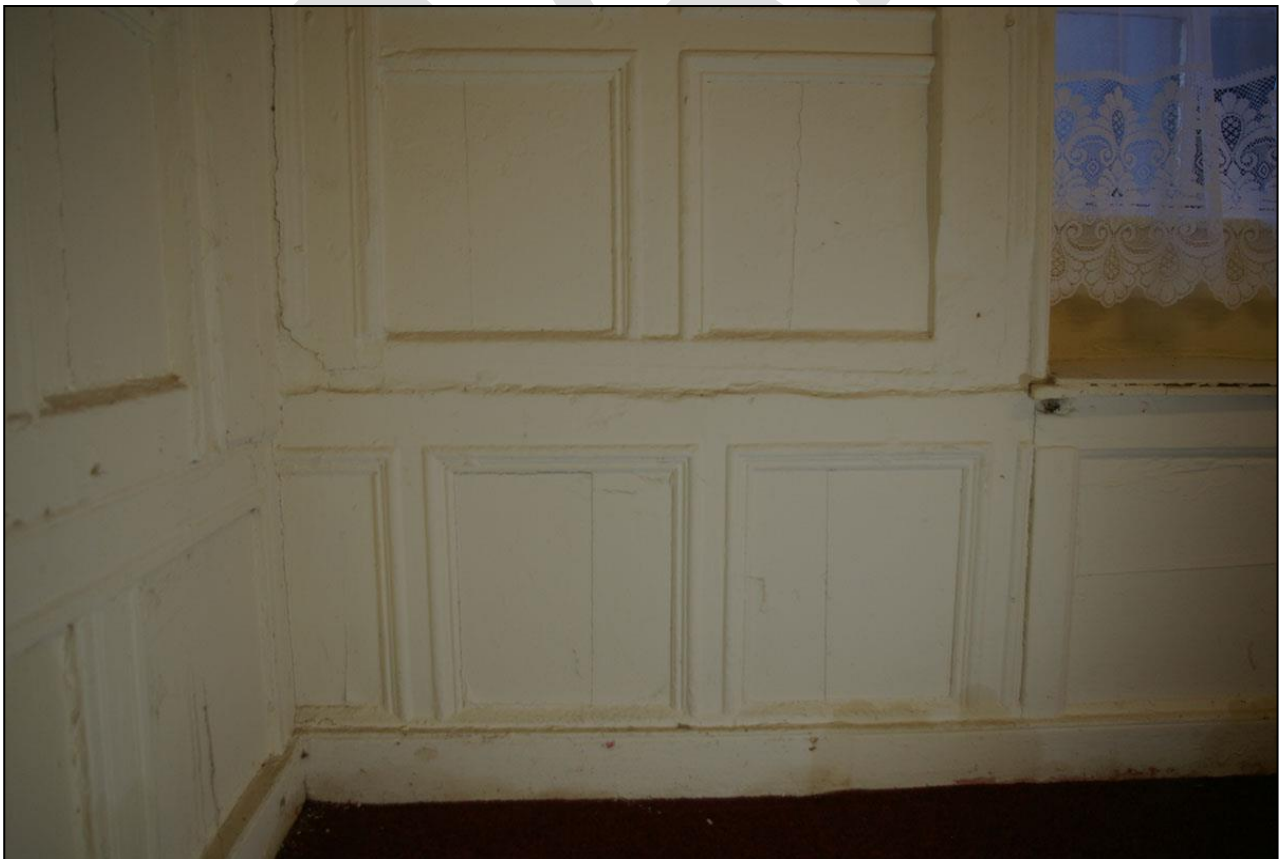
76. THE RAGGED JOINTS BETWEEN THE SECTIONS OF PANELLING ON THE EAST WALL; FROM THE WEST
