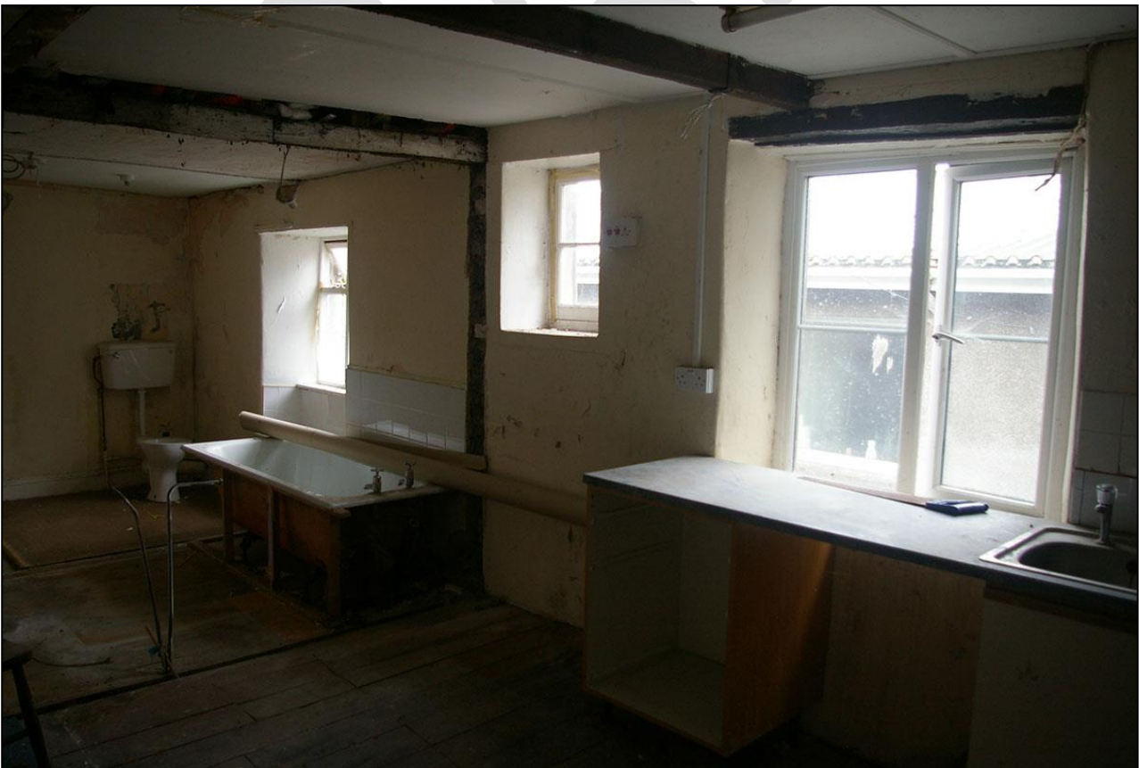
48. THE EAST WALL, ROOM 20, SHOWING W17, W18 AND W19; FROM THE SOUTH-WEST.
