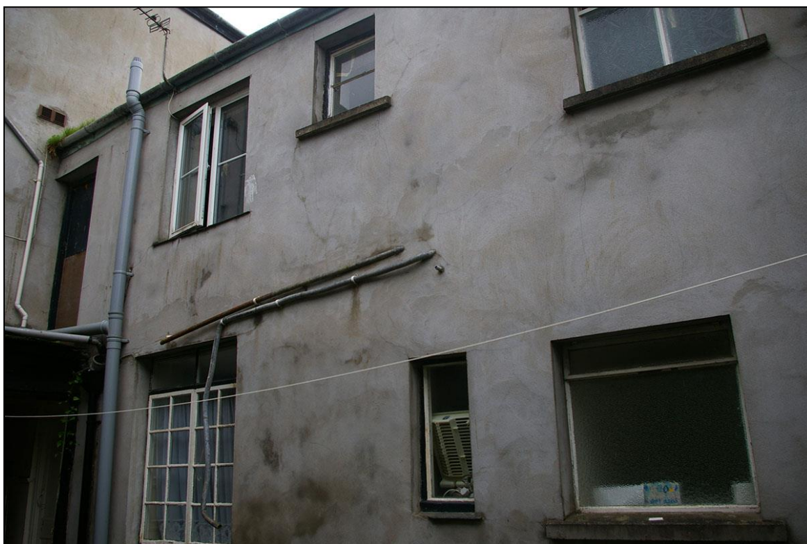
FIGURE 6: THE EAST ELEVATION OF BUILDING 2, SHOWING THE MODERN CHARACTER; FROM THE NORTH-EAST
