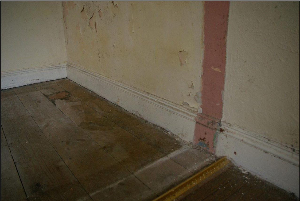
57. THE BEADED SKIRTING, IN ROOM 20, VICTORIAN IN STYLE WHICH RUNS ALONG THE WEST AND NORTH WALLS OF BR4; FROM THE EAST.
