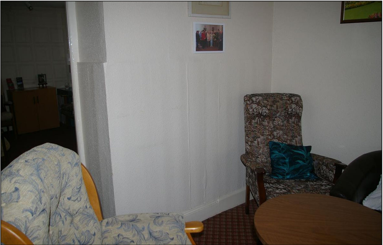
19. THE SURVIVING BEADED PLANK PANELLING IN THE NORTH-EAST CORNER OF R2, RUNNING INTO THE FORCED DOORWAY OPENING, PAPERED OVER WITH WOODCHIP WALLPAPER; FROM THE SOUTH-WEST.
