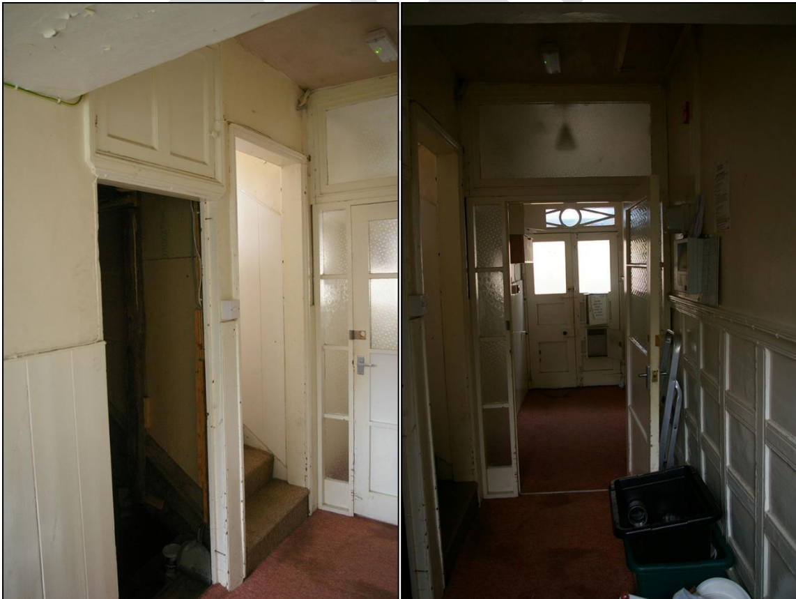
7. LEFT: THE EAST WALL OF R1A, WITH THE DOOR TO THE COLD STORE AND THE STAIRCASE; FROM THE NORTH-WEST. 8. RIGHT: VIEW FROM THE REAR DOOR OF THE CROSS PASSAGE LOOKING TO THE FRONT DOORS; FROM THE NORTH.
