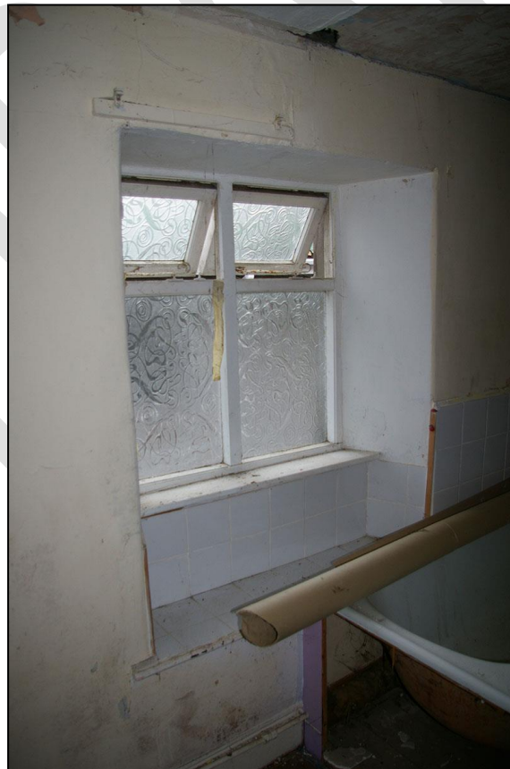
52. W19, SHOWING THE LOWERED WINDOW SEAT BEHIND THE BATH; FROM THE NORTH-WEST.
