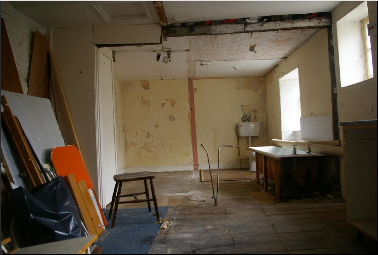
47. ROOM 20, SHOWING THE REMOVAL OF PARTITIONS INSTALLED IN THE MID-20 TH CENTURY TO FORM A STUDIO STYLE FLAT; FROM THE SOUTH.
