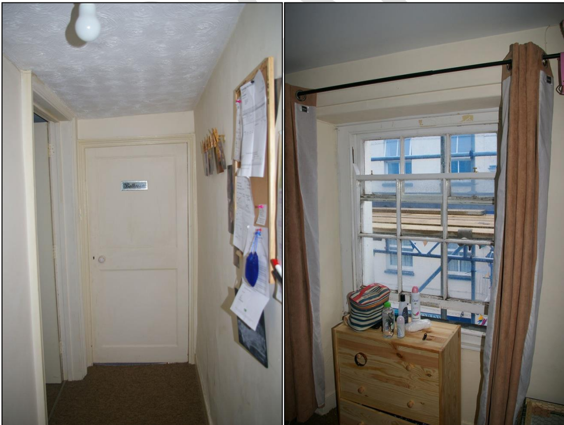
31. LEFT: THE FLAT TWO PANEL MOULDED 18 TH CENTURY DOOR, RESET HERE IN AN AWKWARDLY REFITTED MOULDED FRAME; BETWEEN R12 AND R16 IN THE SECOND FLOOR FLAT; FROM THE EAST.
