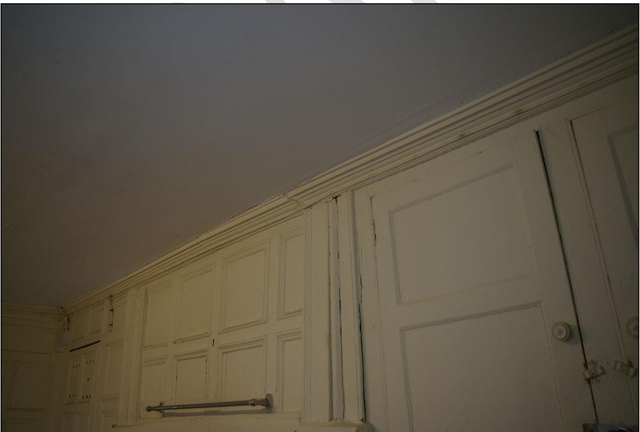
97. THE CUT AND RESET WOODEN CORNICE ALONG THE WEST WALL; FROM THE NORTH, NORTH-EAST
