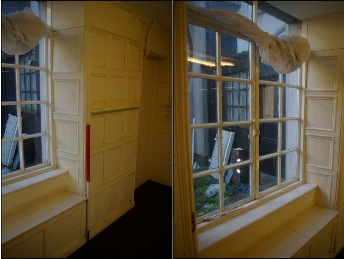
80. LEFT: THE PANELLED SHUTTERS TO THE SOUTH SIDE OF W13, WITH 1M SCALE; FROM THE NORTH-NORTH-EAST.
