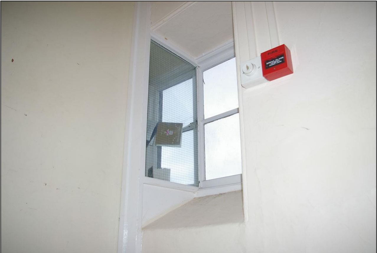
30. THE SMALL, TWO LIGHT CASEMENT WINDOW WHICH LIGHTS THE SECOND FLOOR LANDING; FROM THE SOUTH-EAST.
