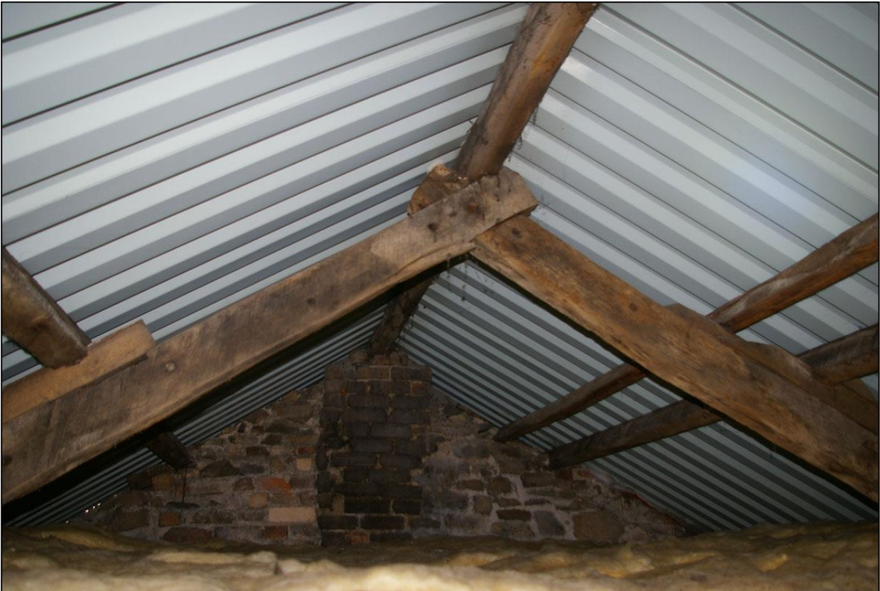
59. THE ROOF STRUCTURE OVER BUILDING 2, SHOWING REUSED BLADES IN THE TRUSSES AND PEGGED RIDGE, THE NORTHERNMOST TRUSS OF 3; FROM THE SOUTH-WEST.
