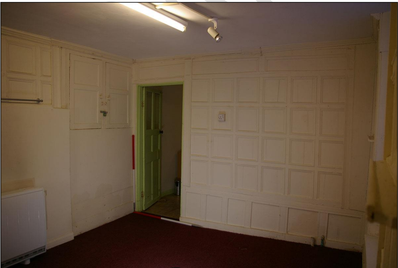
66. THE WEST AND NORTH WALLS, WITH 2 X 1M SCALE, WITH D25 AND BLOCKED FIREPLACE AND CUPBOARD; FROM THE SOUTH-EAST.
