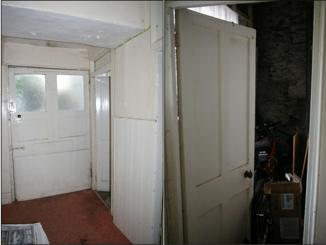
5. LEFT: THE DOOR TO R4, FROM WITHIN R1A, THE REAR PART OF THE CROSS PASSAGE; FROM THE SOUTH-WEST. 6. RIGHT: PLAIN FOUR PANEL 19 TH CENTURY DOOR TO ROOM 4; FROM THE WEST, SOUTH-WEST
