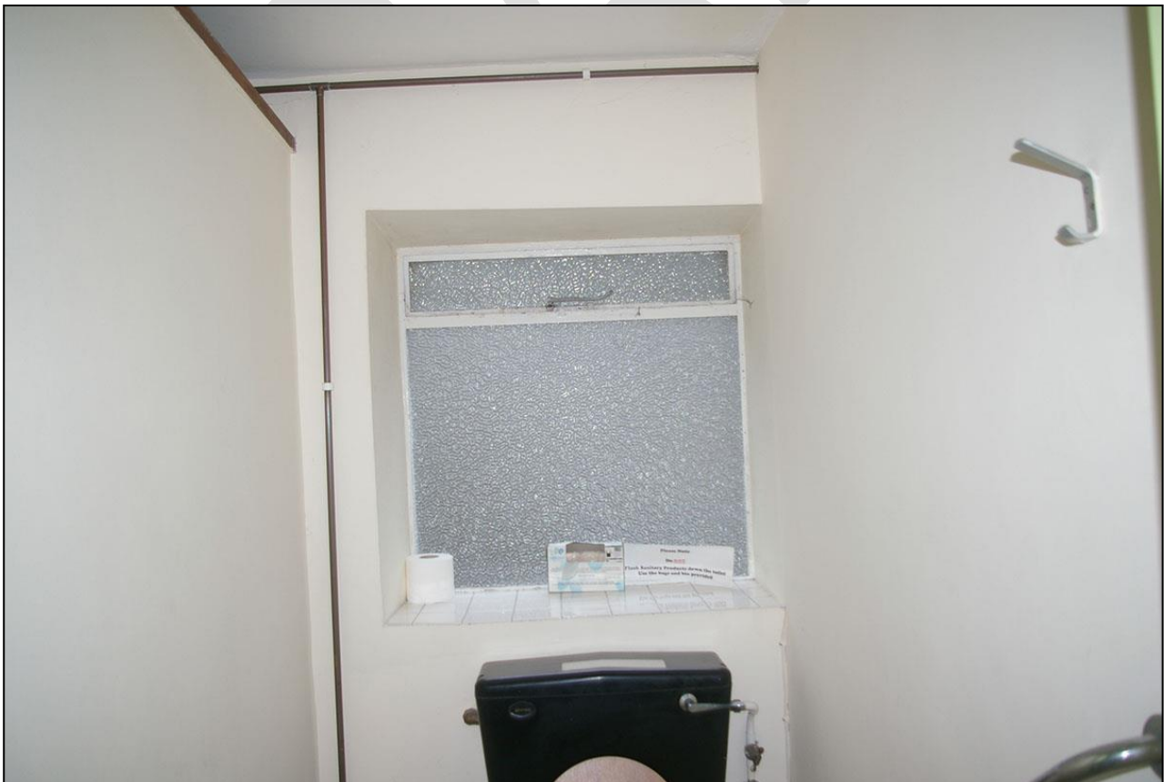
43. W15, ONE OF THE METAL FRAMED CRITTAL-STYLE WINDOWS IN ROOM 19; FROM THE WEST.
