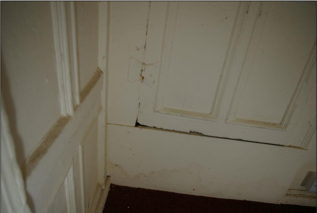
94. THE BUTTERFLY HINGES TO THE CUPBOARD IN THE SOUTH-WEST CORNER OF ROOM 17; FROM THE EAST.
