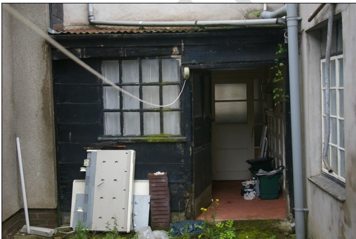
FIGURE 3: THE BEADED PLANK TIMBER STRUCTURE WHICH ENCLOSES THE GROUND FLOOR OF THE REAR ELEVATION; FROM THE NORTH.
