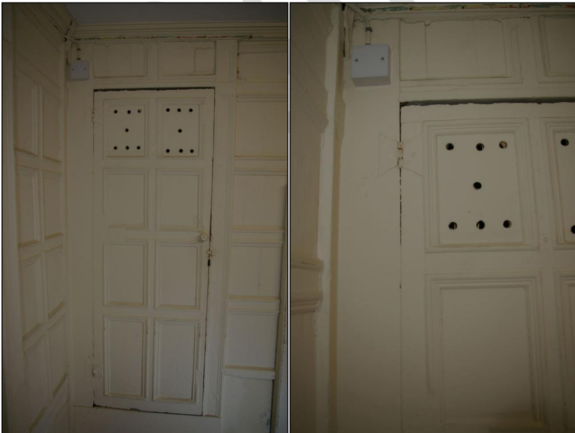
92. LEFT: THE FINE PANNELLED DOOR TO THE SOUTH OF THE WEST WALL; FROM THE EAST
