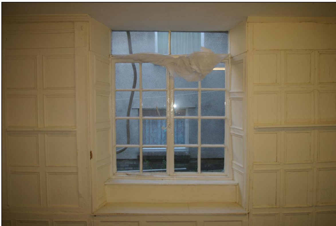
FIGURE 7: W13 IN ROOM 17, WITH RECYCLED AND RESET 18TH CENTURY PANELLED SECTIONS TO THE SIDES, SHUTTERS, CUT AND NAILED SHUT, AND EARLY 19TH CENTURY PANELLING FORMING A WINDOW SEAT; FROM THE WEST.
