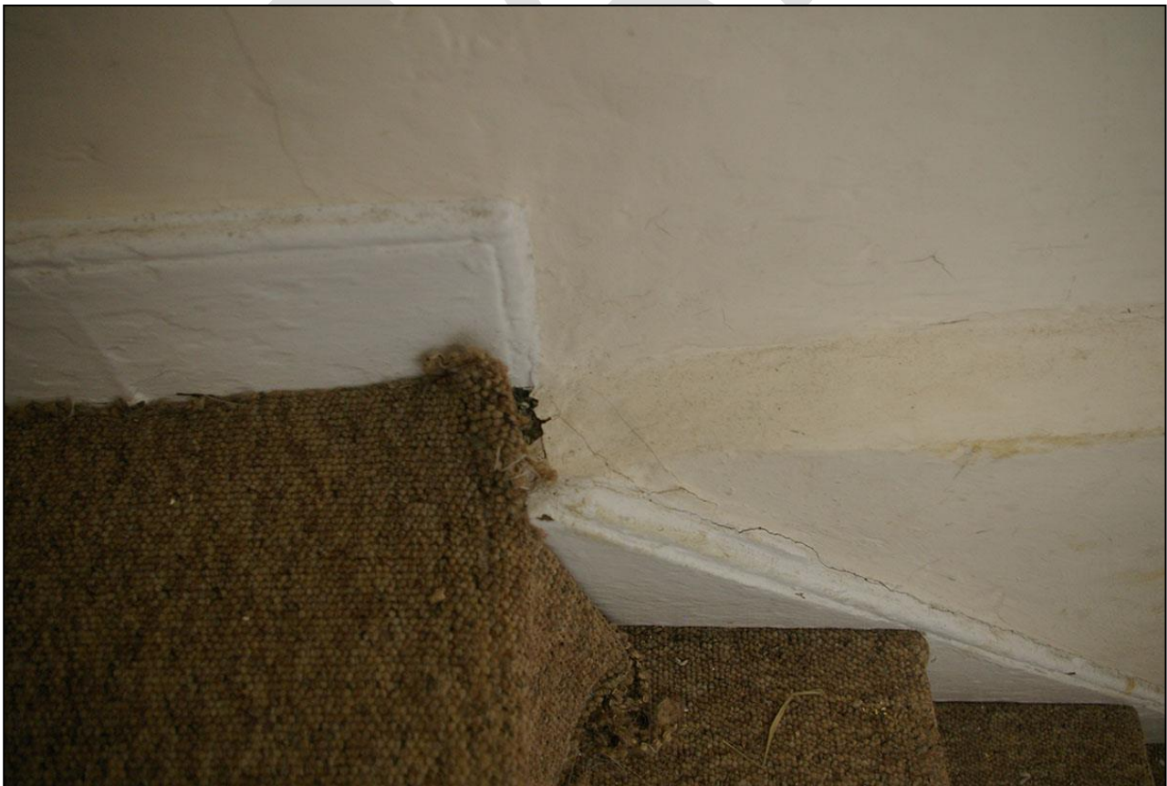
23. THE THICK SECTION OF GROUND FLOOR WALL, SHOWING A LEDGE DESIGNED FOR A FIRST FLOOR, SHOWING THIS STAIRCASE IS INSERTED INTO AN EARLIER SECTION OF BUILDING; FROM THE SOUTH-WEST.
