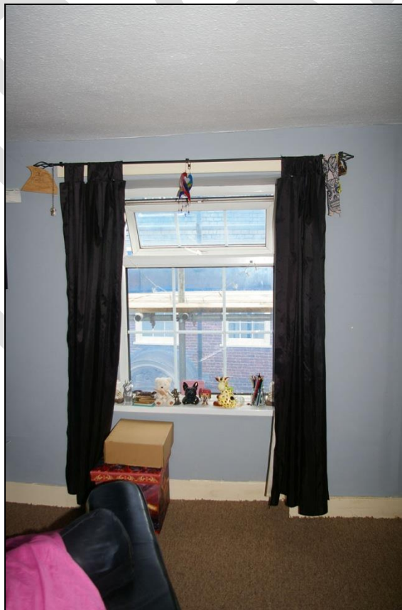
34. THE PVC SASH EFFECT MODERN WINDOW FITTED TO THE WESTERNMOST WINDOW IN THE FRONT WALL OF THE SECOND FLOOR LEVEL, ROOM 15; FROM THE NORTH, NORTH-WEST.
