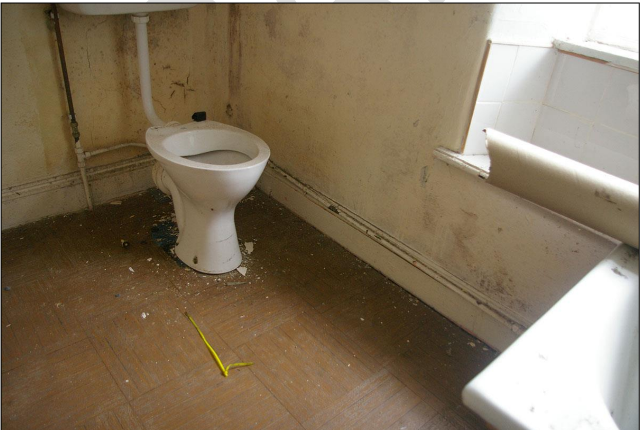
58. R20, THE BEADED SKIRTING RUNS BEHIND, AND IS CUT BY, THE MID-20 TH CENTURY TOILET SUGGESTING IT MAY BE VICTORIAN OR EDWARDIAN; FROM THE SOUTH-WEST.
