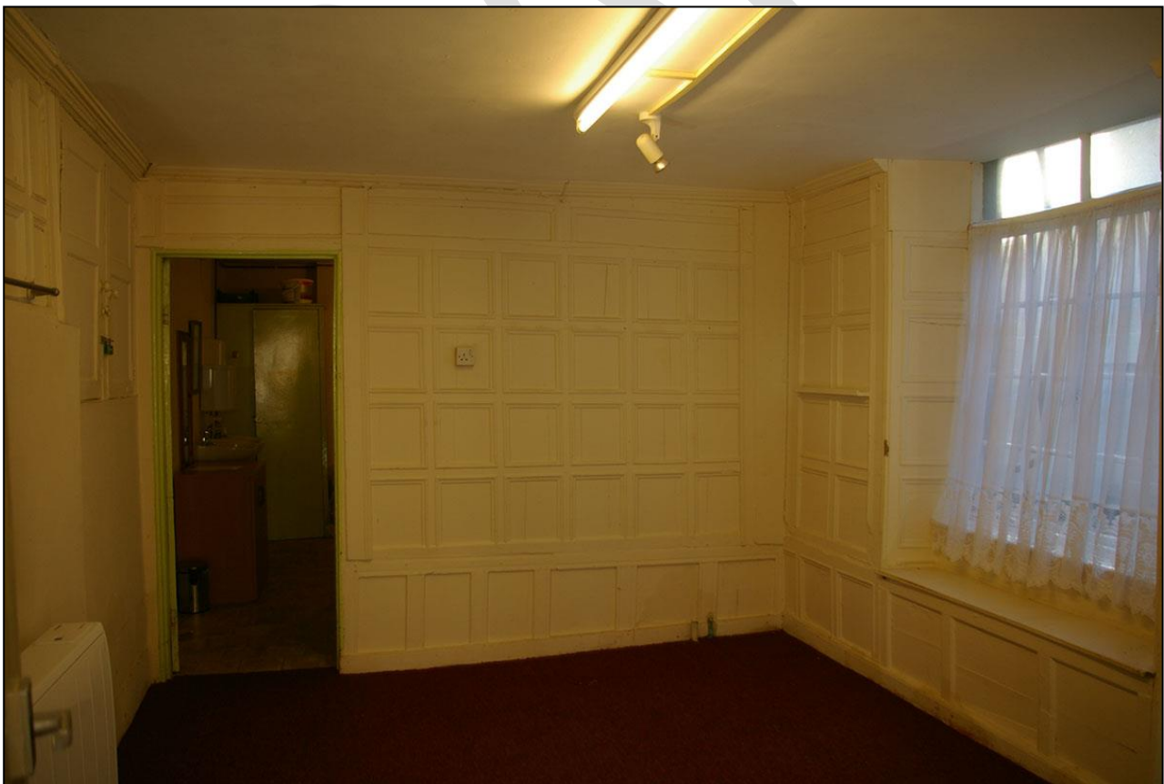
36. R17, SHOWING RESET 17 TH CENTURY PANELLING SECTIONS ON THE WALLS; FROM THE SOUTH-WEST.
