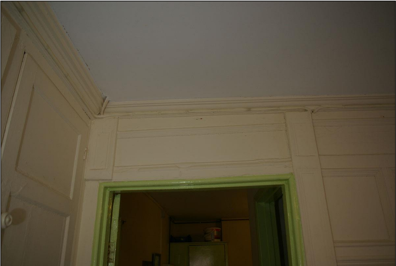
67. THE RESET PANELS ABOVE D25 ON THE NORTH WALL; FROM THE SOUTH.
