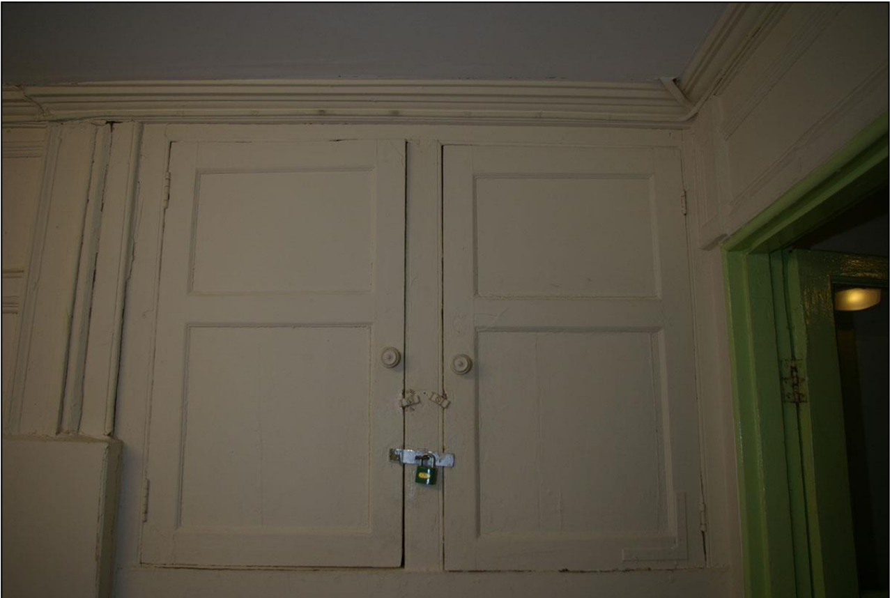
39. THE 18 TH OR EARLY 19 TH CENTURY BEADED, FLAT PANELLED CUPBOARD DOORS TO THE NORTH OF THE STACK IN R17; FROM THE EAST.
