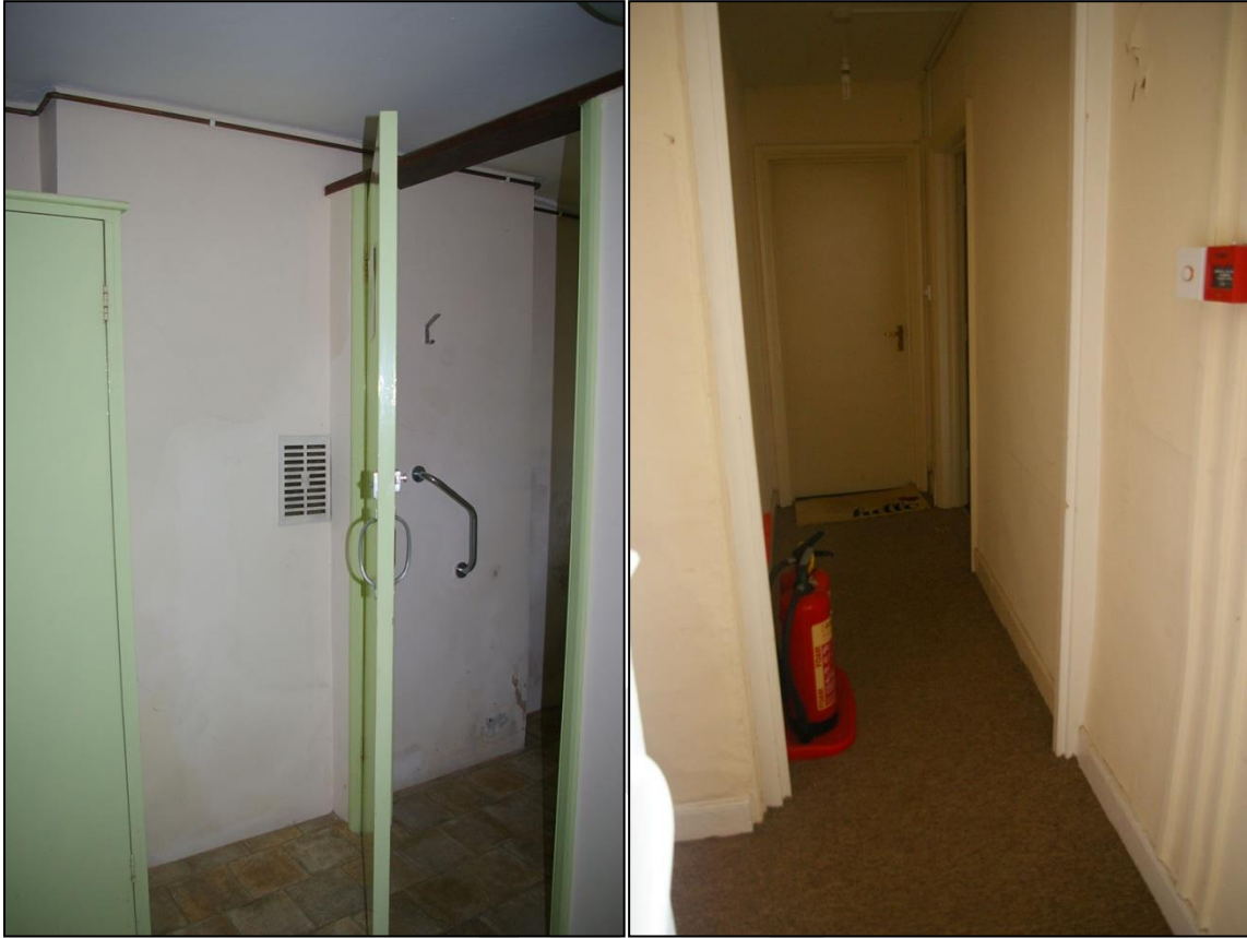
44. LEFT: AIR VENT SET INTO THE FORMER HEARTH IN THE NORTH WALL OF R19; FROM THE SOUTH-WEST.
