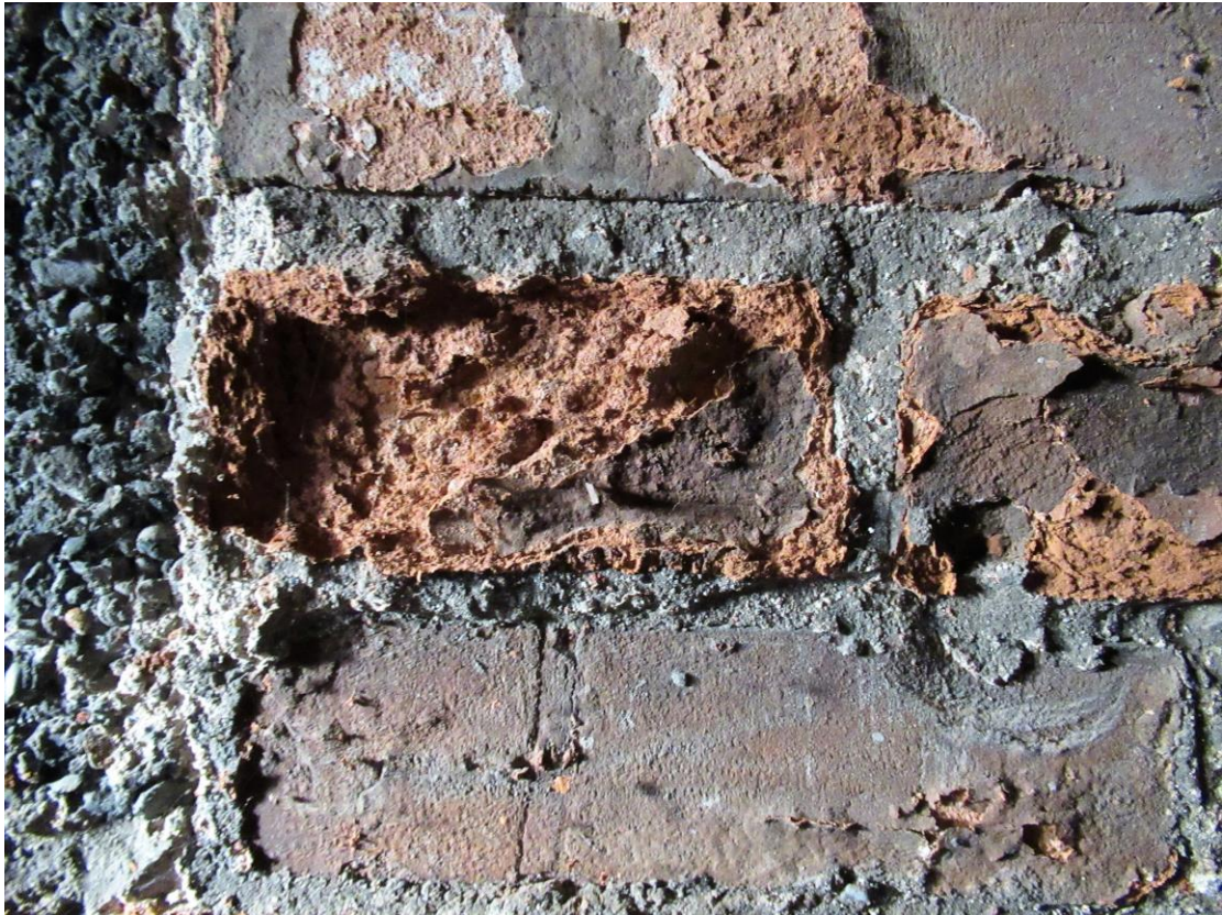
Plate 18: Spalling of brick on west wall of first floor
