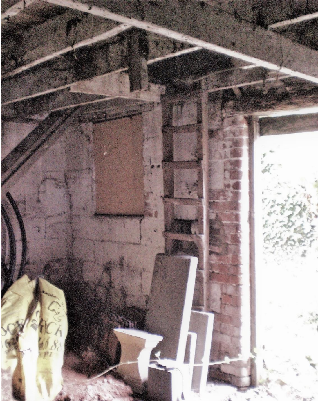
Plate 11: East wall of ground floor showing vertical ladder and brick quoins around doorway
