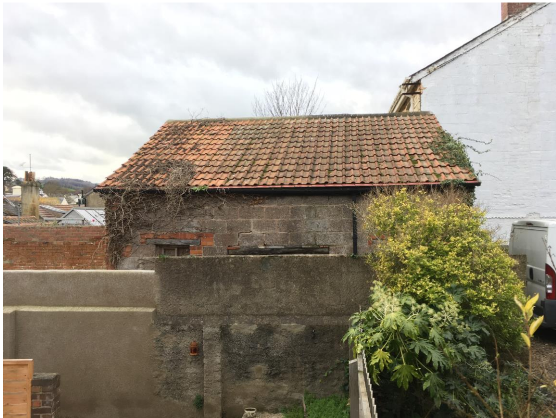
Plate 3: View of upper part of east elevation of the stable from east showing Double-Roman tile roof
