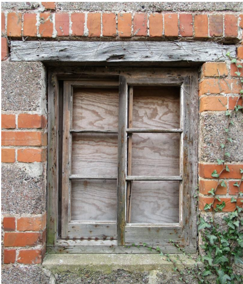
Plate 9: Timber sliding sash window in east wall with timber lintel and concrete sill. Both ground floor windows are now boarded up
