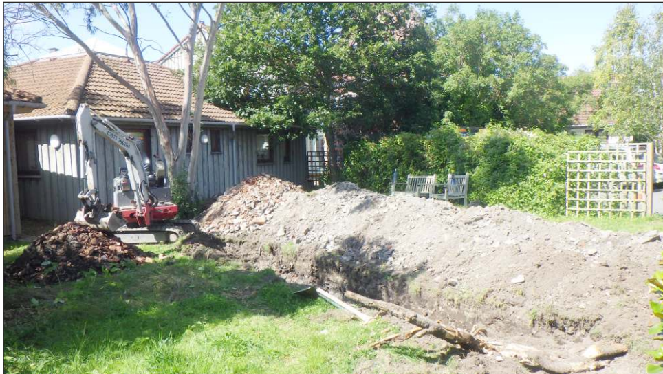
Plate 1: General view of the site with Trench 1 in the foreground, with standing kiln behind tree, looking west
