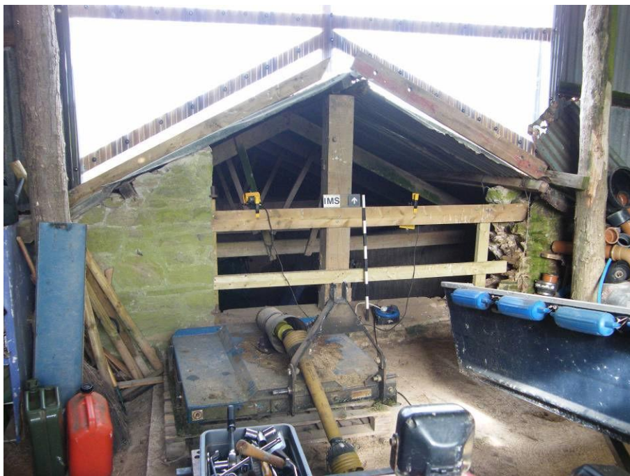
Plate 8: Southeast elevation of the threshing barn from the interior of the modern workshop
