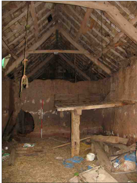
Plate 13: Partition wall to the stable and surviving loft floor in the threshing barn, looking west (2m scale)
