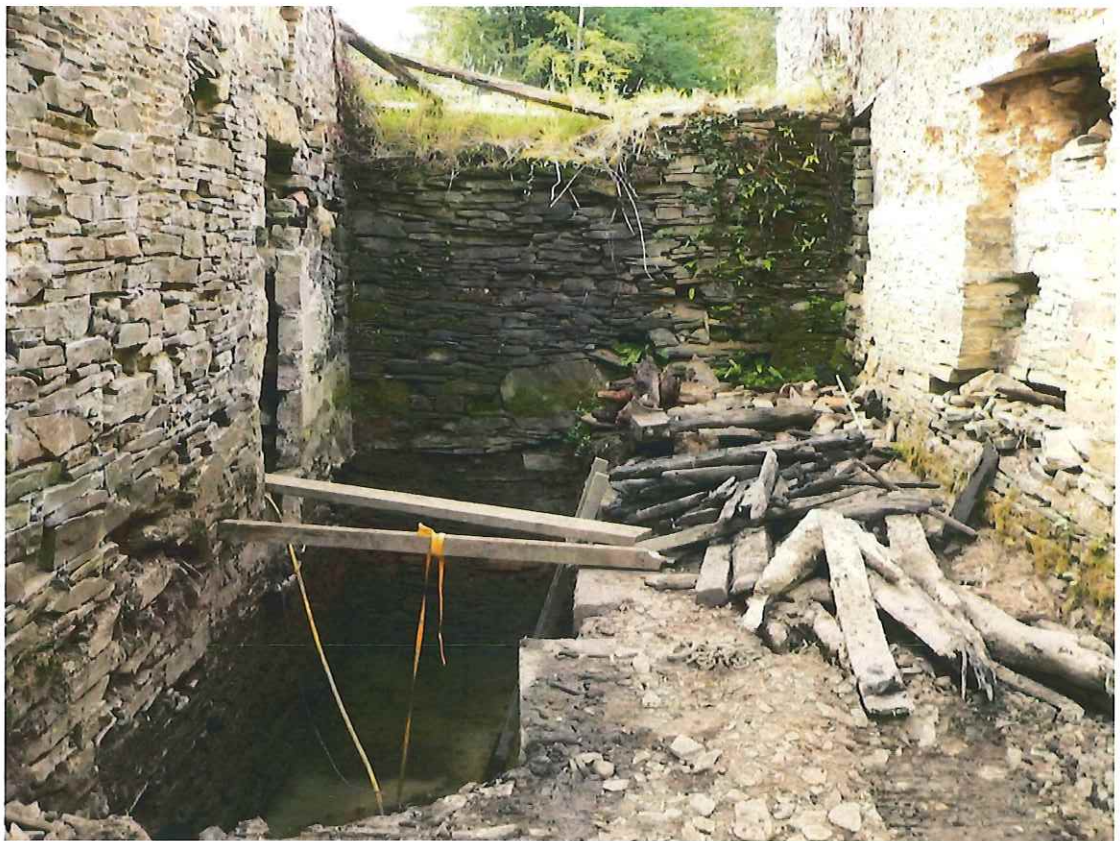
Wheelpit during excavation and clearance, with mill to left and cider barn to right. July 2011
