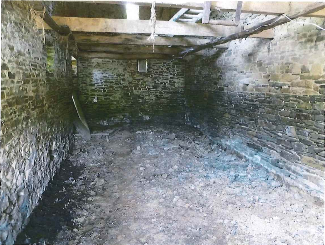
Animal house, adjoining east side of mill, after floor cobbles have been lifted. August 2011
