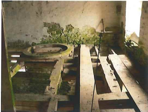
1st floor, looking south penstock control
