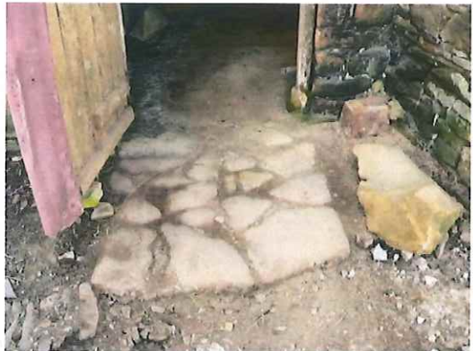
Mill door threshold
