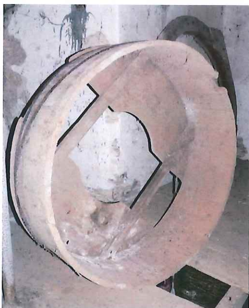
Millstone case and displaced stone skirting (behind) at 1st floor level
