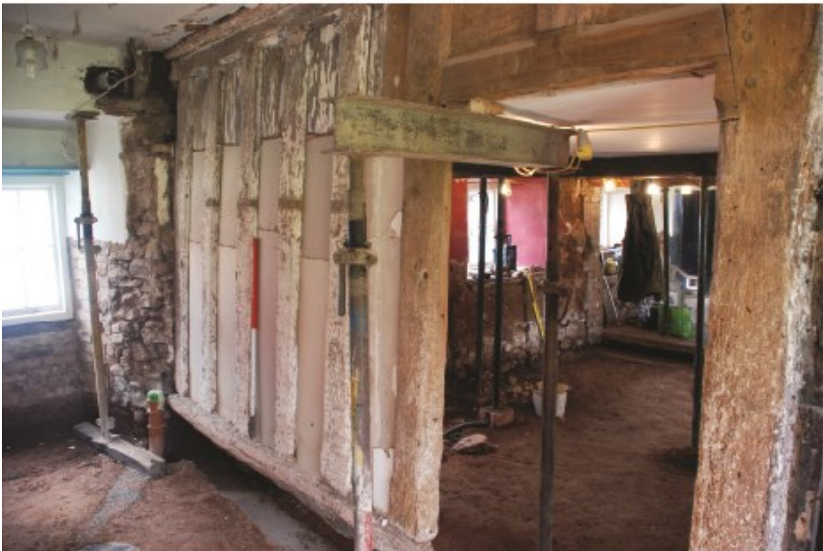
Plate 20 The screen on the lower, kitchen side of the passage, looking northeast.
