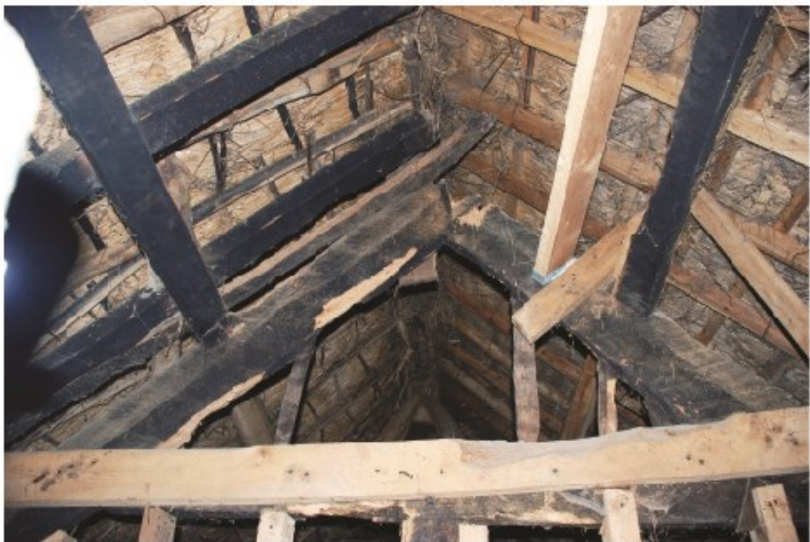
Plate 16 The early 17th-century A-frame truss supporting the east end of the medieval roof, looking east.
