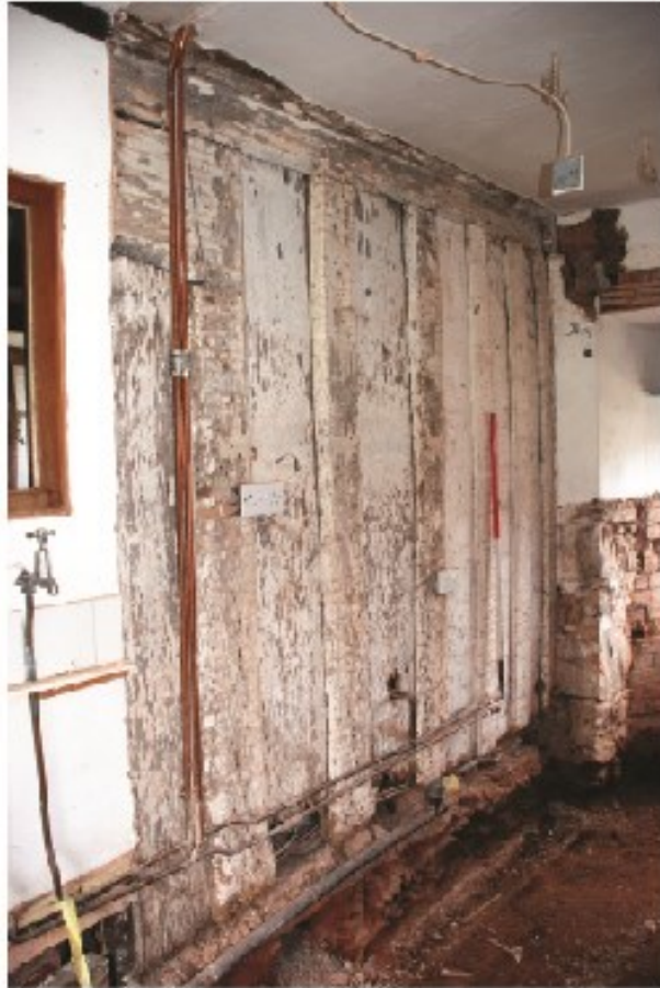
Plate 25 The screen on the hall side of the passage showing blocked Phase 4 doorway to rear, looking northwest.
