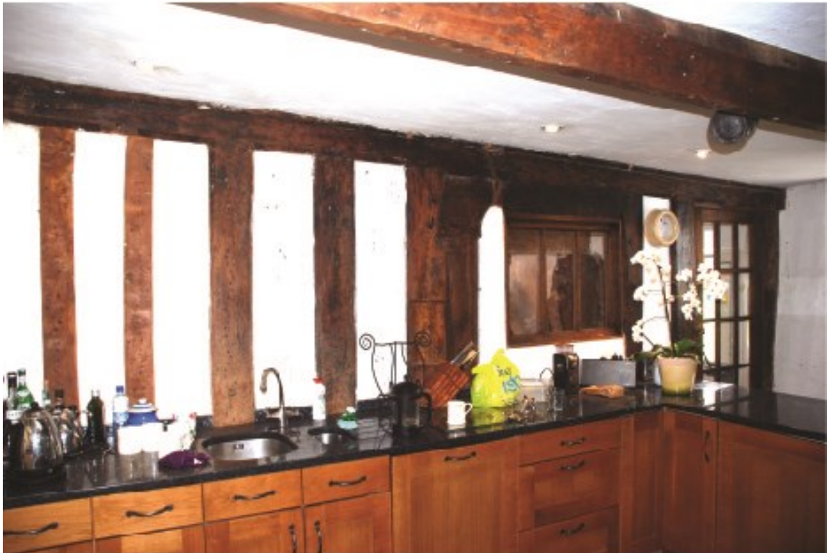
Plate 23 The screen on the hall side of the passage showing the original doorway toward the centre blocked by a later window, looking southeast.
