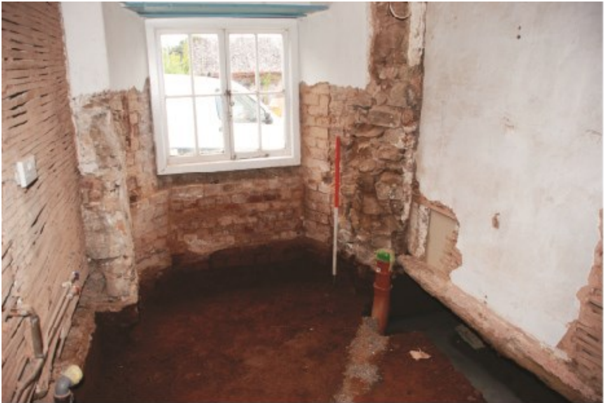
Plate 29 19th-century rubble masonry to each side of the north end of the former cross-passage, looking north.
