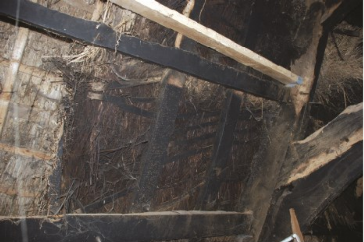
Plate 9 Smoke-blackened thatch above the former kitchen, looking southwest.
