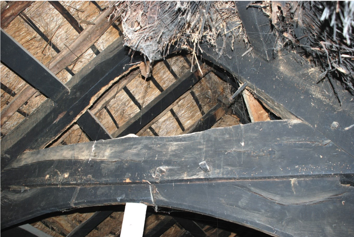
Plate 6 Arch braces beneath collar of the medieval roof, rising to separate block tenoned into the underside of the collar, looking west.
