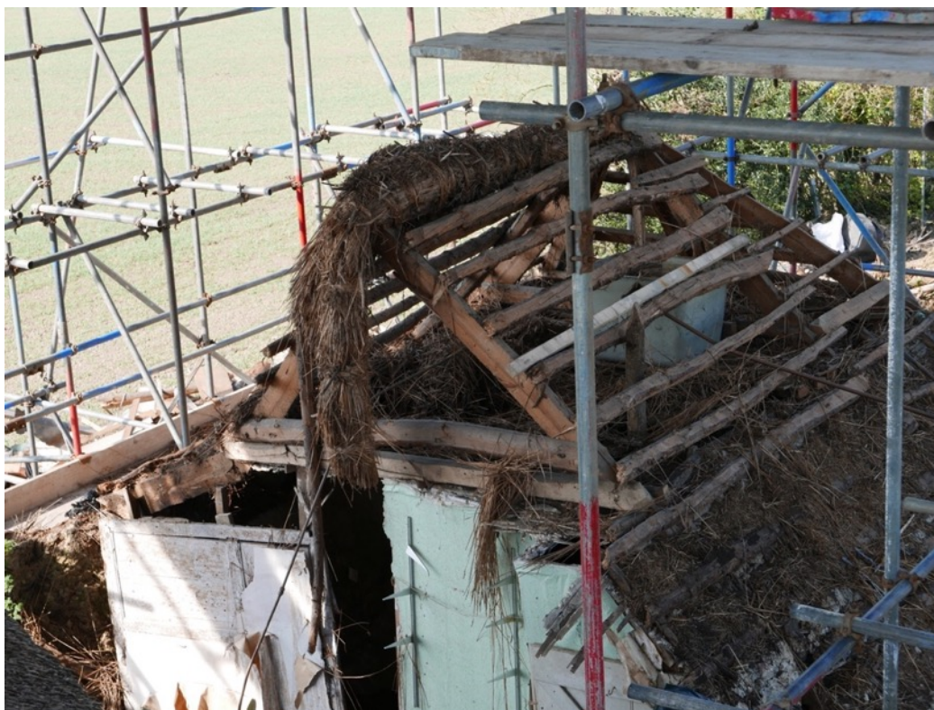
View of the western part of the roof structure of Number 2 prior to its collapse and removal. Thatch
