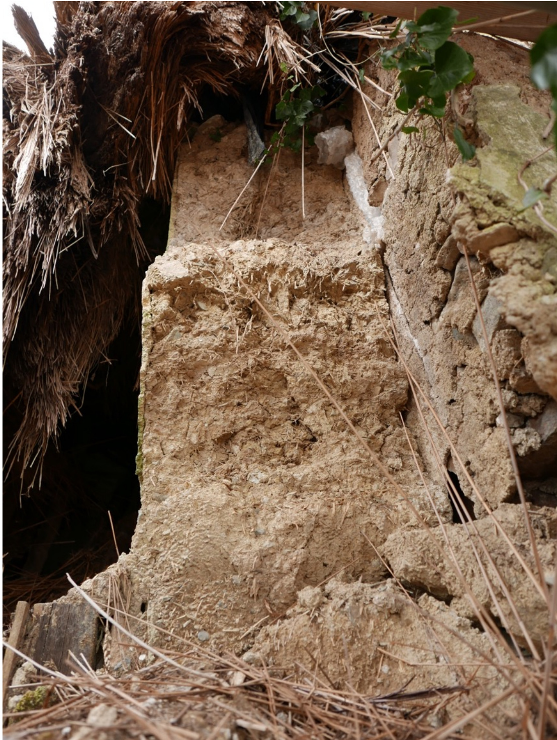
SE corner of cob wall of Number 2 in area of collapse showing how the predominantly stone rubble wall (right) of Number 1 abuts it.
