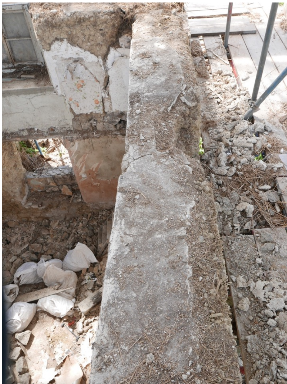
Wall top of Number 2 showing how internal plaster has been returned on to the head.
