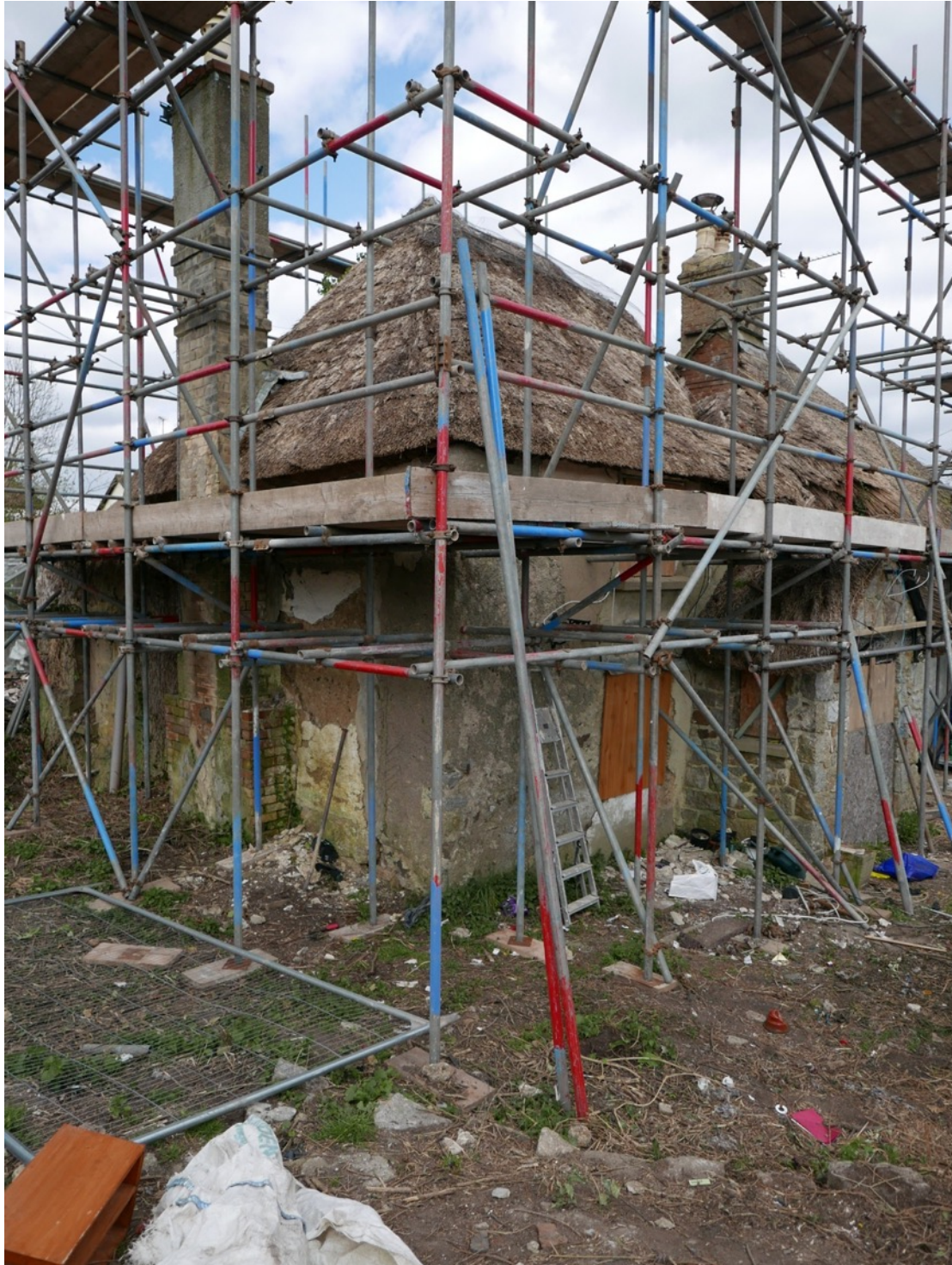
View of cottages from SW with Number 2 in the foreground (before collapse of remainder of south wall and roof).
