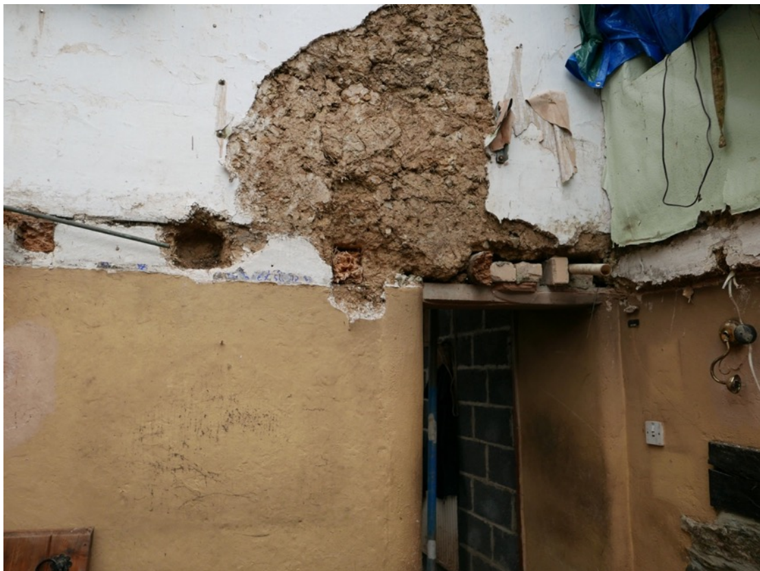
View of rotten joist ends, and sockets in north wall of Number 2
