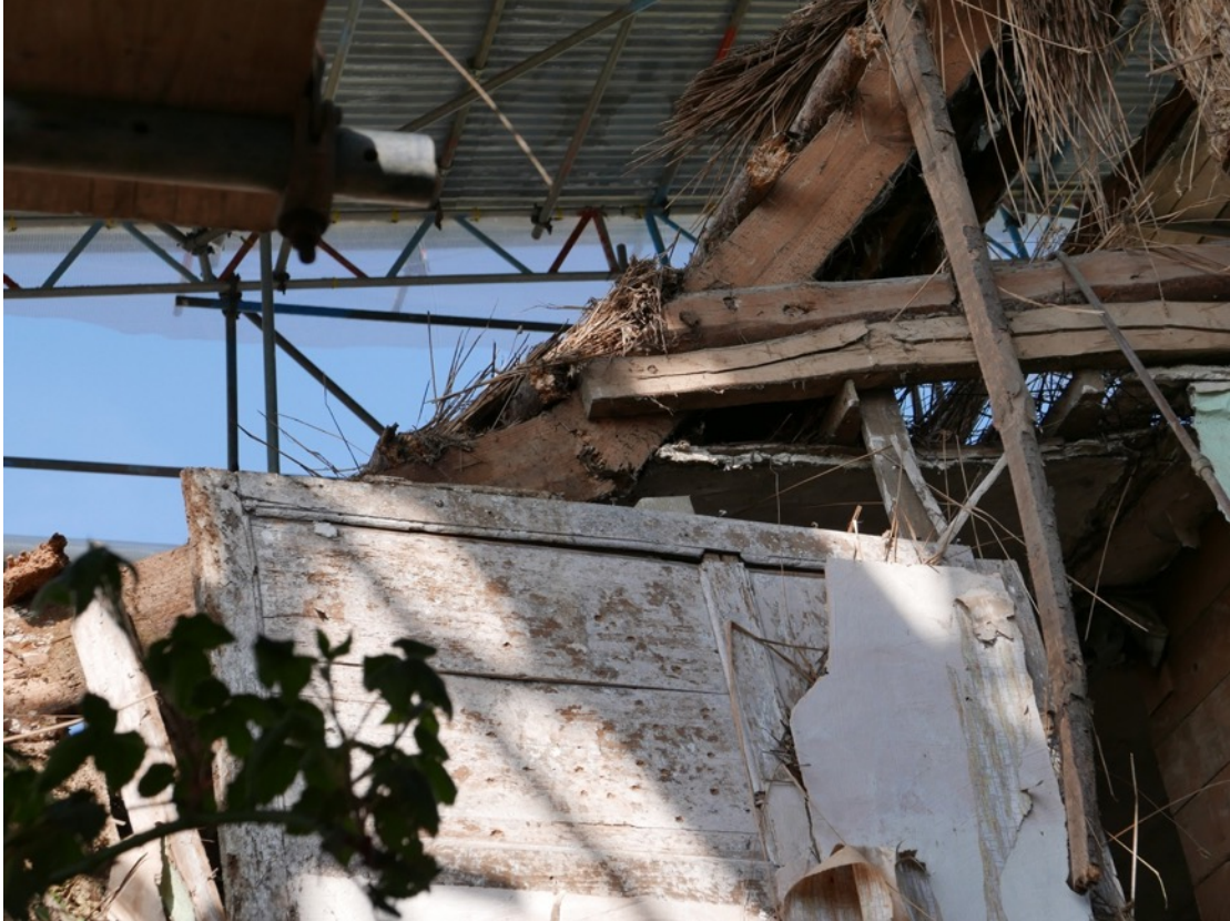
Fractured principal rafter in roof of Number 2.
