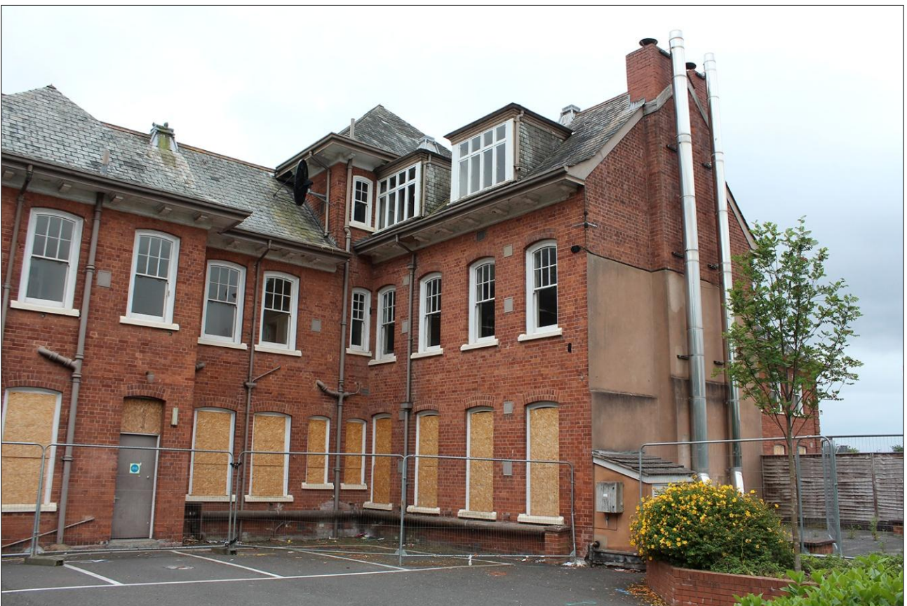
8. REAR (NORTH-EAST) EXTERNAL ELEVATION OF BUILDING, EAST END; VIEWED FROM THE NORTH-EAST.
