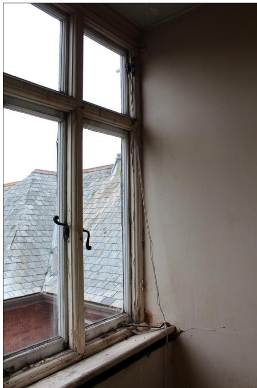
98. DETAIL OF THE WINDOW OPENING IN THE SOUTH-EAST WALL OF ROOM S7; VIEWED FROM THE NORTH.
