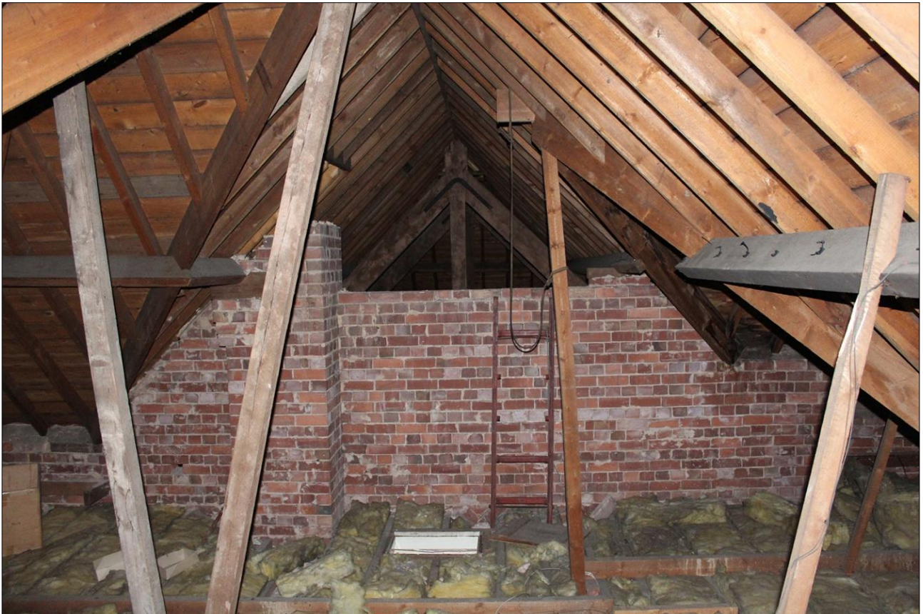
88. DETAIL OF THE ROOF STRUCTURE WITHIN ROOM S13 WITH DIVIDING BRICKWORK; VIEWED FROM THE NORTH-WEST.
