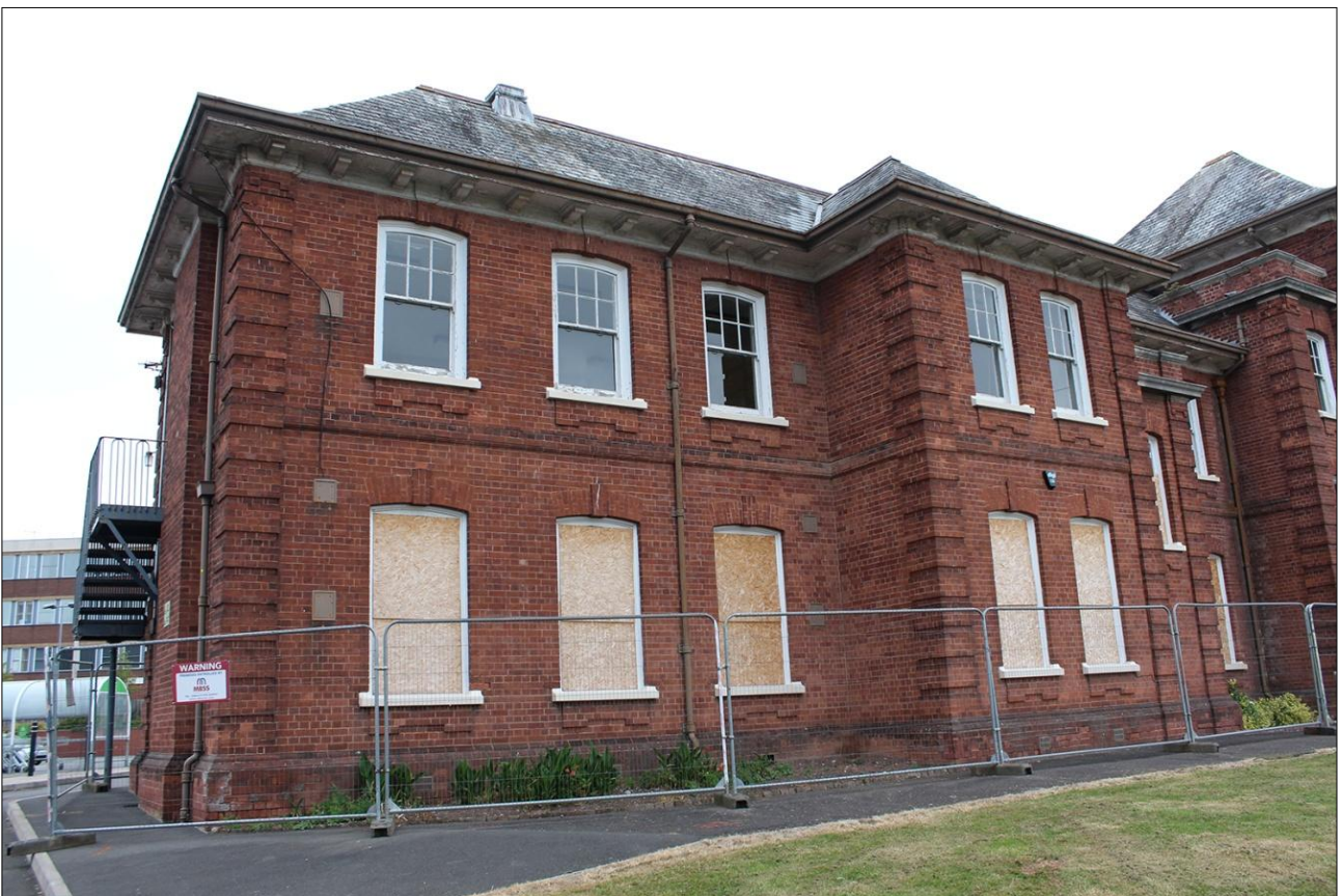
22. FRONT (SOUTH-WEST) EXTERNAL ELEVATION OF BUILDING, WEST END; VIEWED FROM THE SOUTH-WEST.
