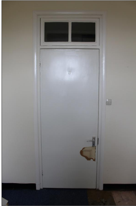
59. VIEW OF THE DOOR IN THE NORTH-EAST WALL OF ROOM F13, SHOWING IT TO BE AN ORIGINAL 1913 PANELLED DOOR; VIEWED FROM THE SOUTH-WEST.
