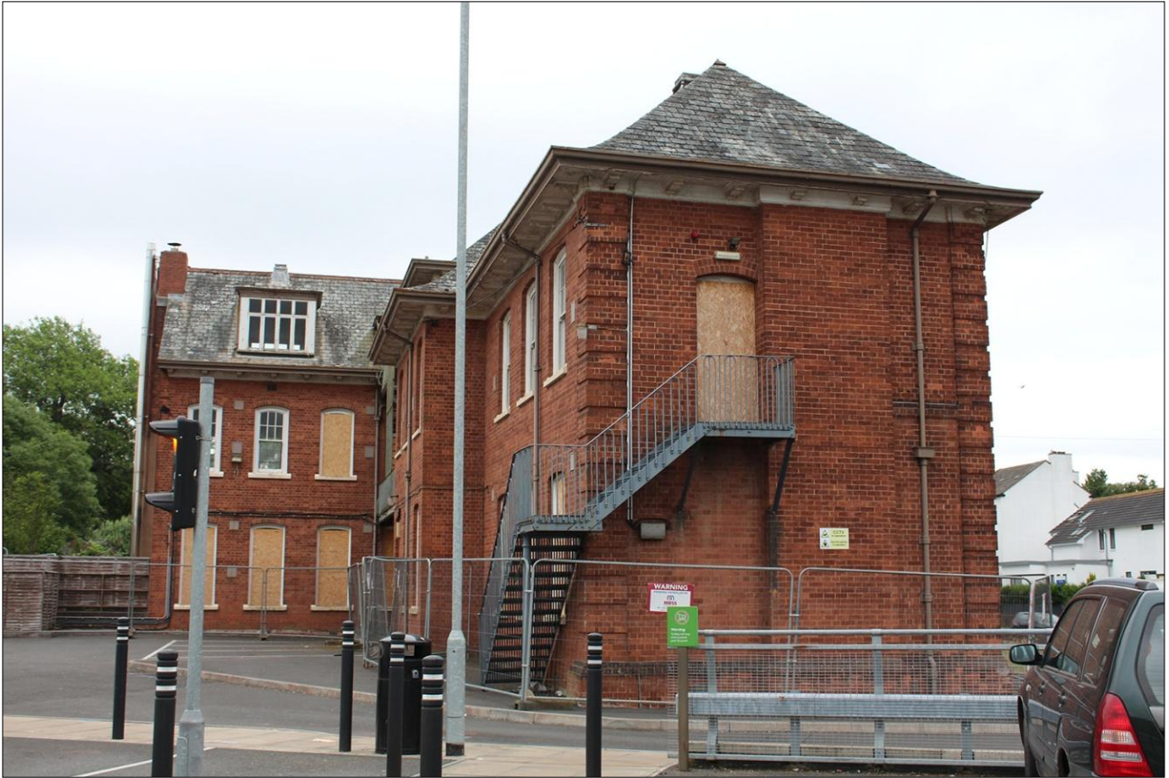
19. REAR (NORTH-EAST) AND NORTH-WEST EXTERNAL ELEVATIONS OF BUILDING; VIEWED FROM THE NORTH-WEST.
