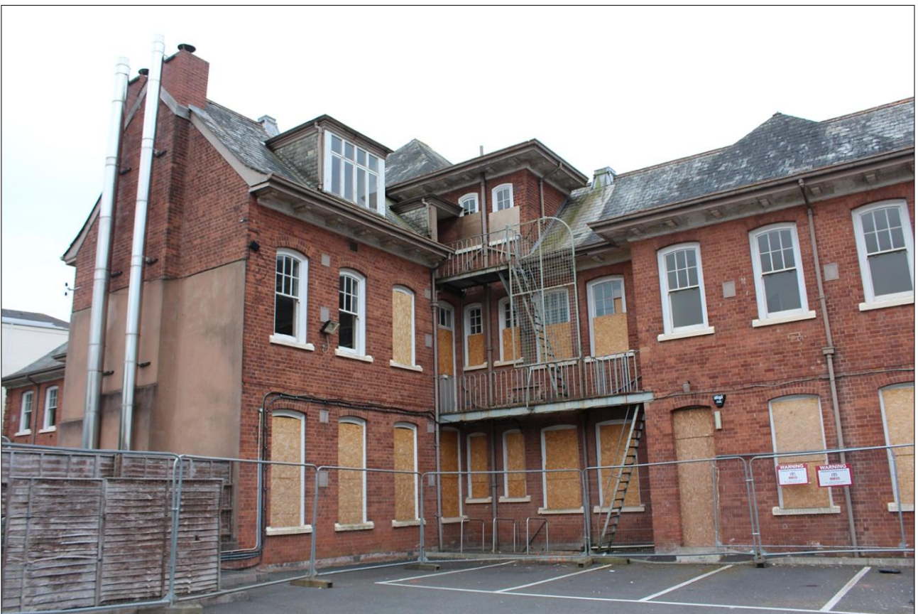
14. REAR (NORTH-EAST) EXTERNAL ELEVATION OF BUILDING, WEST END; VIEWED FROM THE NORTH-WEST.
