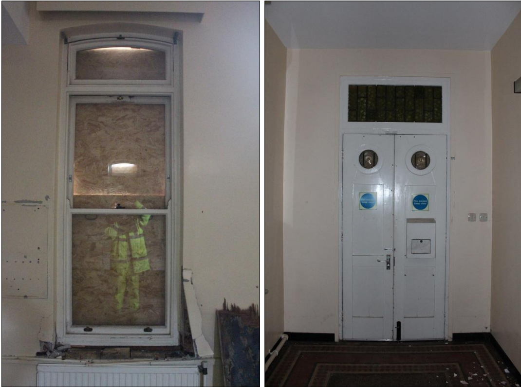
LEFT: 40. DETAIL OF WINDOW OPENING IN NORTH-WEST WALL, ROOM 20; VIEWED FROM THE SOUTH-EAST. RIGHT: 41. DETAIL OF THE FRONT DOOR, ROOM 22; VIEWED FROM THE NORTH-EAST.
