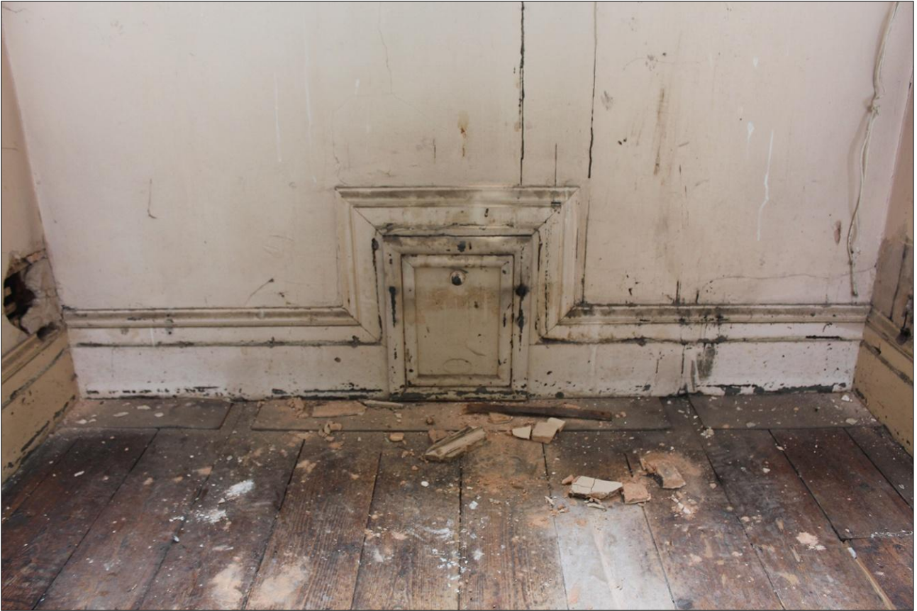
99. DETAIL OF THE VENT OPENING IN THE SOUTH-EAST WALL OF ROOM S7; VIEWED FROM THE NORTH-WEST.
