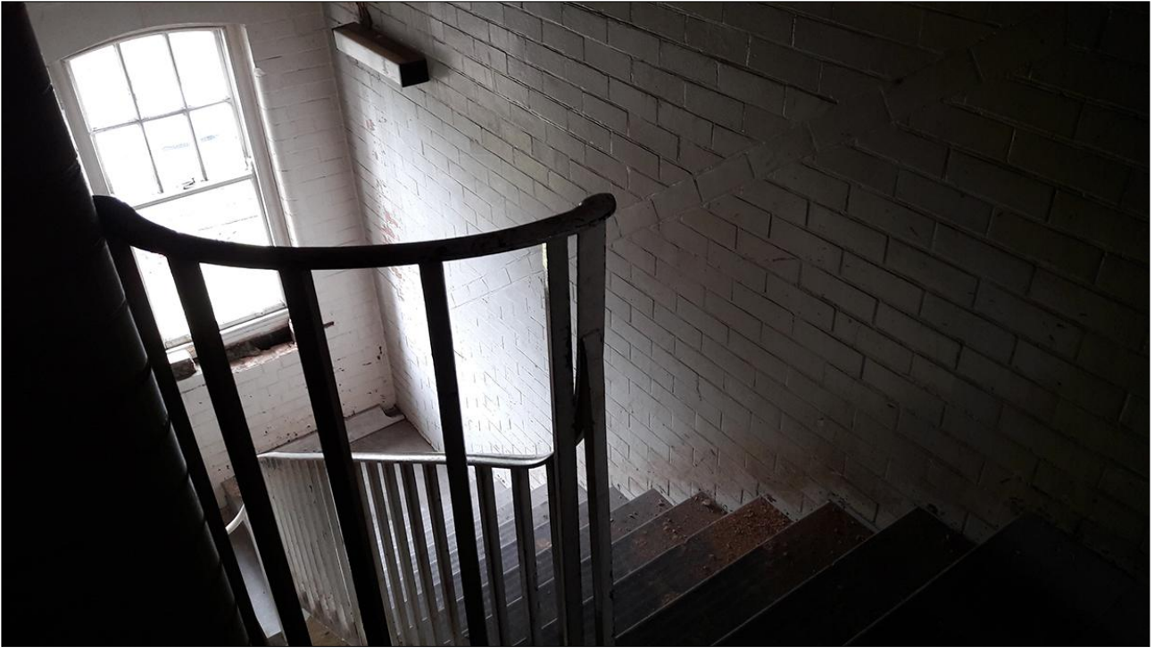
74. DETAIL OF STAIRWELL G7 FROM SECOND FLOOR LANDING; VIEWED FROM THE NORTH-EAST.
