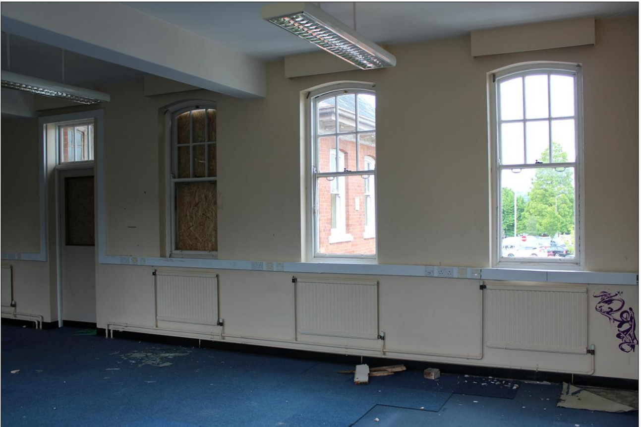
65. DETAIL OF ROOM F12 SHOWING WINDOW OPENINGS IN THE NORTH-EAST WALL; VIEWED FROM THE SOUTH-EAST.
