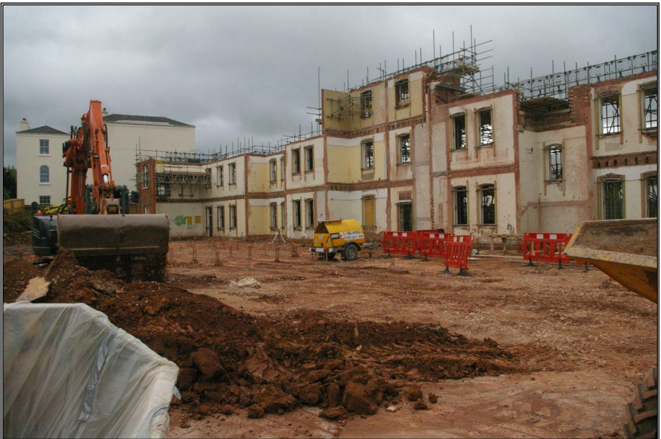
21. VIEW OF THE REAR OF THE BUILDING AFTER DEMOLITION; VIEWED FROM THE NORTH-WEST (NO SCALE).
