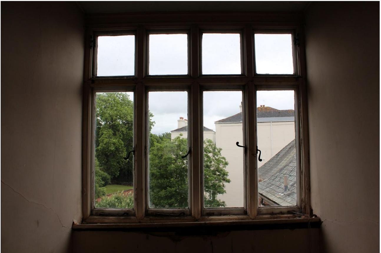
97. DETAIL OF THE WINDOW OPENING IN THE SOUTH-EAST WALL OF ROOM S7; VIEWED FROM THE NORTH-WEST.
