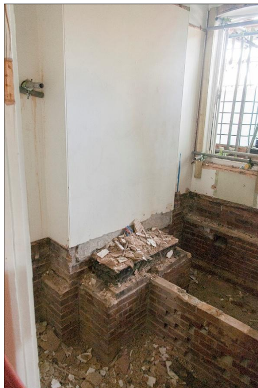
107. ROOM G4, SHOWING THE UNDER-FLOOR CAVITY AND THE BASE OF THE HEARTH; VIEWED FROM THE NORTH.
