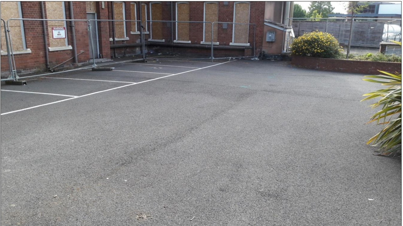
2. CAR PARK AREA TO REAR (NORTH) OF BUILDING, EAST END; VIEWED FROM THE EAST (NO SCALE).
