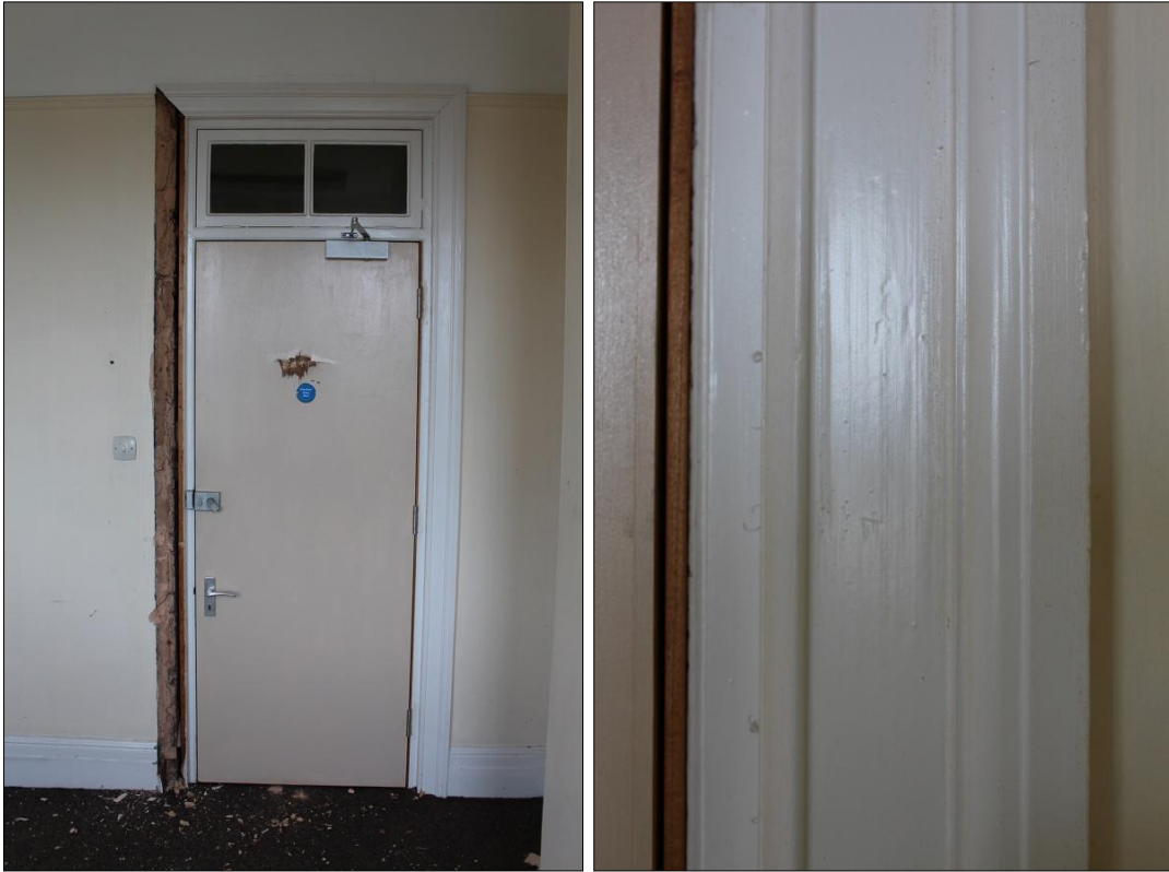
LEFT: 51. DETAIL OF DOOR IN NORTH-EAST WALL, ROOM F4; VIEWED FROM THE SOUTH-WEST.
