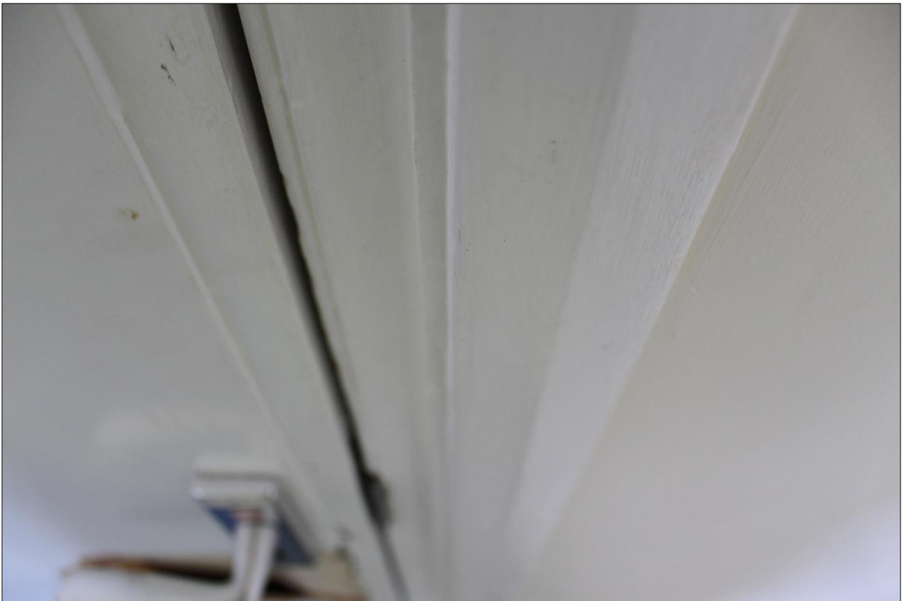
60. DETAIL OF THE MOULDINGS ON THE DOOR FRAME IN THE NORTH-EAST WALL, ROOM F13; VIEWED FROM THE SOUTH-WEST.
