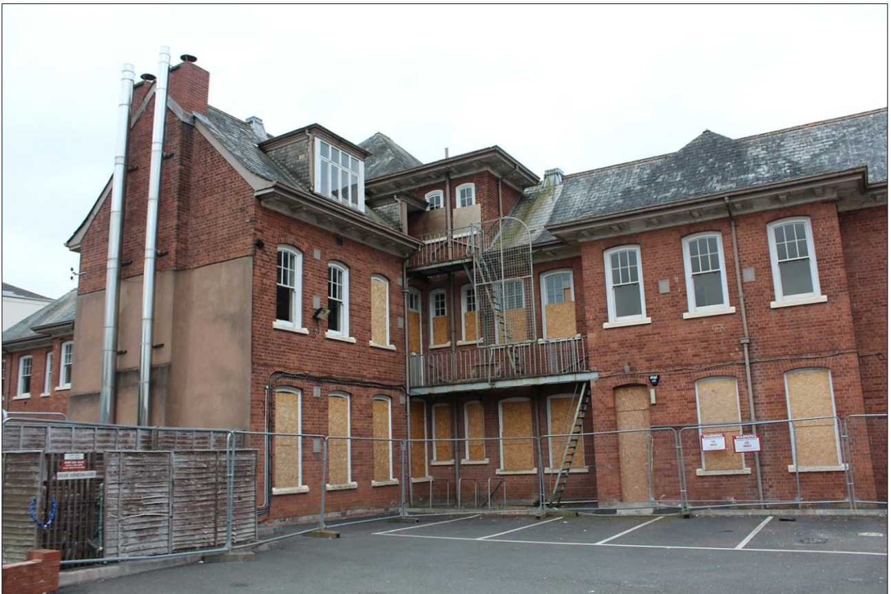
16. REAR (NORTH-EAST) EXTERNAL ELEVATION OF BUILDING, WEST END; VIEWED FROM THE NORTH-WEST.
