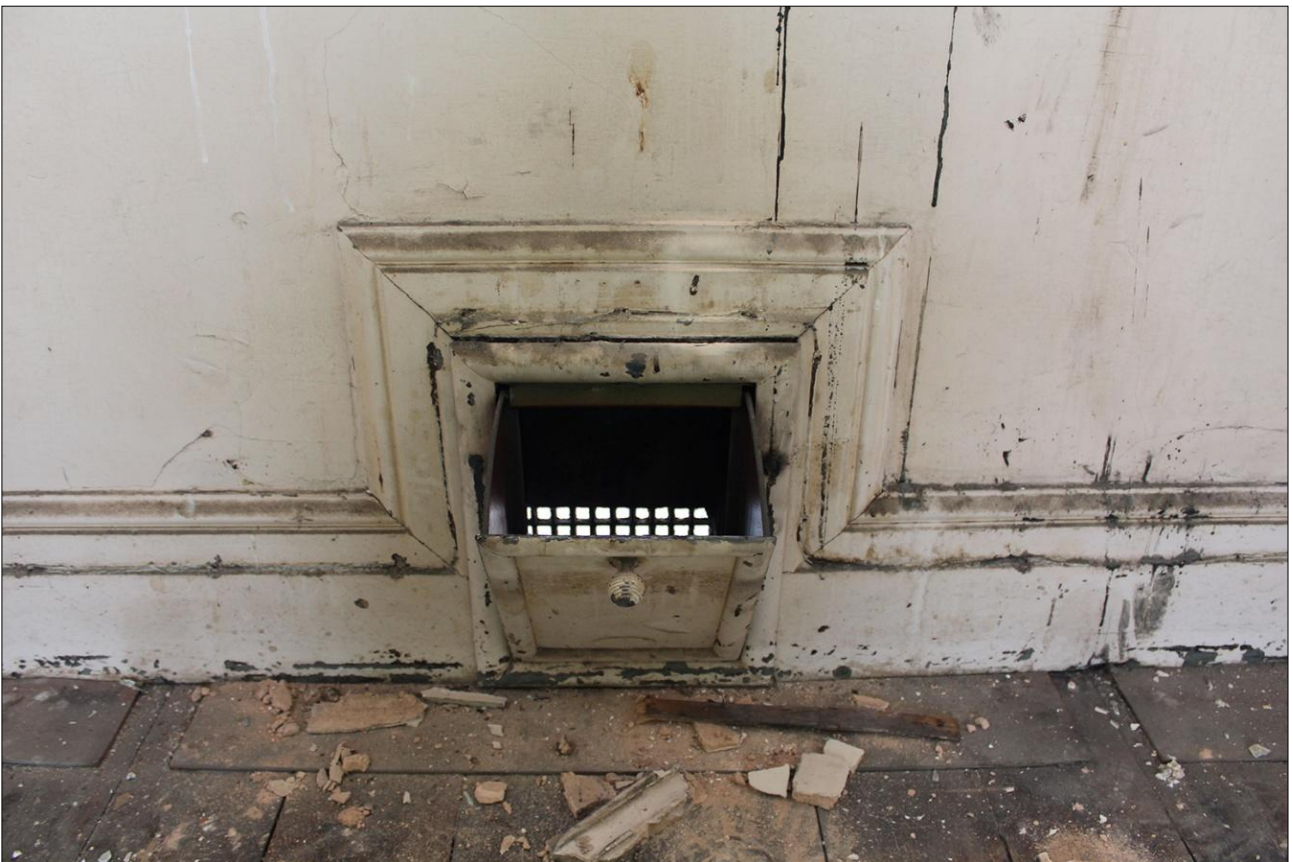
100. DETAIL OF THE VENT OPENING IN THE SOUTH-EAST WALL OF ROOM S7; VIEWED FROM THE NORTH-WEST.
