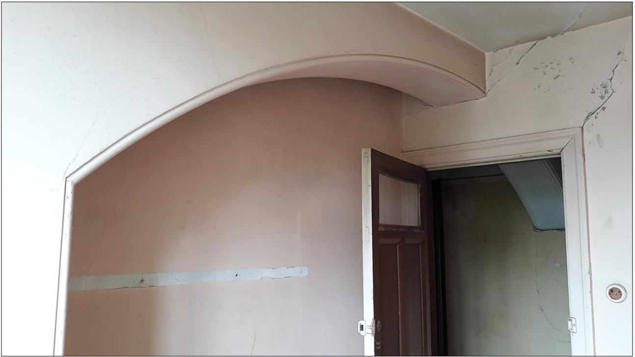
92. VIEW DETAILING THE INSERTED WALLS DIVIDING ROOMS S8, S9, S10, FROM WITHIN ROOM S9; VIEWED FROM THE NORTH-EAST.
