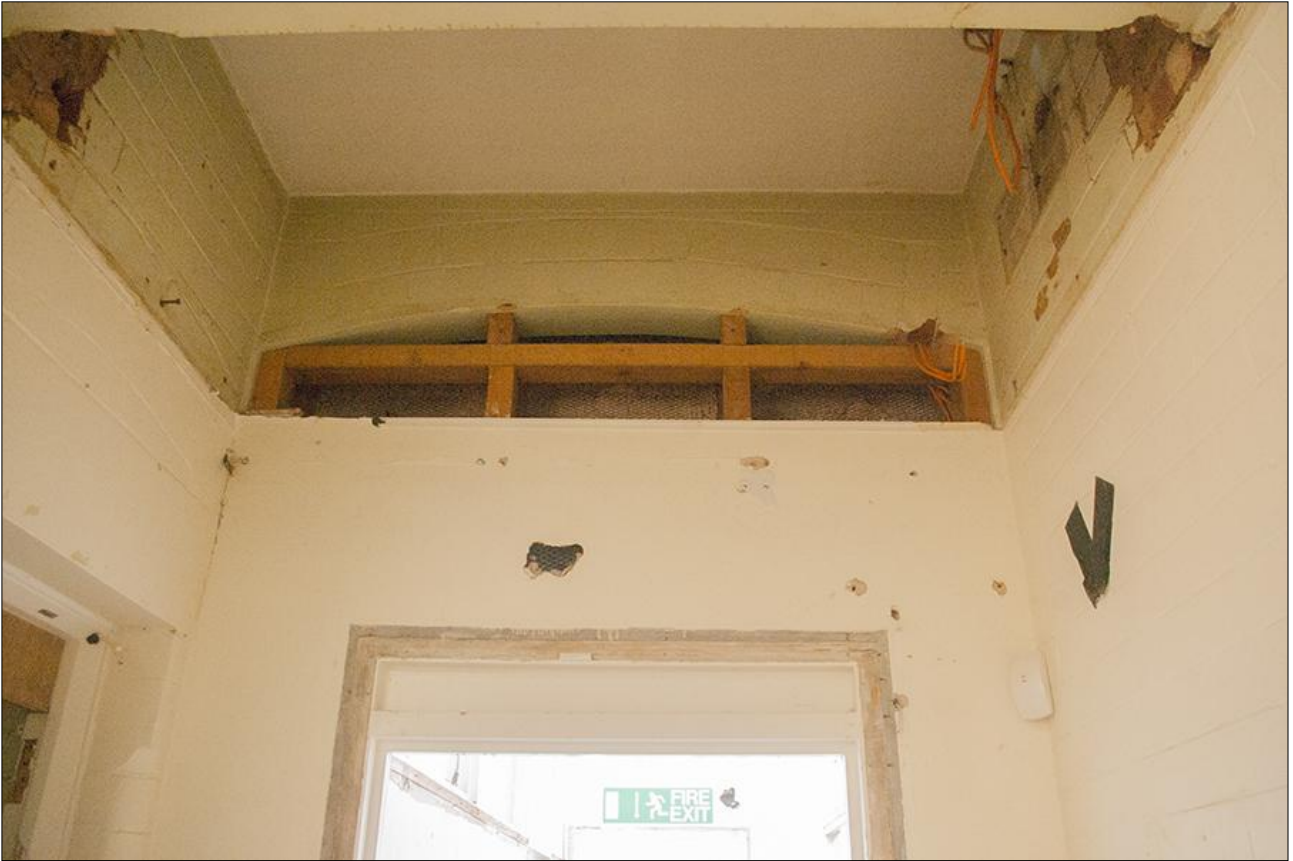
108. THE PARTITION WALL WITH DOOR BETWEEN ROOM G3 AND ROOM G6, SHOWING THE ORIGINAL HEIGHT OF THE OPENING; VIEWED FROM THE NORTH-WEST.
