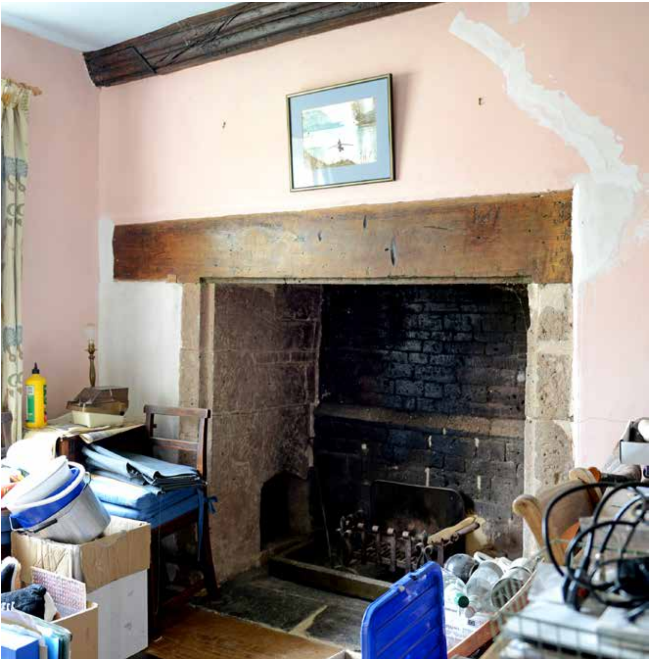
21. The chamber fireplace from the southeast showing the doorway to the fire-box in the western cheek.
