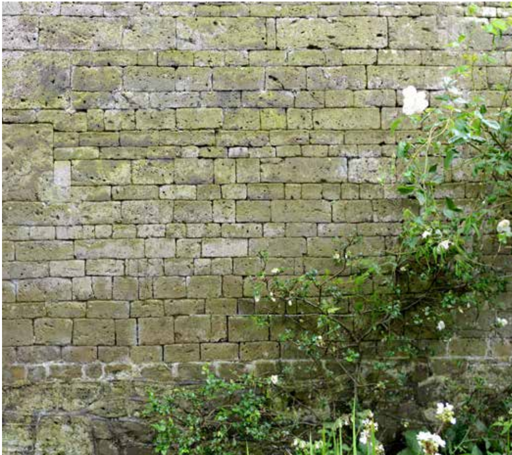
5. Detail of the volcanic ashlar masonry on the north wall - there is no plinth on this side.
