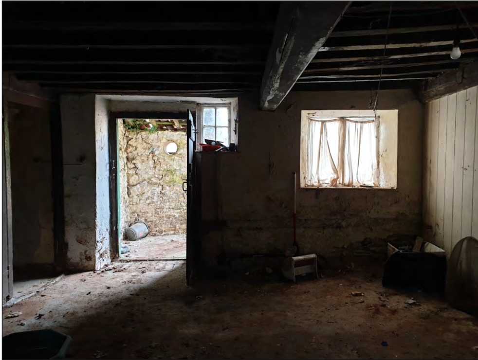
Pl. 9 General view of west elevation in G02 showing 18th century doorway and window arrangement with original joists resting on top of, rather than within the replacement beam. 1m scale. Looking west.
