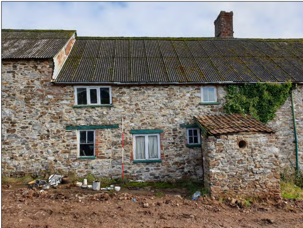
Pl. 6 General view of north end showing ground- and first-floor fenestration and blocked doorway. 2m scale. Looking east.
