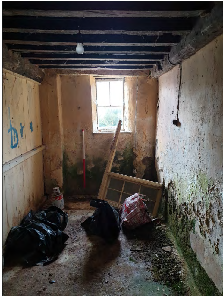
Pl. 14 General view of former corridor G03 showing blocked doorway. 1m scale. Looking west.
