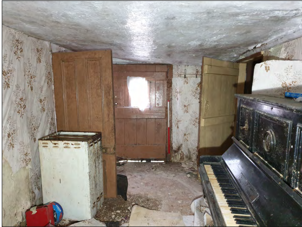
Pl. 21 General view of former cross-passage G05 defined by cob-and-stud partitions with 19th century doorways leading to G04 and G06 respectively. The additional width on the south side suggests the position of a former stair. 1m scale. Looking east.
