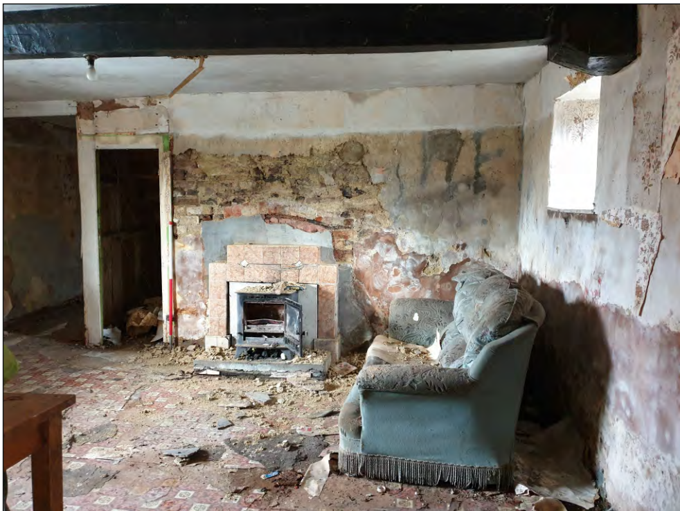
Pl. 16 General view of north elevation in G04 showing inserted fireplace with later 19th century rebuilding and modern infilling. 1m scale. Looking north.
