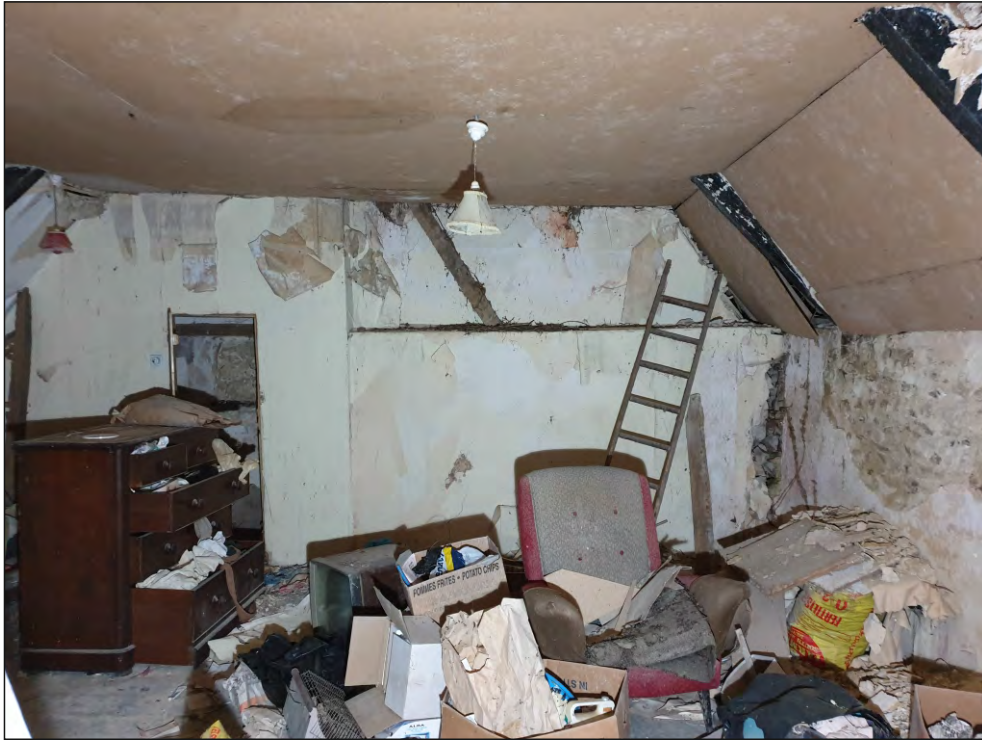
Pl. 29 General view of south elevation in F01 showing chimney stack with the cupboard to the left with its blocked window the possible position of a former staircase. The roof over the southern end has been replaced in the 19th century. Looking south.
