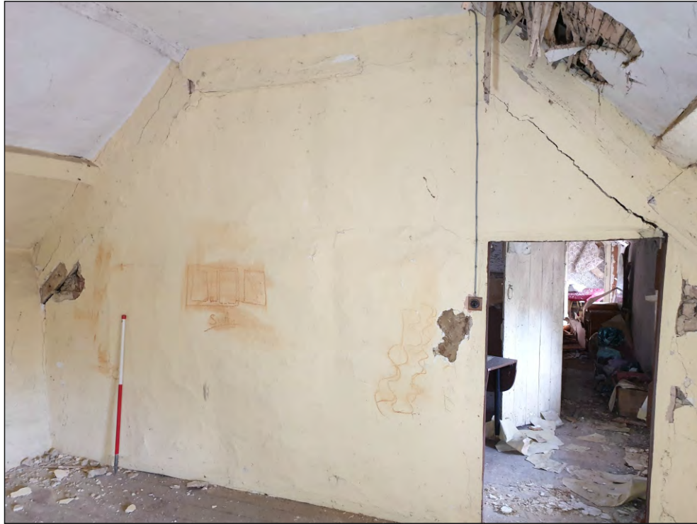
Pl. 33 General view of south elevation in F05 showing the cob-and-stud partition with later doorway. 1m scale. Looking south.
