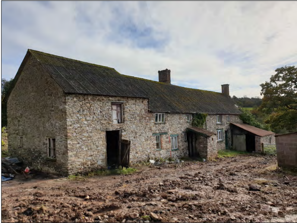
Pl. 3 General view of the farmyard elevation showing the barn at the northern end of the main range. 2m scale. Looking southeast.
