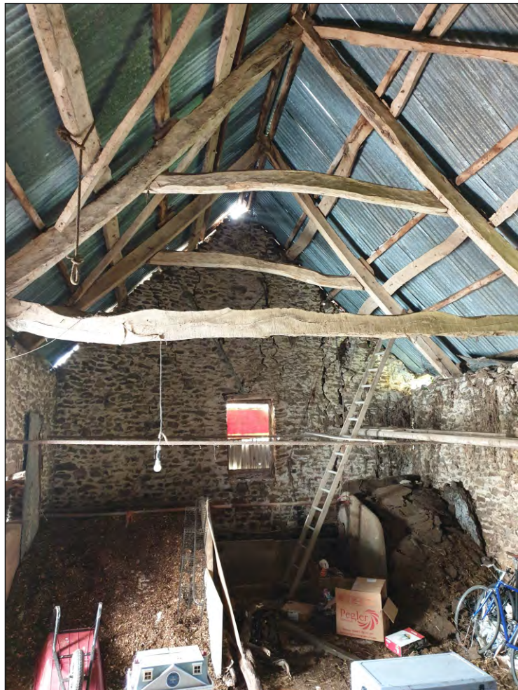
Pl. 44 General view of south elevation of former threshing barn showing roof construction. Looking south.
