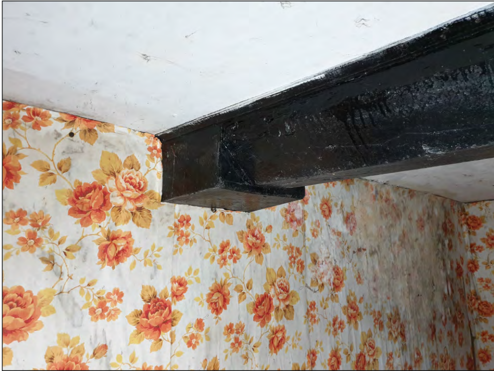
Pl. 25 Close-up showing the projecting bracket supporting the west end of the 17th century beam in G06. Looking northwest.
