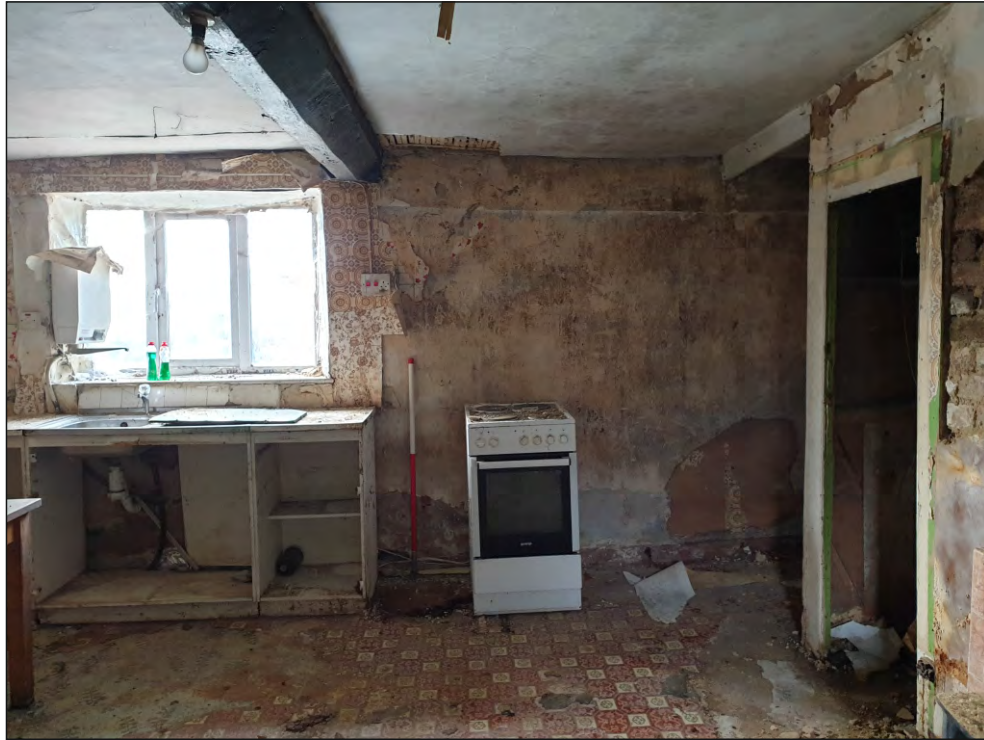
Pl. 19 General view of west elevation in G04 showing modern uPVC window and 17th century beam. 1m scale. Looking west.
