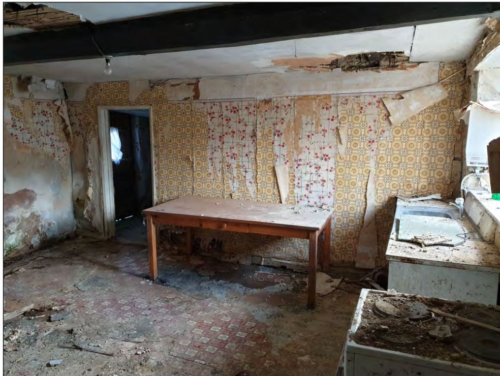
Pl. 20 General view of south elevation in G04 showing 19th century doorway. The beam above the cob-and-stud partition has seemingly been removed with the ceiling joists simply resting on top of the partition. Looking south.
