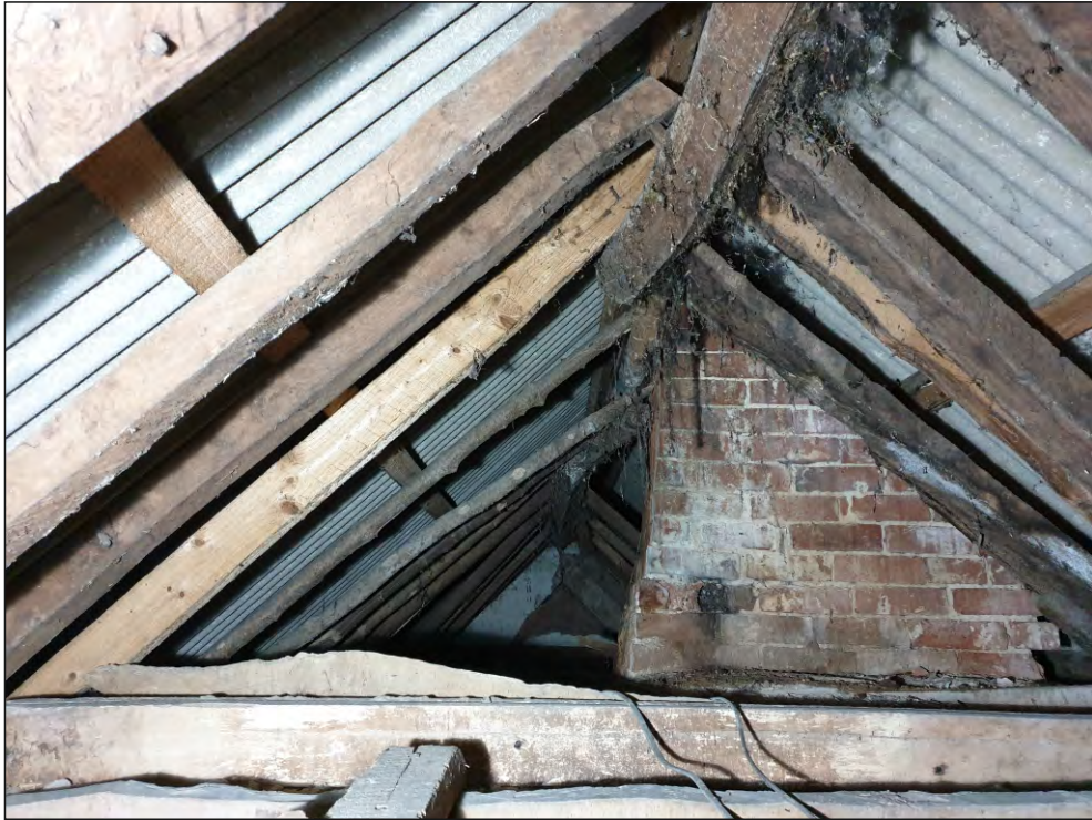
Pl. 35 General view of roof structure showing original section above F03, F04 and F05 truncated by insertion of chimney stack. Looking north.
