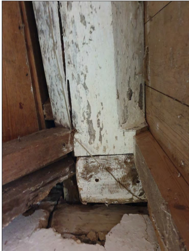
Pl. 26 Close-up showing the projecting bracket supporting the east end of the 17th century beam in G06. Looking east.
