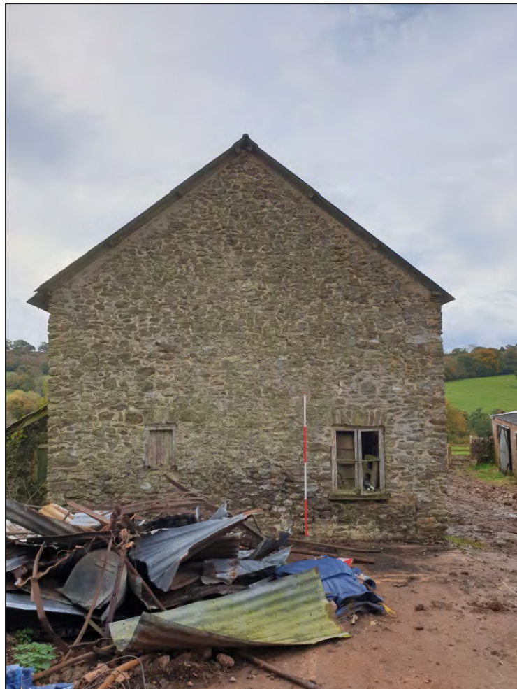
Pl. 8 Close-up of north elevation of barn showing blocked doorway. 2m scale. Looking south.
