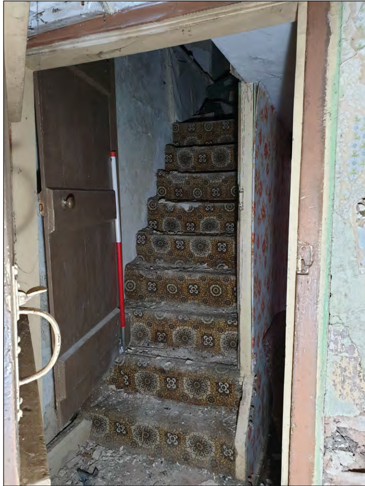
Pl. 23 Close-up of stair within G06 leading to F01. 1m scale. Looking southeast.
