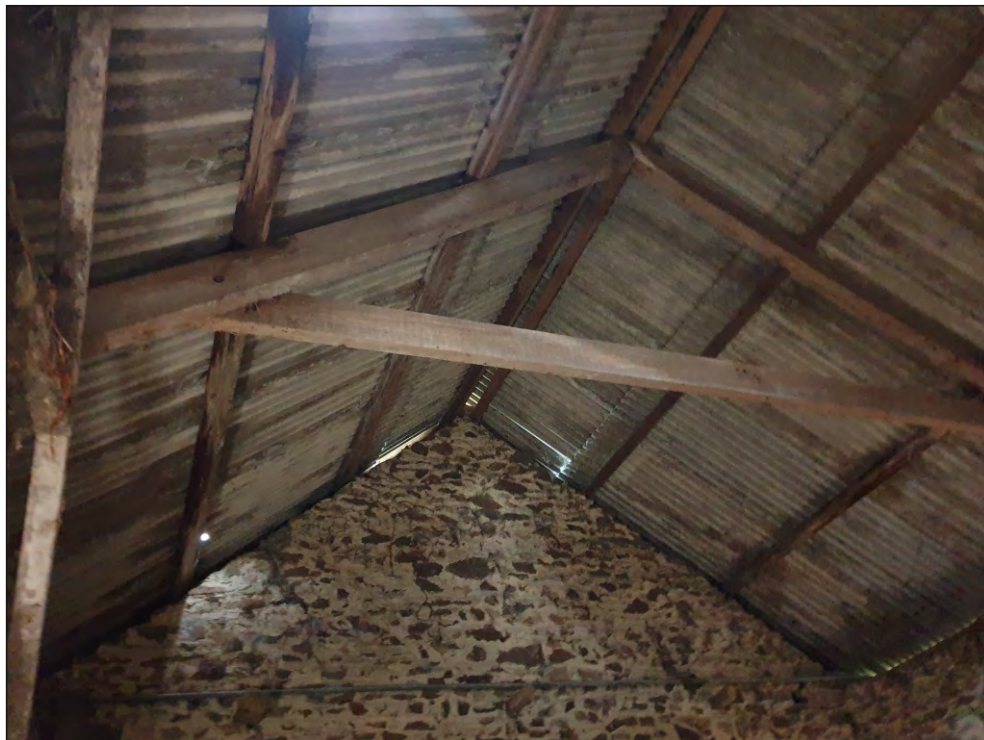
Pl. 40 General view of roof structure showing late 19th or early 20th century A-frame with applied collar. Looking north.
