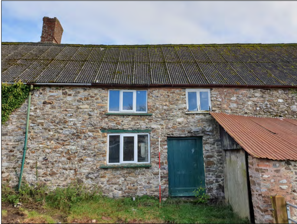
Pl. 5 Close-up of south end showing ground- and first-floor fenestration and position of cross-passage with 17th century doorway. 2m scale. Looking east.
