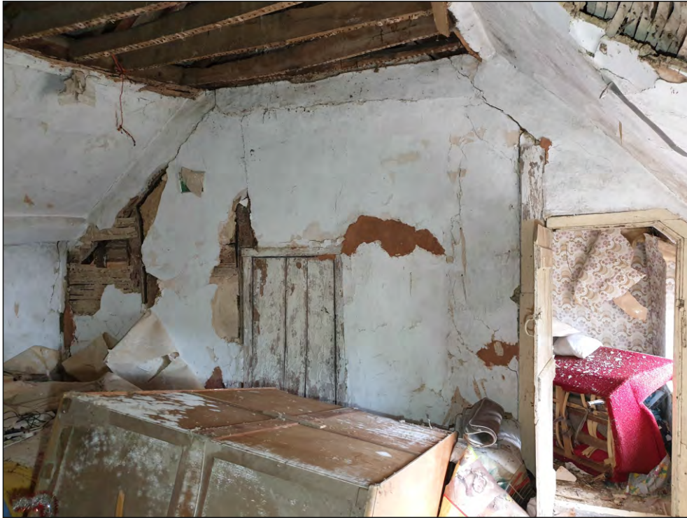
Pl. 31 General view of south elevation in F03 showing original 17th century low doorway in the centre of the cob-and-stud partition with later 19th century doorway inserted to the right. Looking south.
