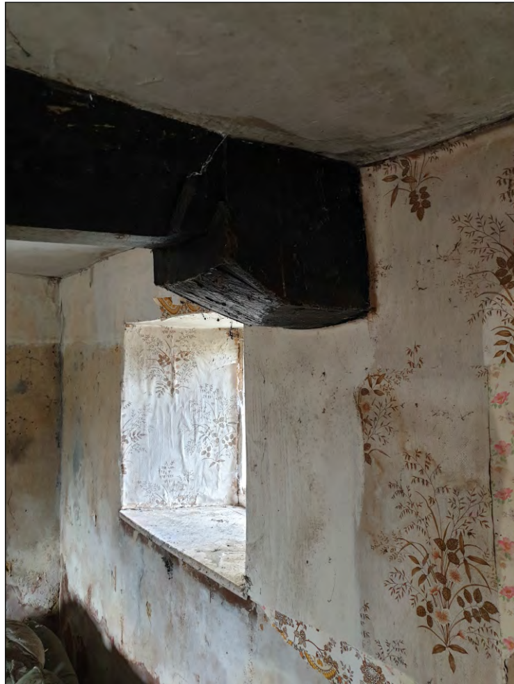
Pl. 18 Close-up showing the projecting bracket supporting the 17th century beam. Looking northeast.
