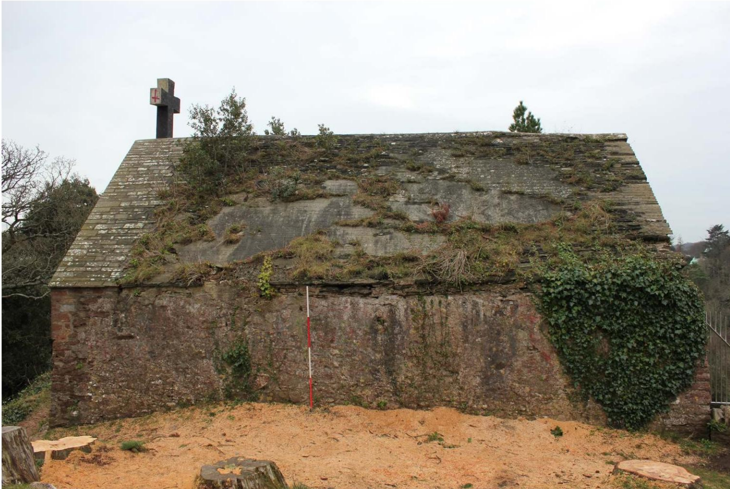
Fig. 3: St Michael's Chapel in 2015 prior to conservation works. Viewed from the north. (2m scale)
