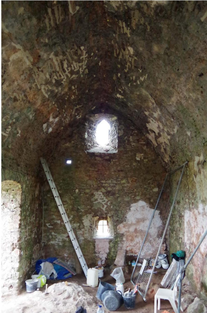
Fig. 14: St Michael's Chapel, interior during conservation works, showing vaulted roof and west end.
