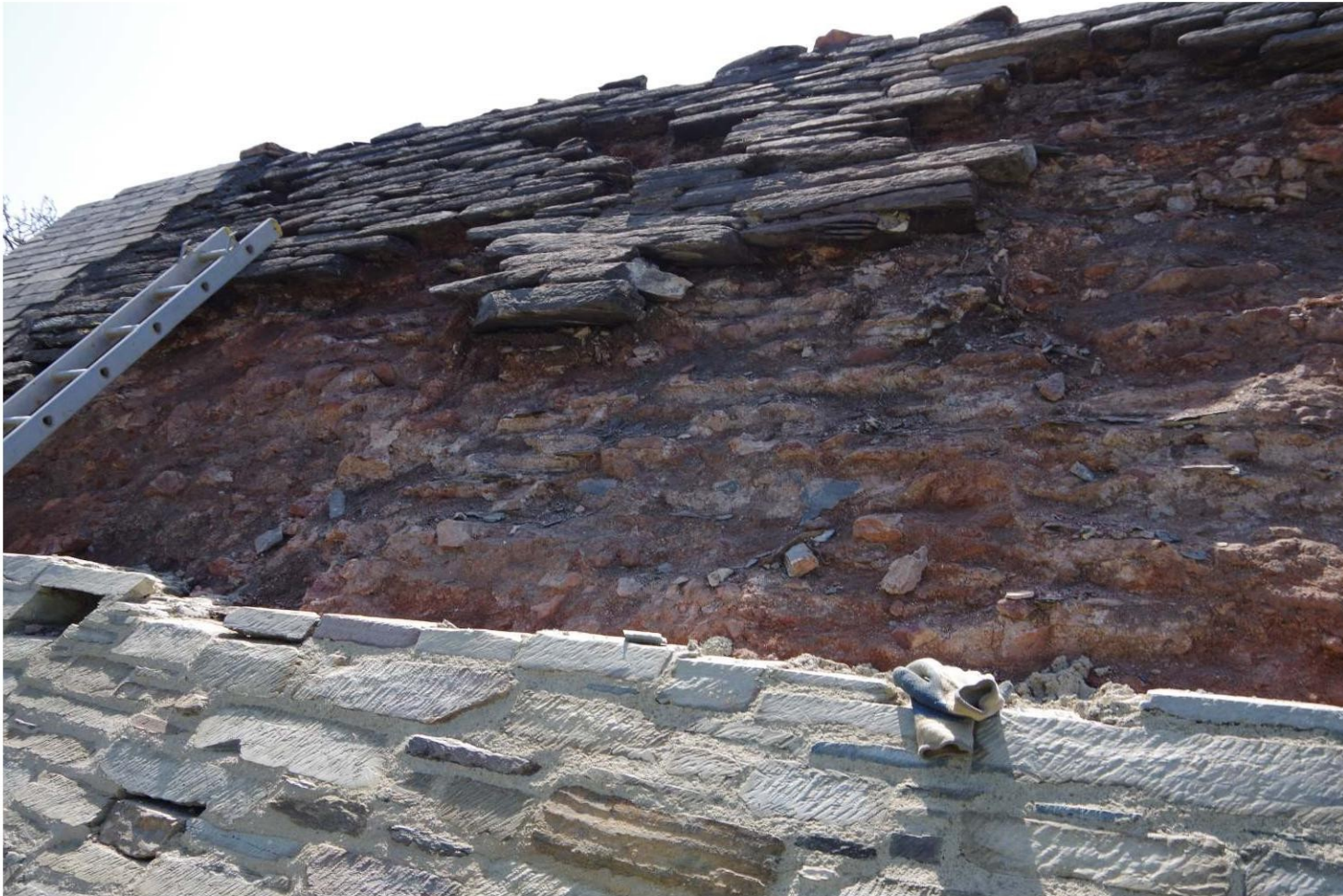
Fig. 13: St Michael's Chapel, northern pitch during conservation works, showing vaulted roof core material.
