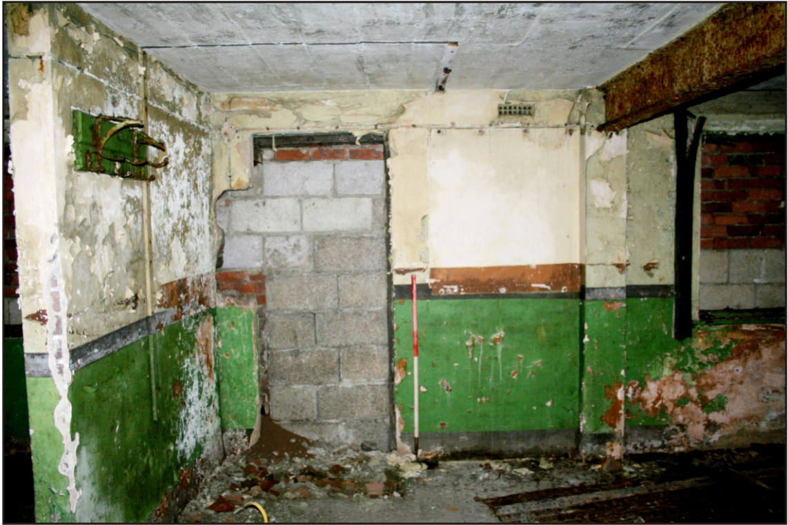
Plate 3 No. 1 gun crew war shelter showing blocked external door, looking north-east. 1m scale.
