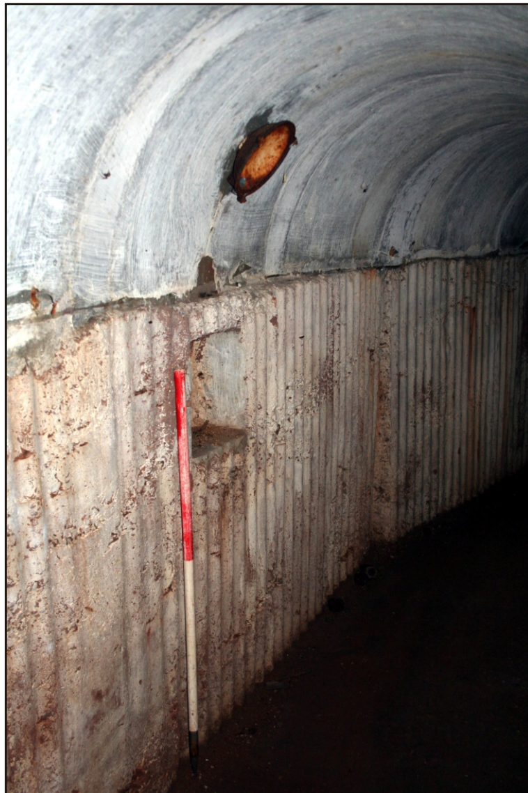
Plate 2 Electric light fitting with void below in the south tunnel, looking south-east. 1m scale.
