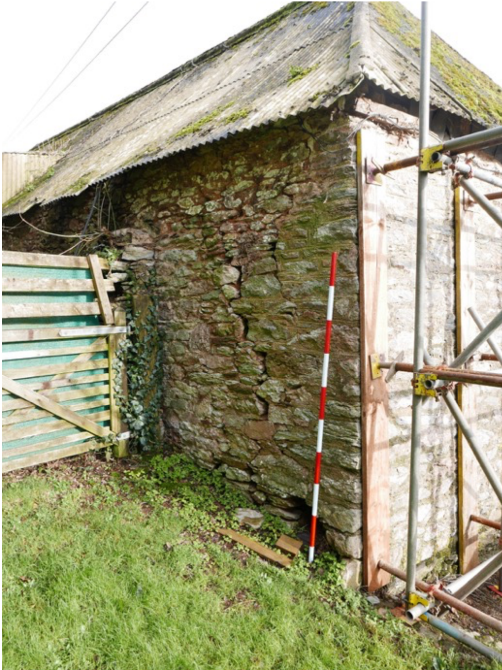
Plate 24. Interior. SW corner showing cracking due to cement pointing.
