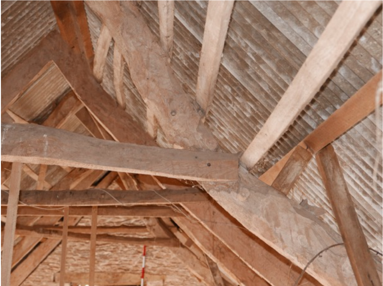
Plate 45. Interior. Roof south end roof timber details showing replacement collar and original peg hole above.
