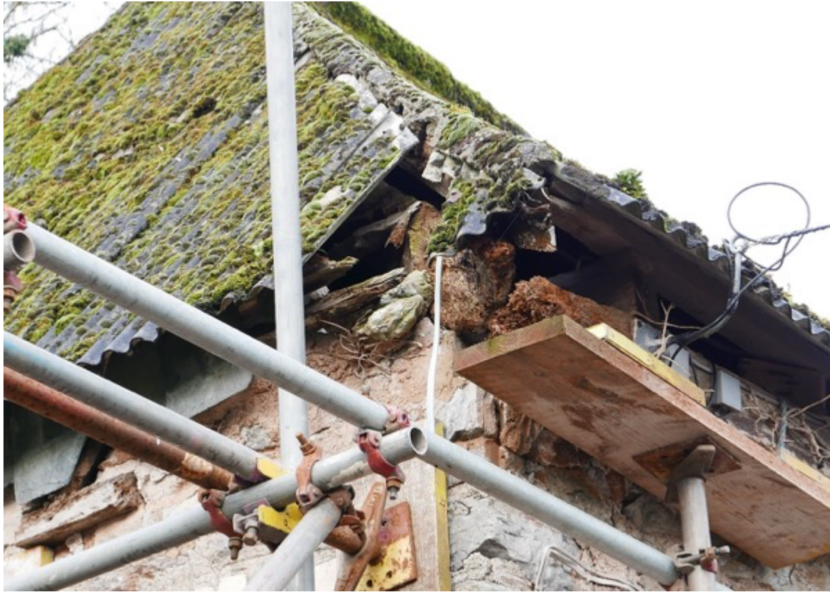
Plate 43. South east corner eaves damage.
