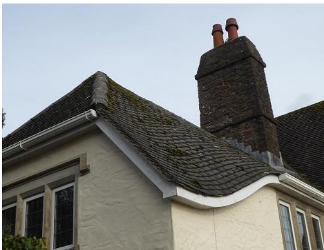
West-facing gable showing the swept eaves to one side of the hipped gable.
