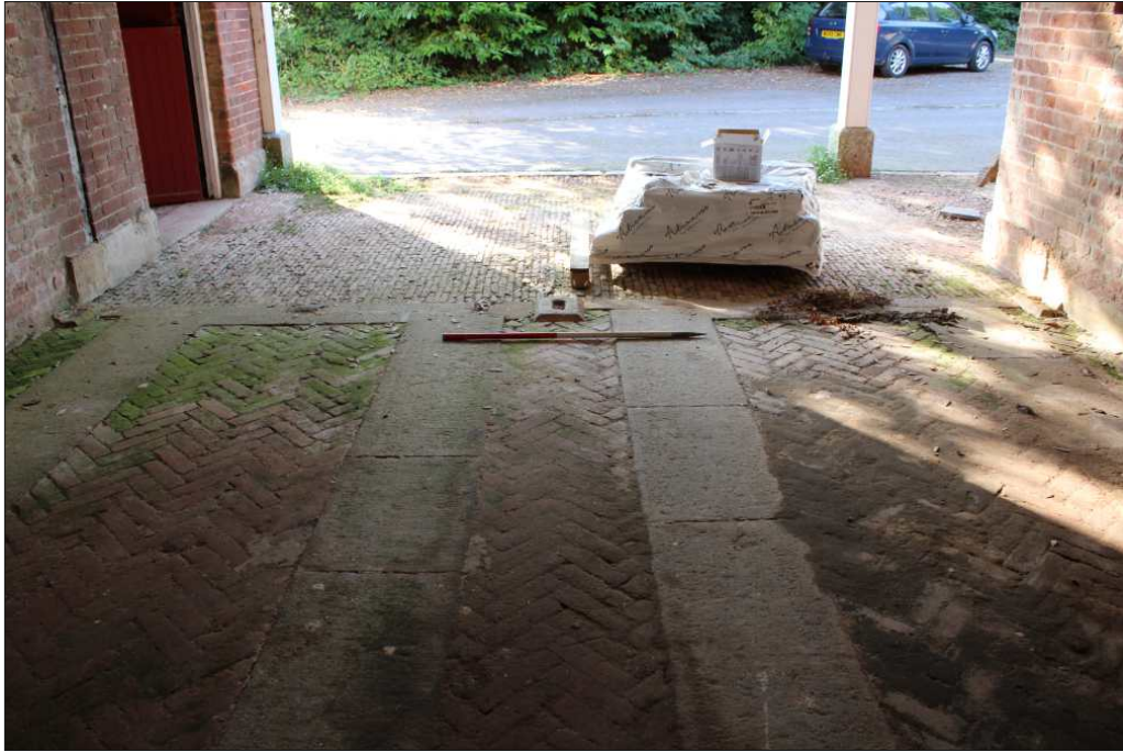
Plate 3: Door fixtures surviving in the floor of the east garage, looking southeast (1m scale)
