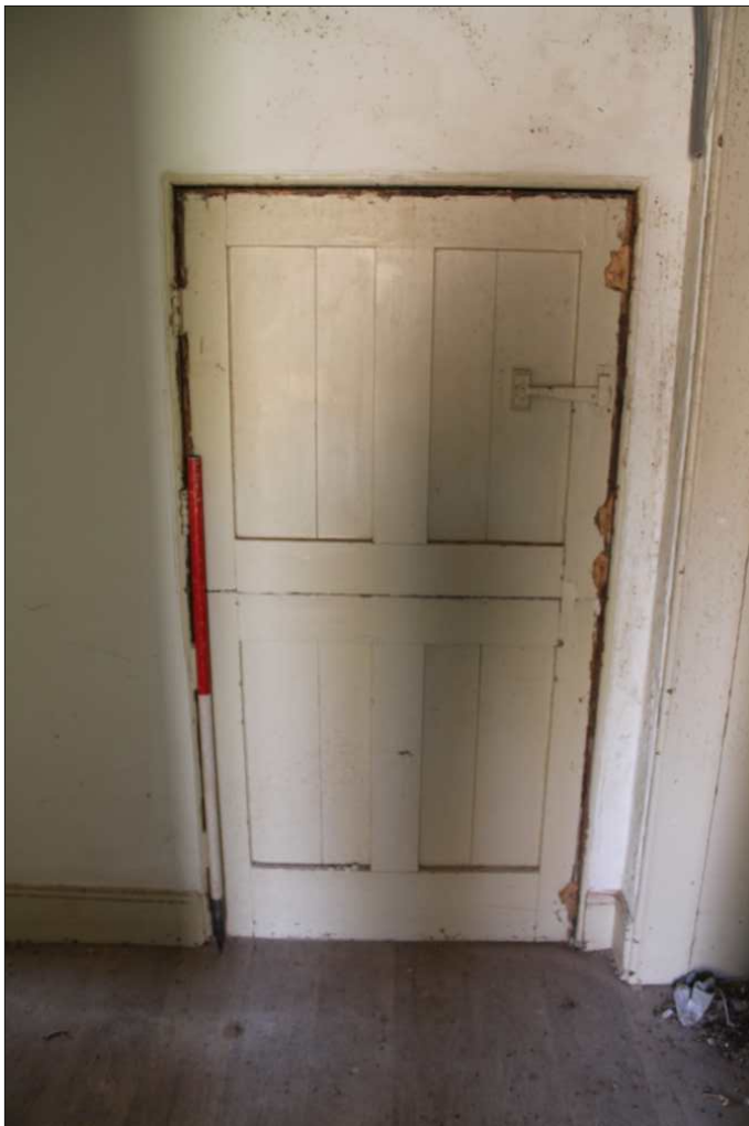
Plate 14: Original door into the lightwell on the first floor, looking southeast (1m scale)
