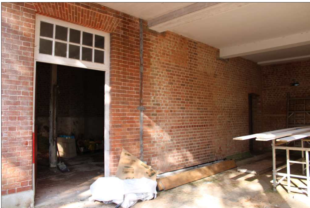
Plate 4: Wall between the west garage and stable, showing the arrangement of doorways (1m scale)
