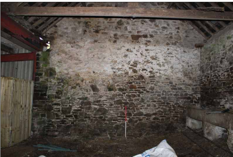
Plate 24: West gable wall of north range showing later phase of stonework to the left, looking west (1m scale)
