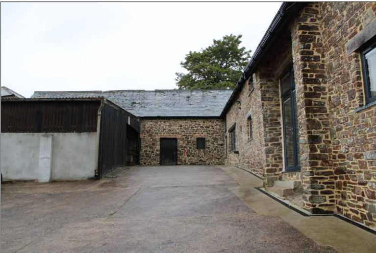
Plate 23: South elevation of the north range, showing the late 20th century lean-to to the left and south range to the right, looking north (1m scale)
