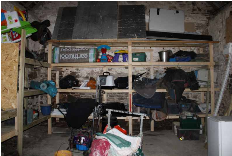
Plate 26: Internal view of east room of north range showing the sloping floor and exposed stone floor to the left, looking east (1m scale)
