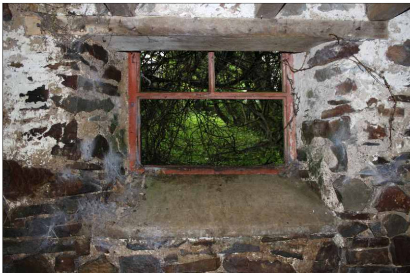
Plate 13: Detail of window on the south-facing internal elevation of the cow house, looking north
